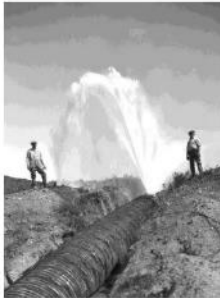
Wooden pipe often failed
