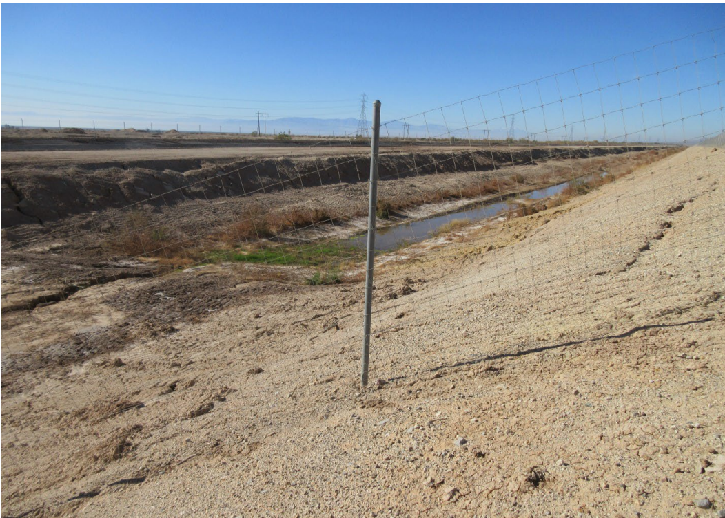
Plate 3. View northwest from Check 11 north from east side of Coachella Canal showing old canal with some remaining water in foreground and newer concrete-lined canal in background.
