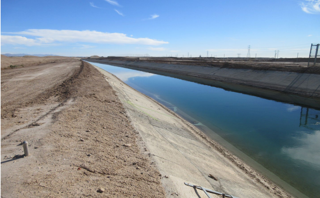
Plate 2. View south from center berm between original and lined canals; concrete-lined canal on right.
