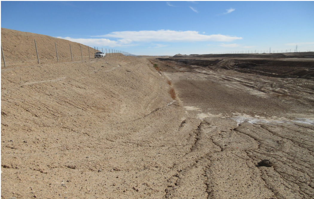
Plate 1. View along east side of original Coachella Canal towards south; embankment created from canal construction spoils shown to east.
