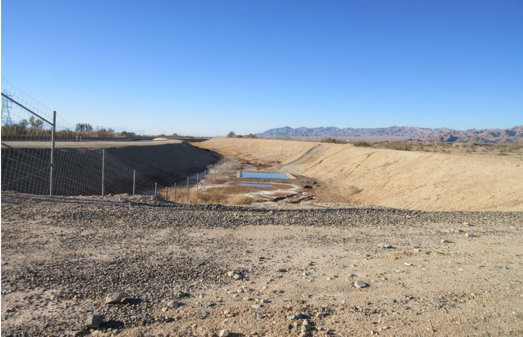
Plate 4. View of old, unlined portion of the Canal towards the north at curve in alignment south of Check 11. Note overall level of disturbance and wildlife drinker midframe. Lined canal is shown to the left.
