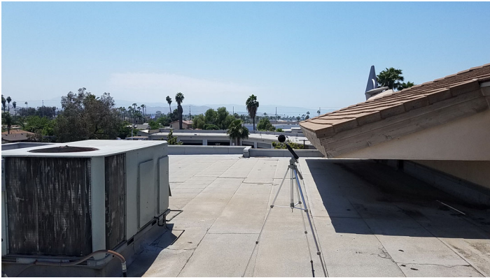
Rooftop HVAC Unit
