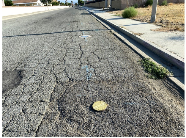
14. View of the typical public right-of-way utilities on the west of the subject property.
