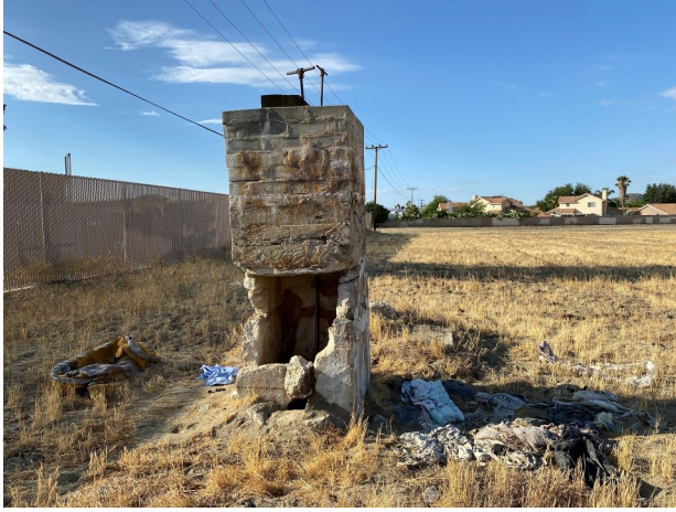
7.View of the irrigation "standpipe style" concrete structure on the east of the subject property.
