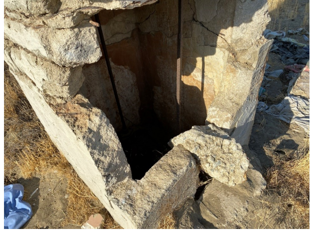
8.View of the irrigation "standpipe style" concrete structure on the east of the subject property.
