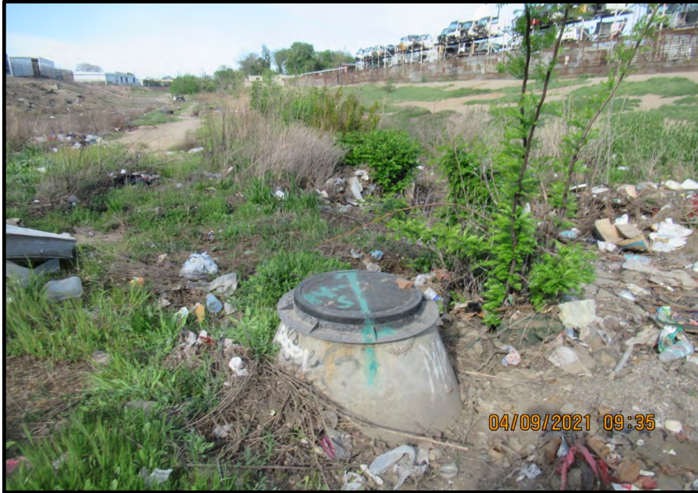
Man hole cover within Mormon Slough in the east part of the site, looking west; 04/09/21.
