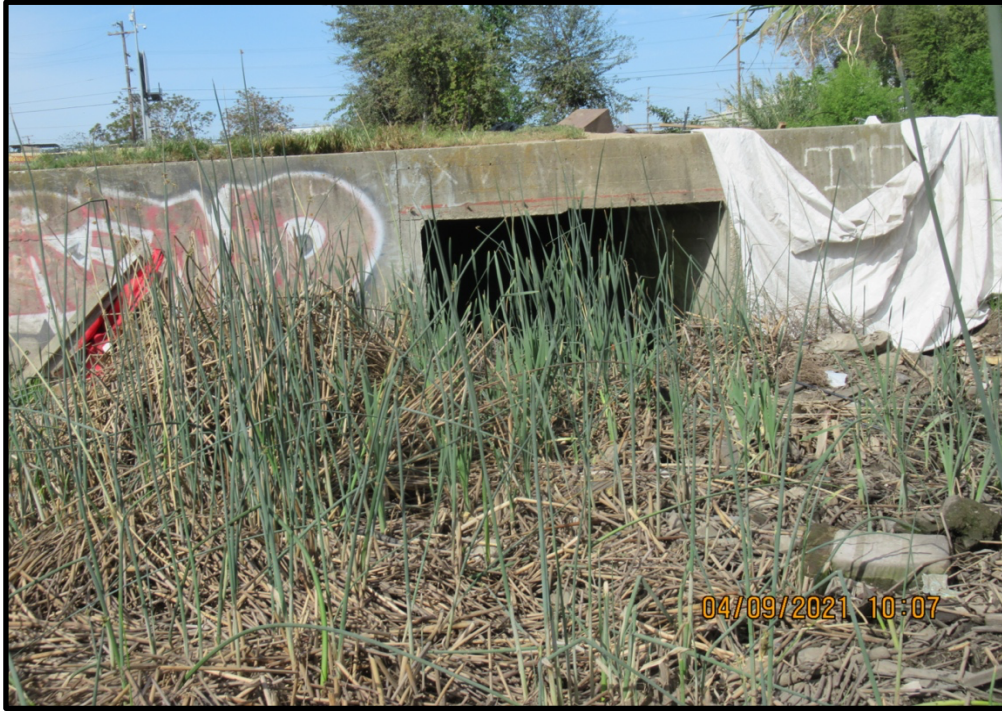
Patch of dense tules at the upstream end of a large box culvert within Mormon Slough; 04/09/21. This is the inlet to a long underground culvert system that conveys flows to the west.
