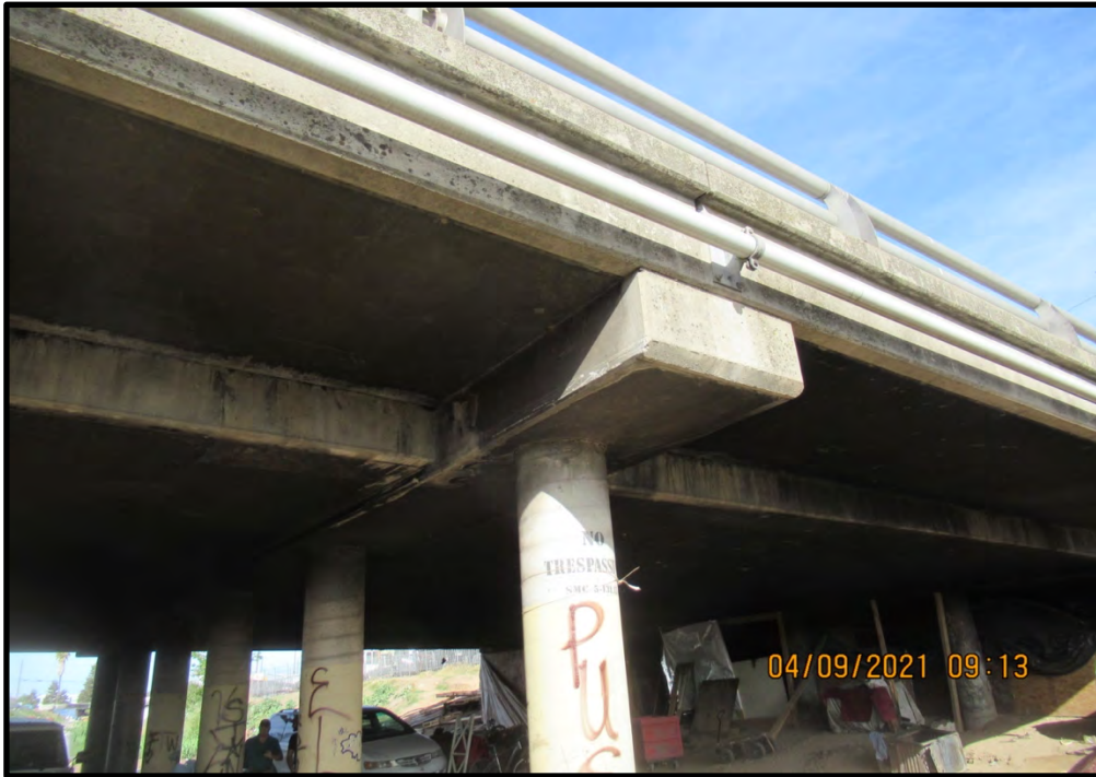
Wilson Way bridge, looking northwest from the east side of the bridge; 04/09/21. There was no evidence of nesting swallows under the bridge.
