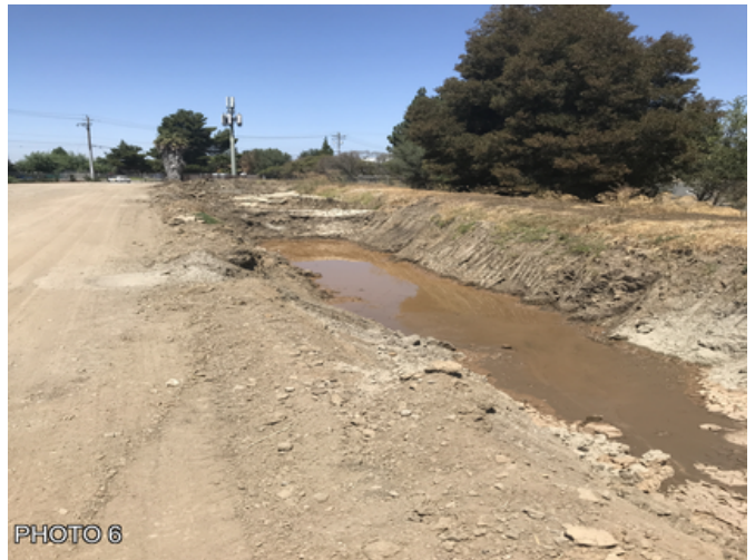
EXCAVATED TRENCH WITH PONDING WATER ALONG NORTHEAST PERIMETER OF PROPERTY
