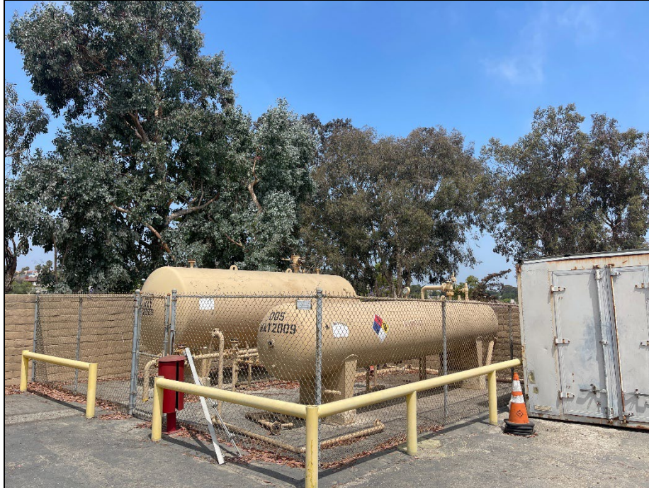
Photo 13: CUP Site No. 6. View of existing structures within the site; eucalyptus trees along boundary wall, facing northwest.
