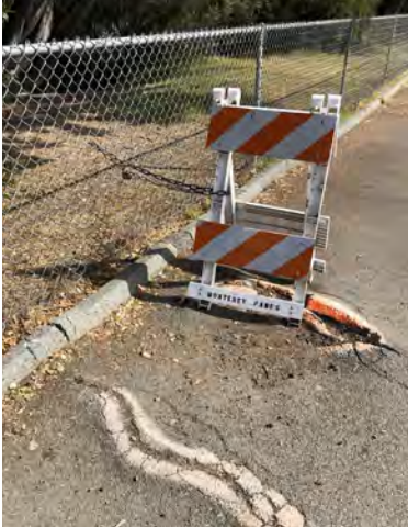
Asphalt Trail Root Impacts
