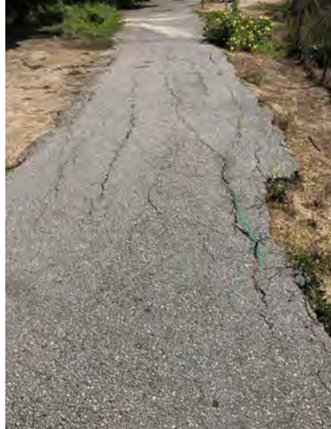
Asphalt Trail in Poor Condition
