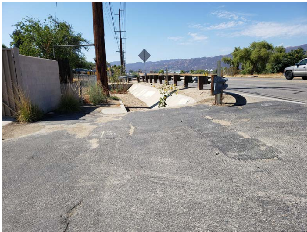
Photo of an open storm drain along Mission Trail south of Olive Street. Photo taken 8/5/2022.
