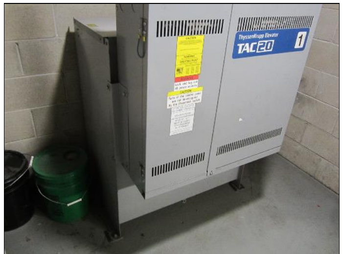
18. Interior of the subject building - elevator equipment.
