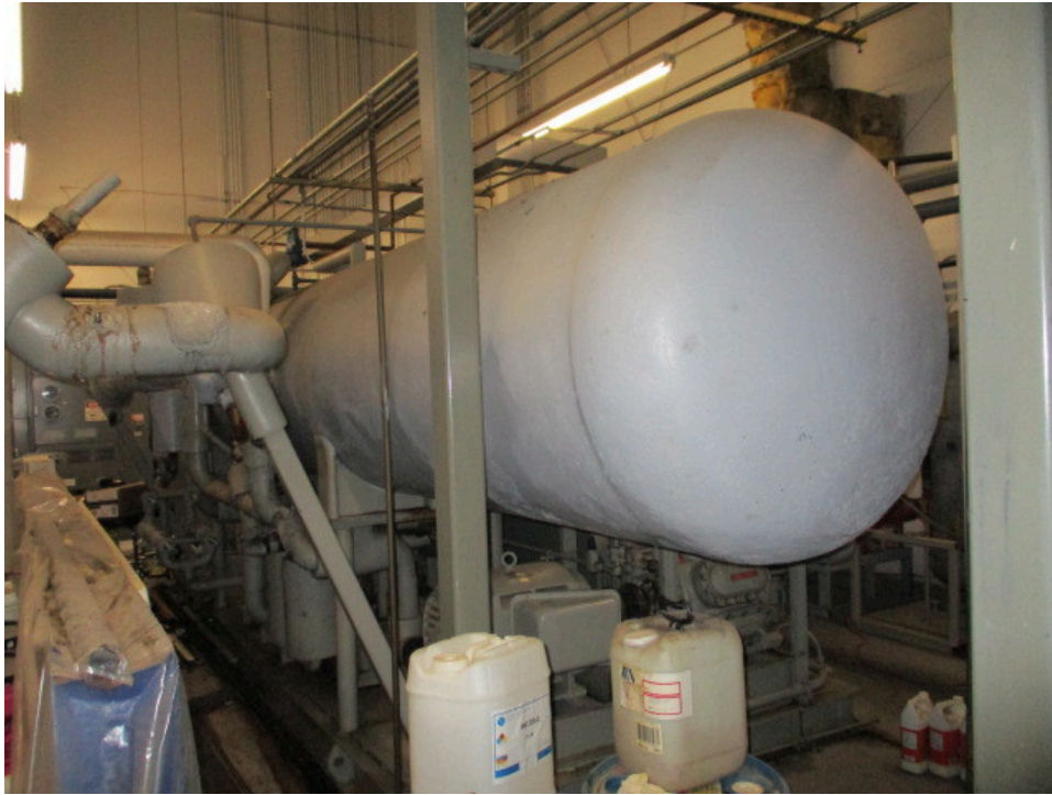
31. Refrigerant tank in the compressor room
