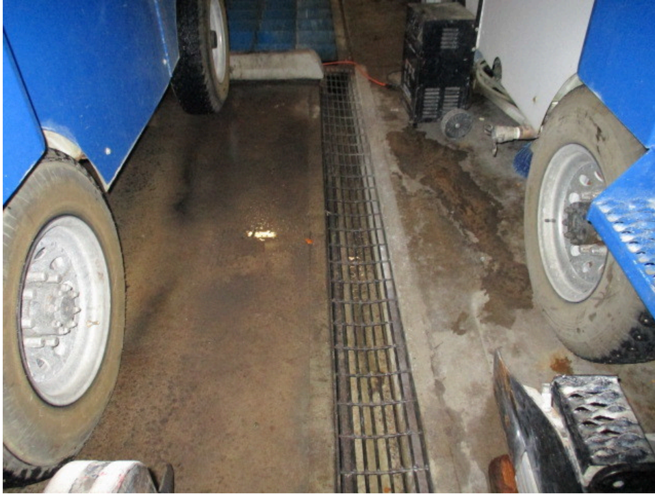
25. Trench drain in the Zamboni storage room
