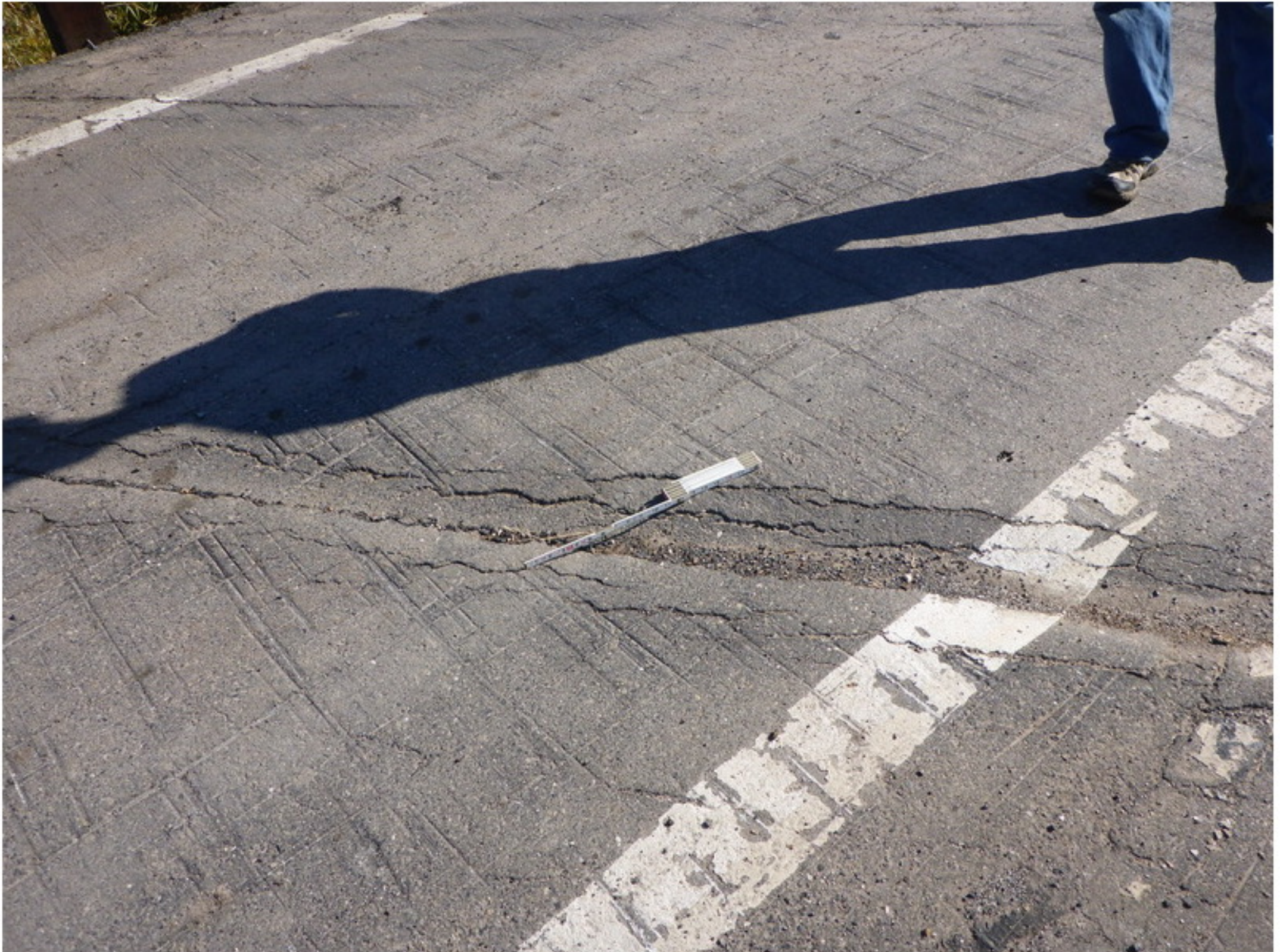
Photo No. 2 Transverse dip in the deck AC at midspan of Span 2
