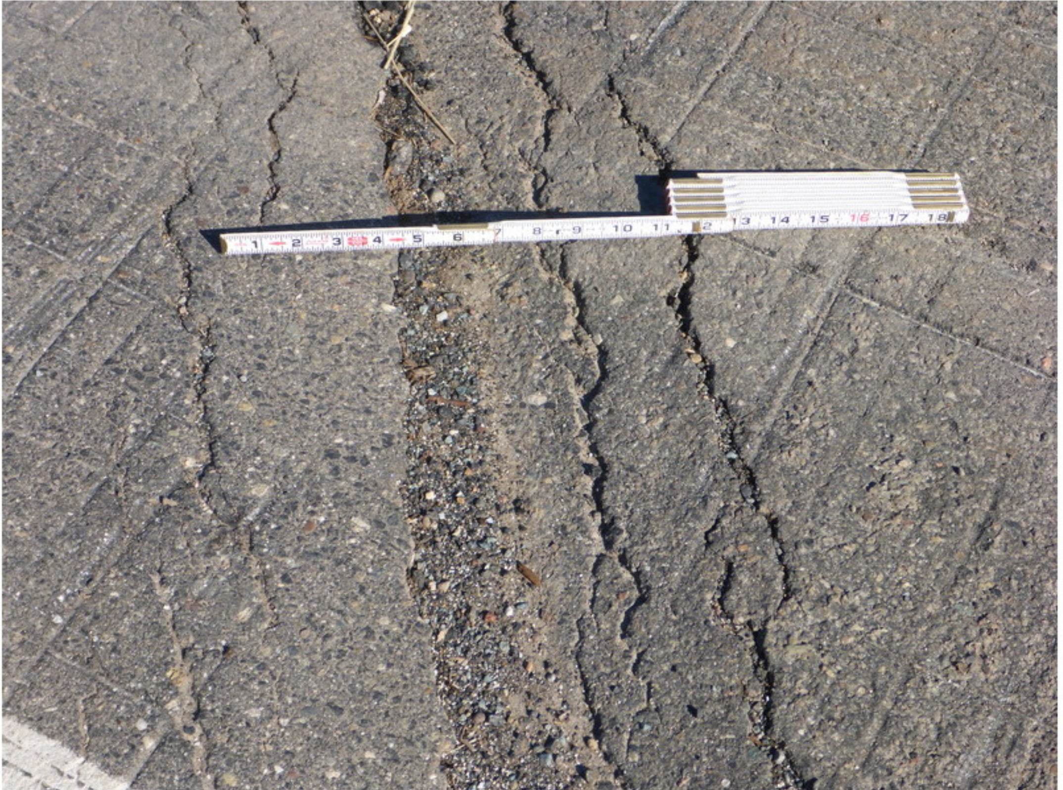
Photo No. 3 Transverse dip in the deck AC at midspan of Span 2
