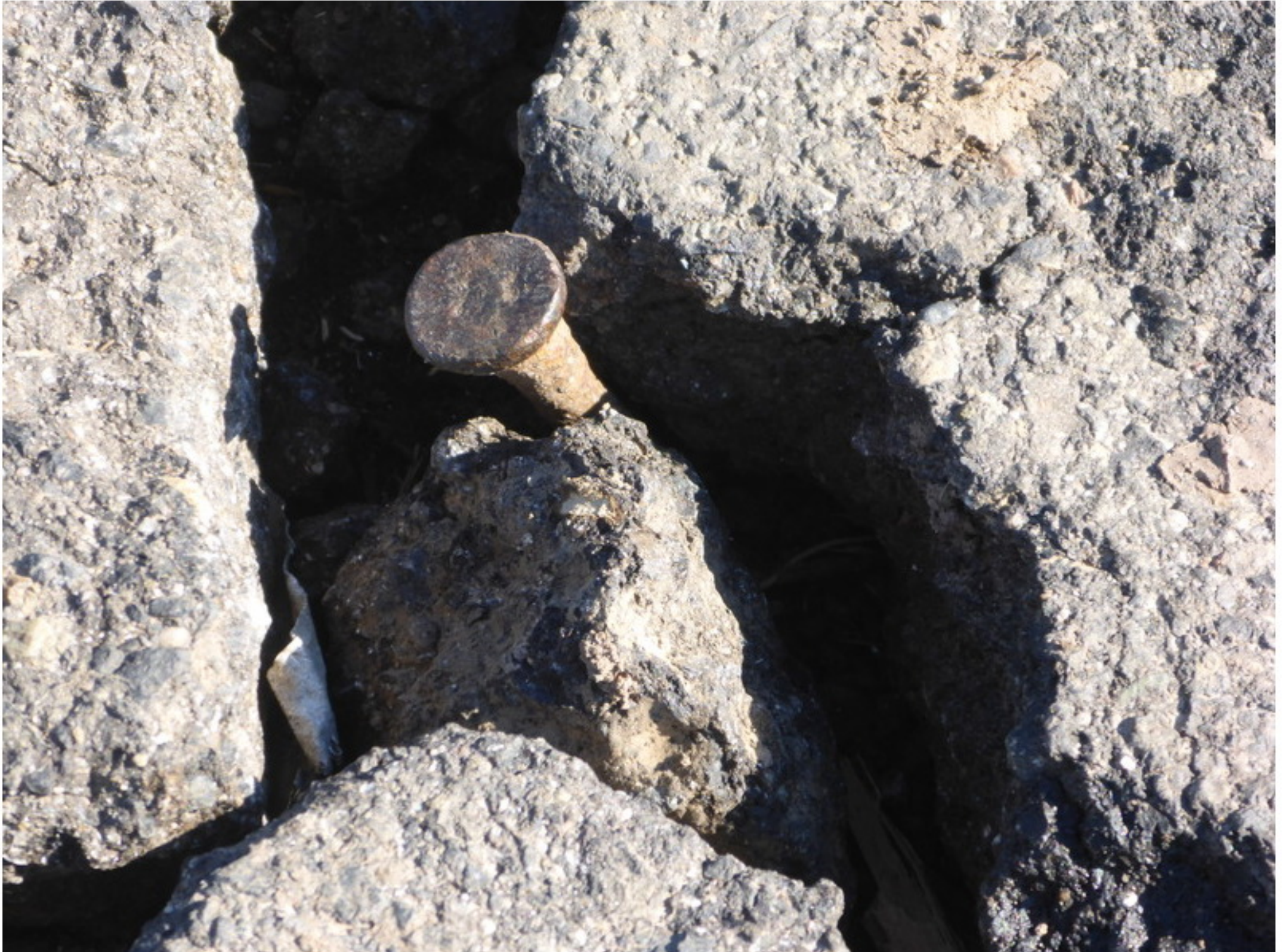
Photo No. 6 Spike sticking out of the deck AC near Abutment 4
