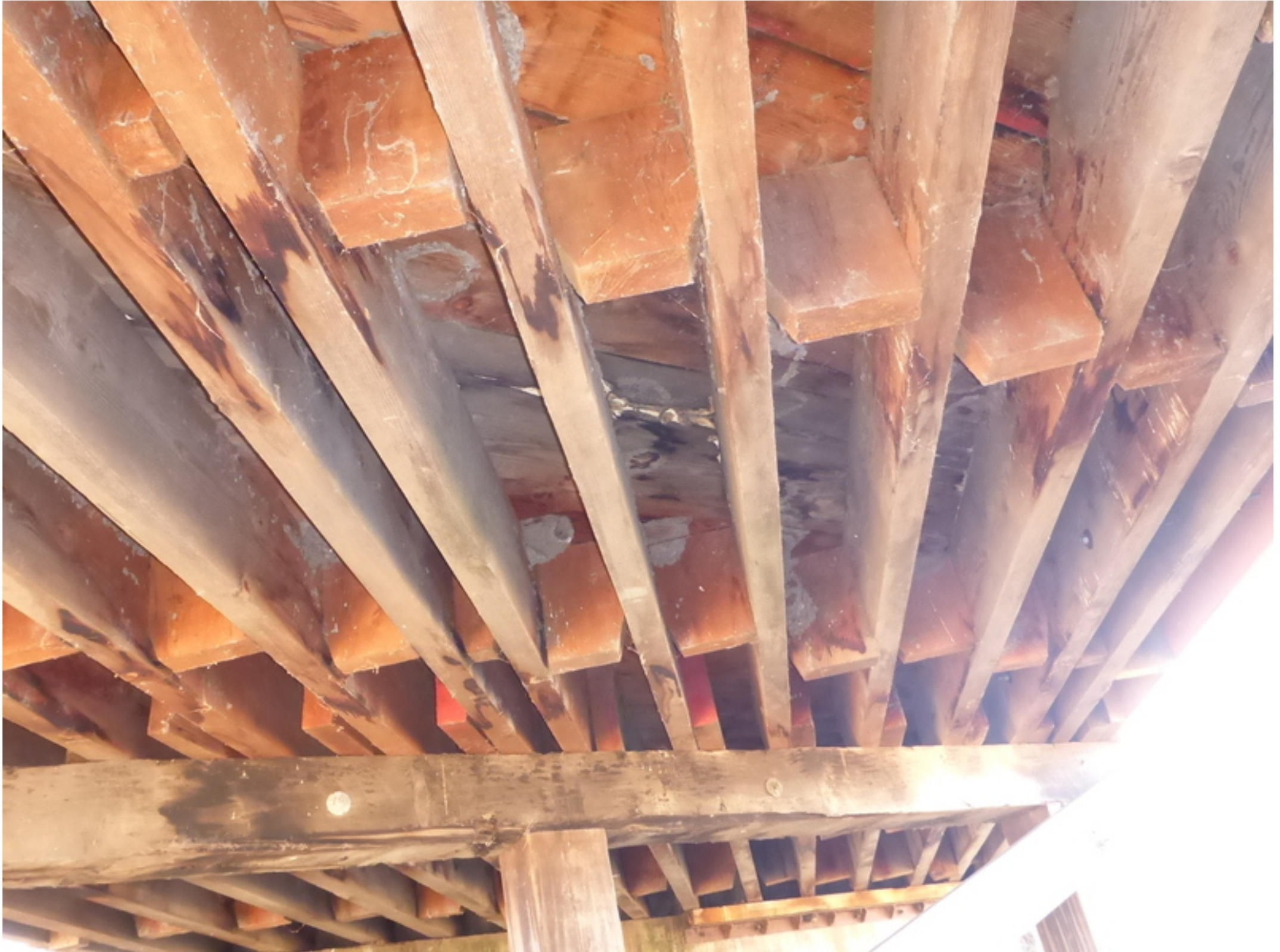
Photo No. 9 White fungus on the soffit of Span 2
