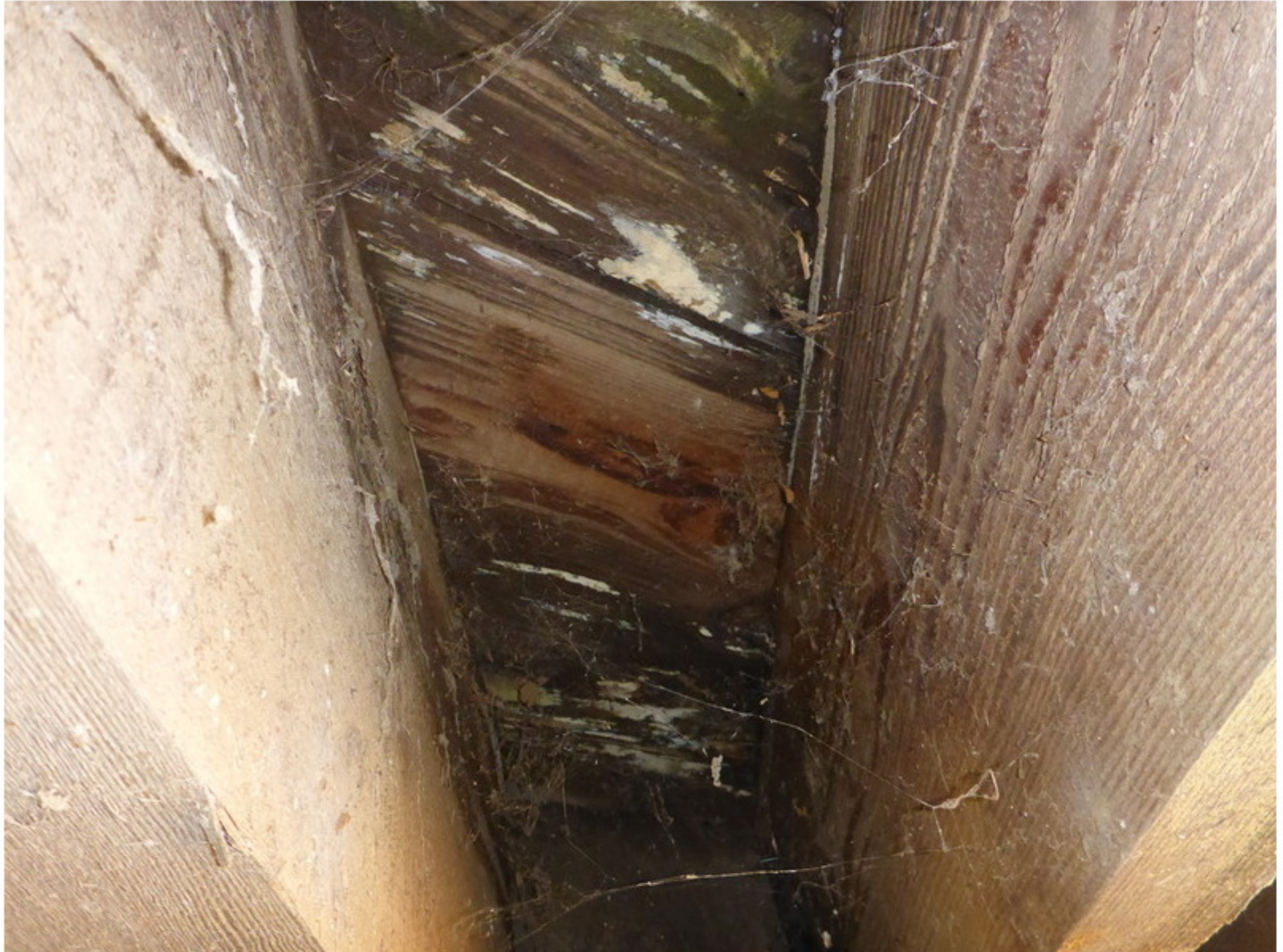
Photo No. 7 White fungus present on the soffit near Abutment 4
