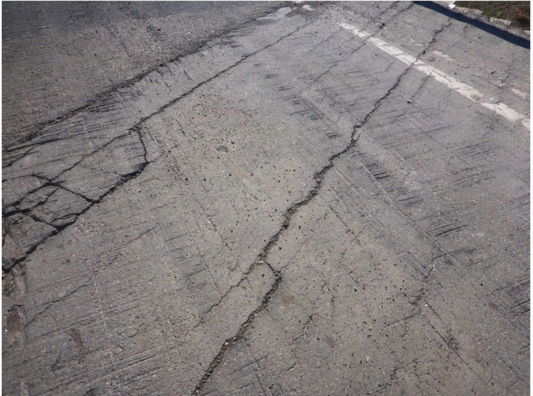
Photo No. 1 Transverse cracks in the deck AC
