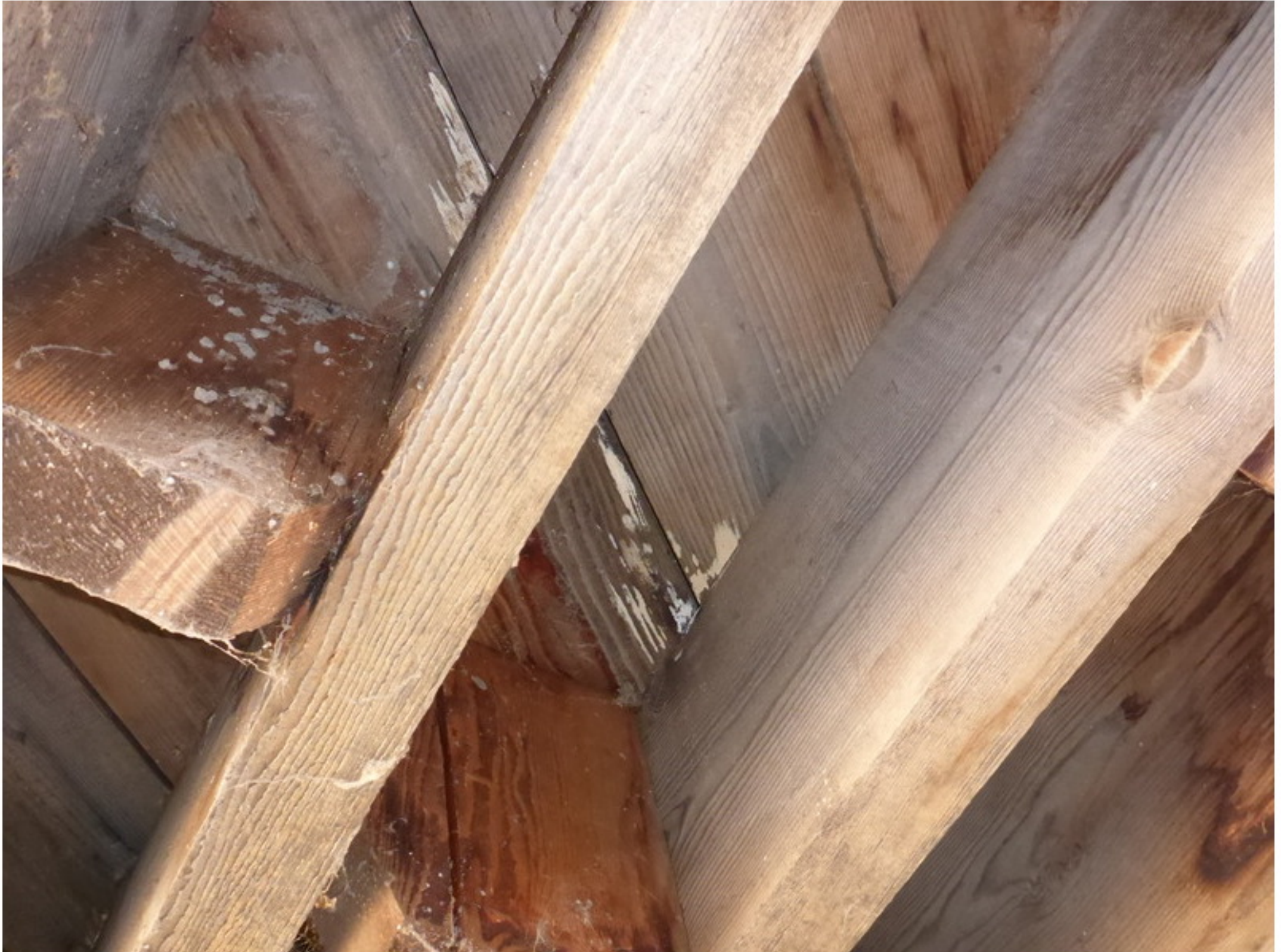
Photo No. 7 White fungus on the left side of Span 3
