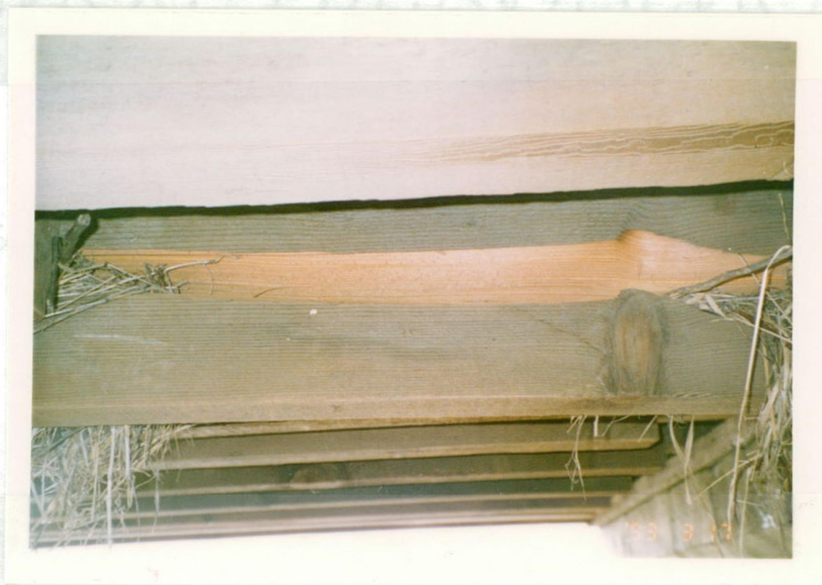
SPLIT ON STRINGER #8 OF SPAN 3 3-16-93.17 TH-4
