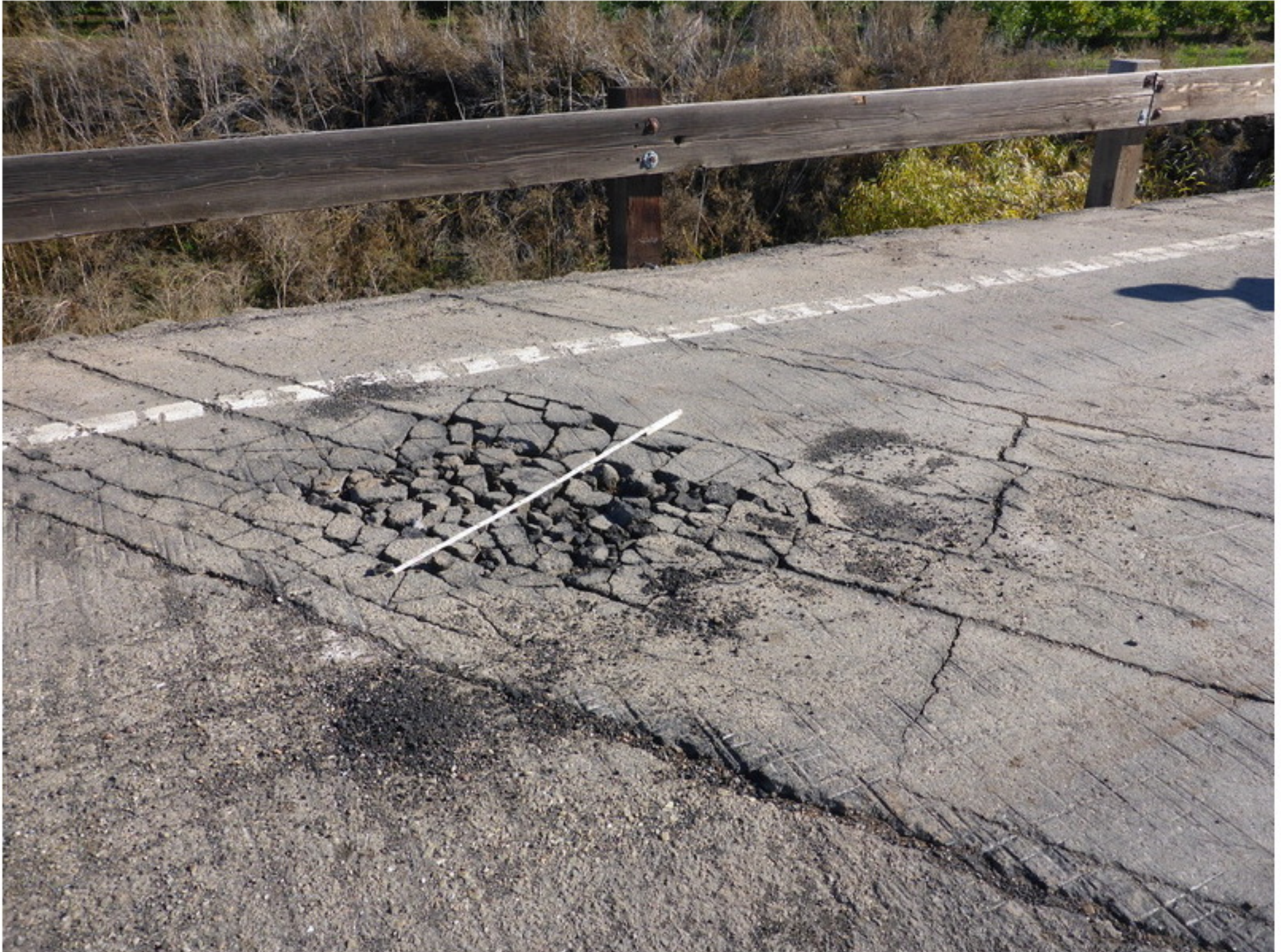
Photo No. 4 AC breaking up in the deck near Abutment 4
