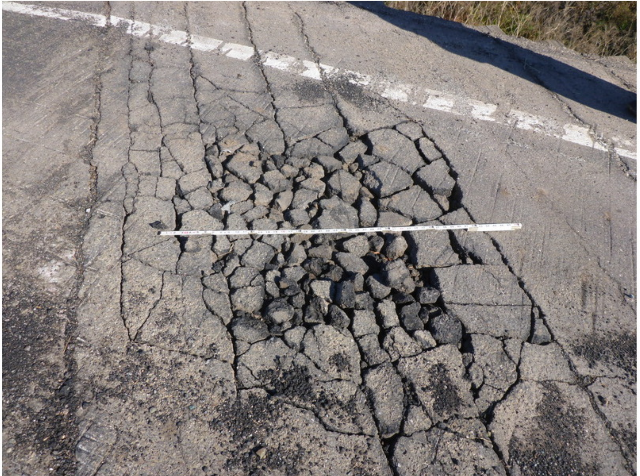
Photo No. 5 AC breaking up in the deck near Abutment 4
