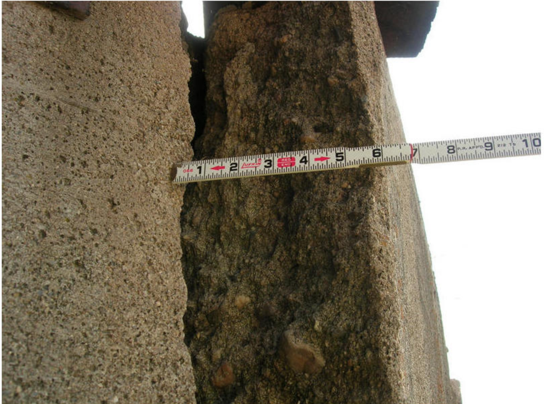
Photo No. 1 Movement of the left wing wall at Abutment 1.
