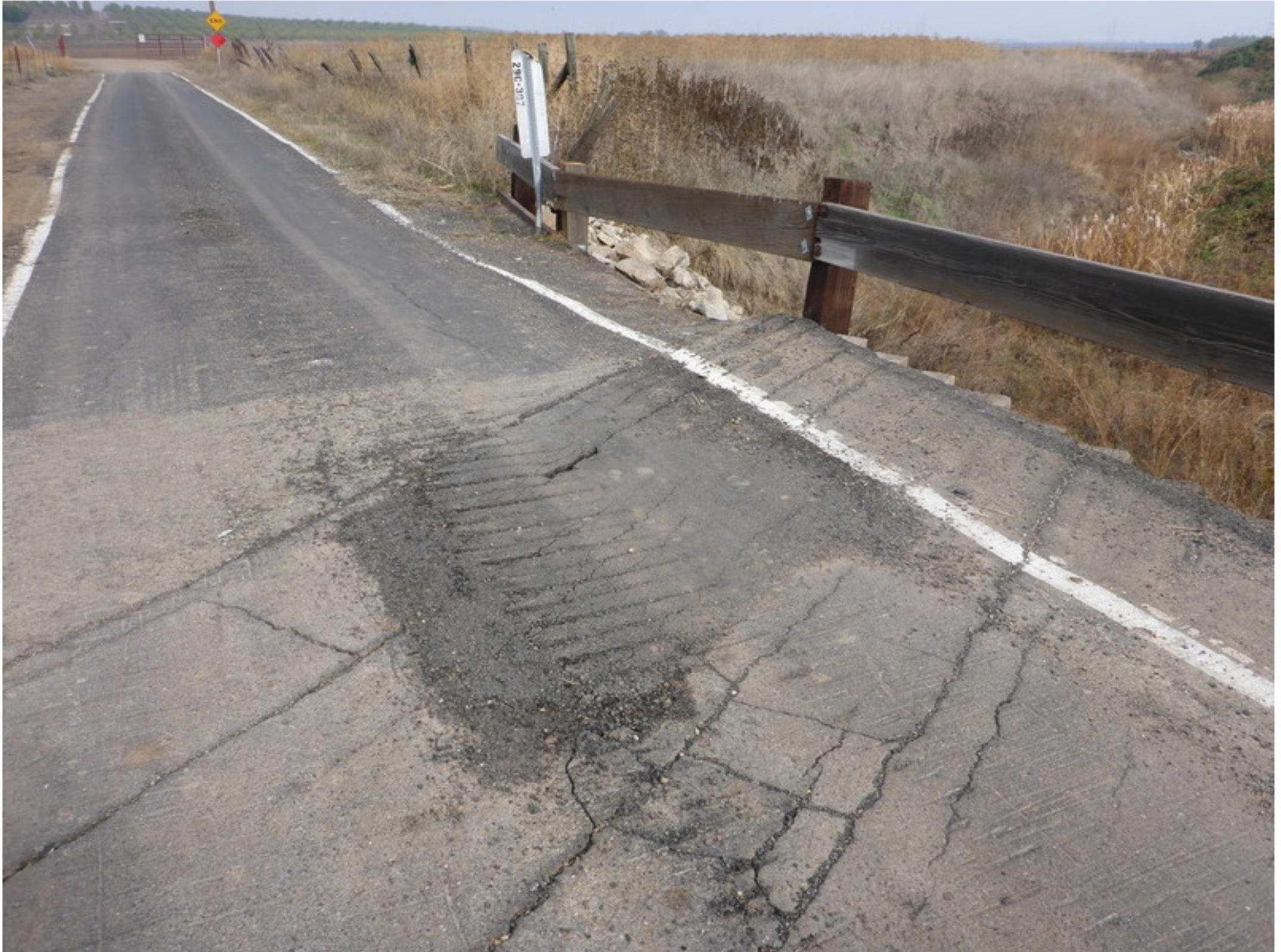
Photo No. 2 AC patch at Abutment 4 right.
