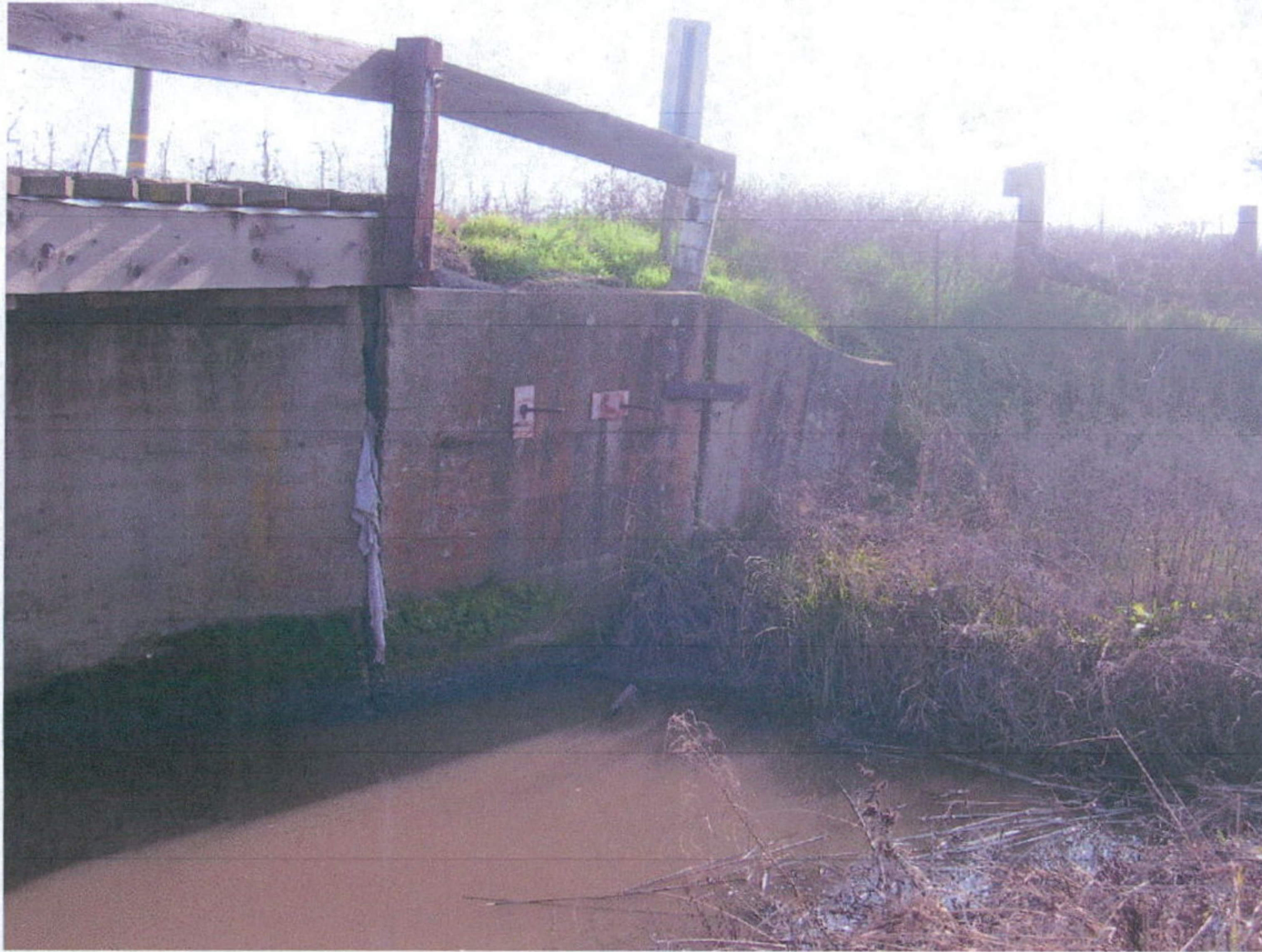
DETERIORATION: Left wingwall at Abutment 1
