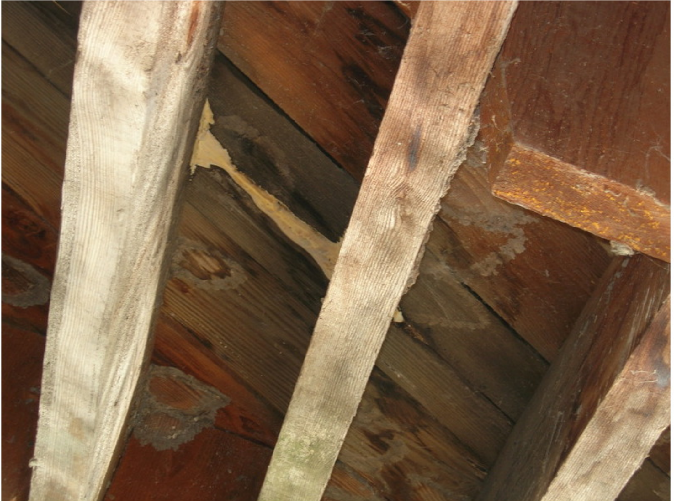
Photo No. 2 White fungus on the soffit of the deck planks.
