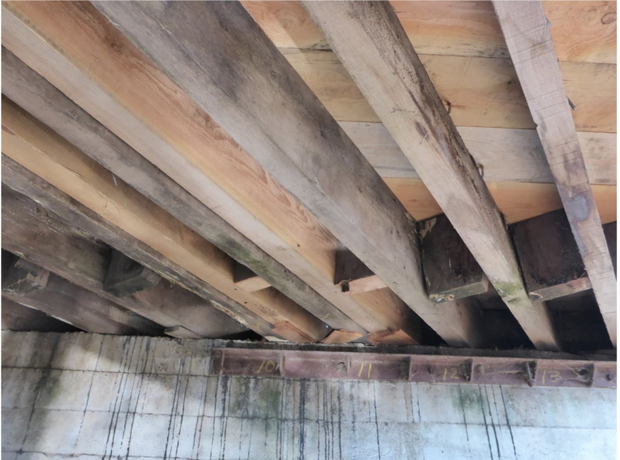
Photo No. 8 Supplemental girders (7 and 8) and new decking as seen from Span 3 right.
