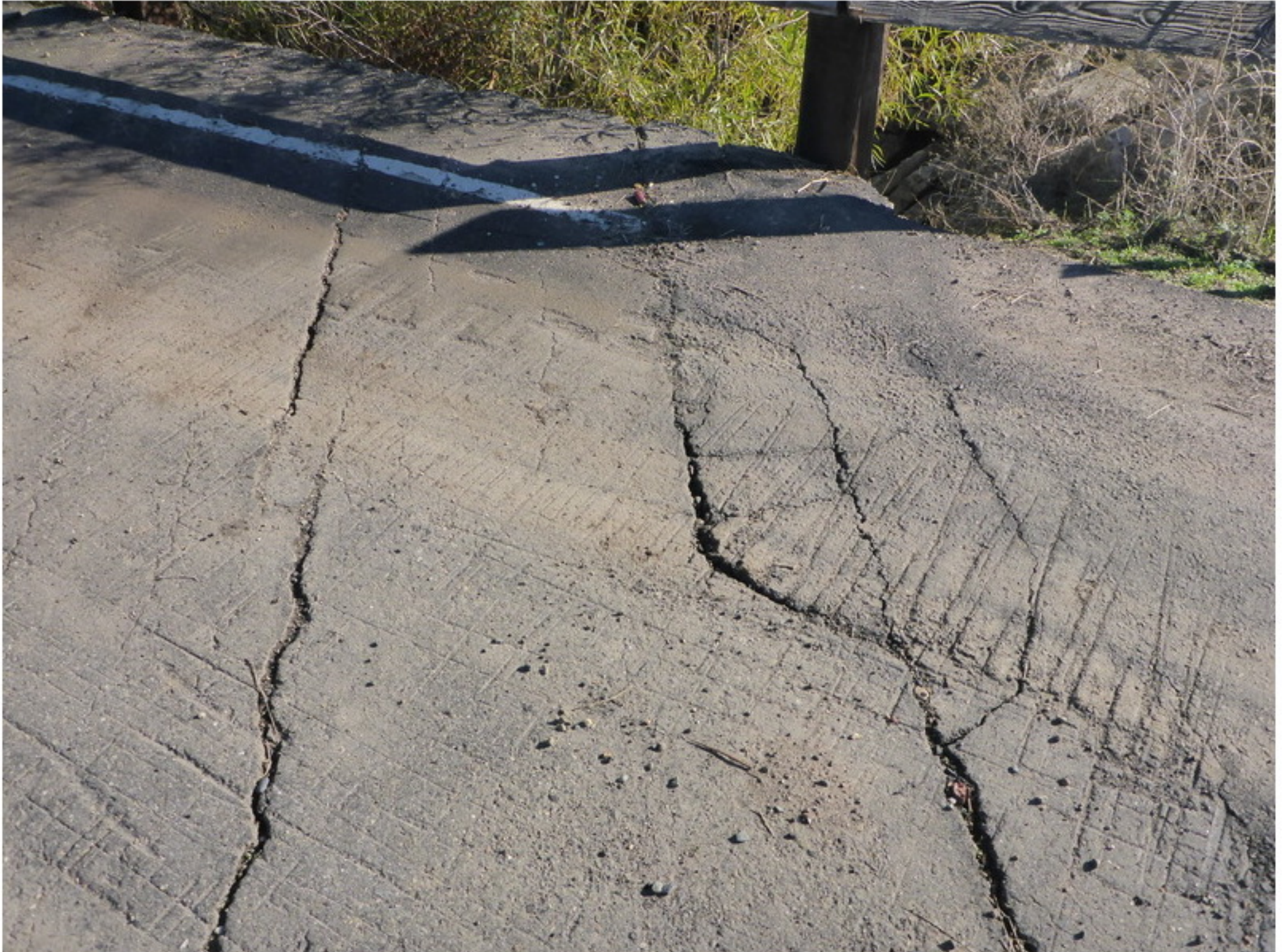
Photo No. 1 Cracking AC at the right side of Abutment 1.
