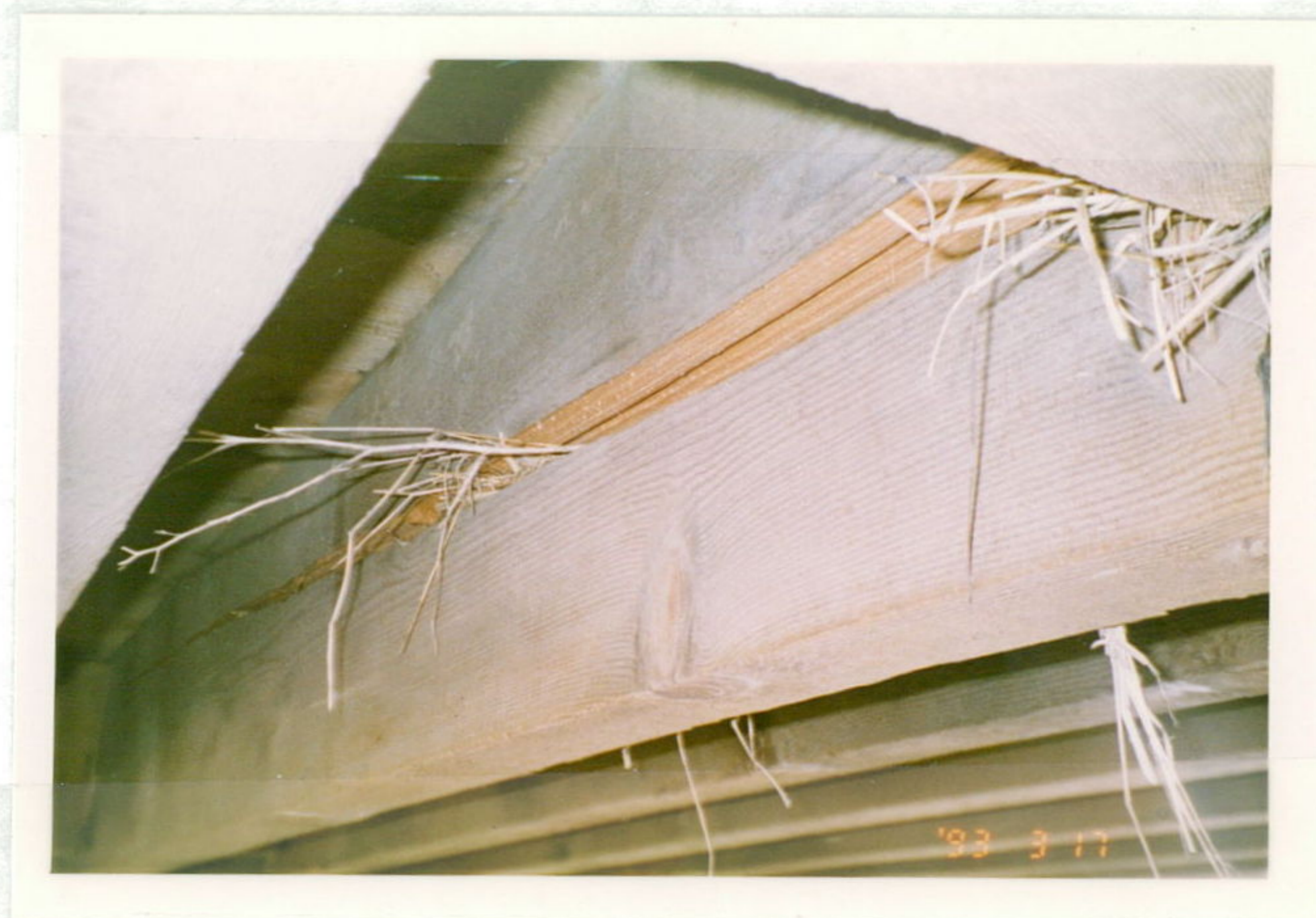
SPLIT ON STRINGER #8 OF SPAN 3 3-16-93.18 TH-4
