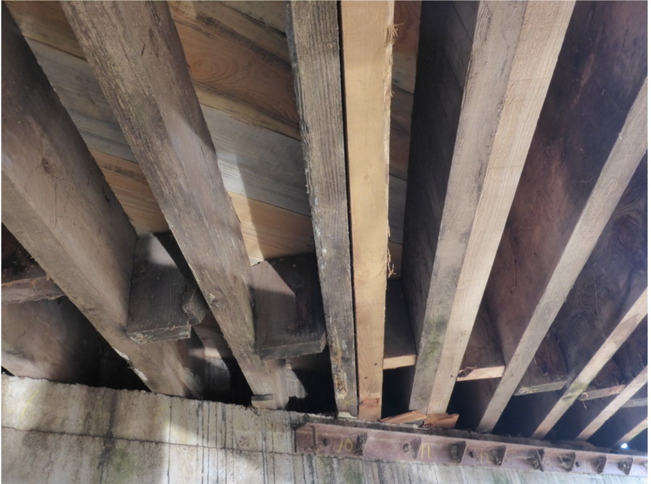
Photo No. 9 Supplemental girders (7 and 8) and new decking as seen from Bent 3.
