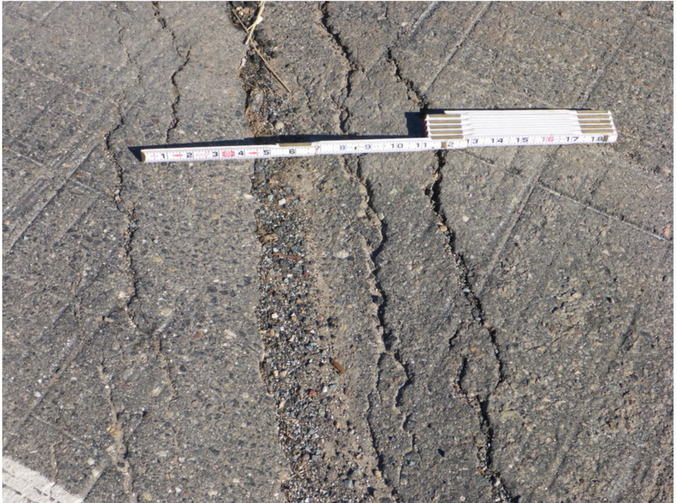
Photo No. 3 Transverse dip in the deck AC at midspan of Span 2
