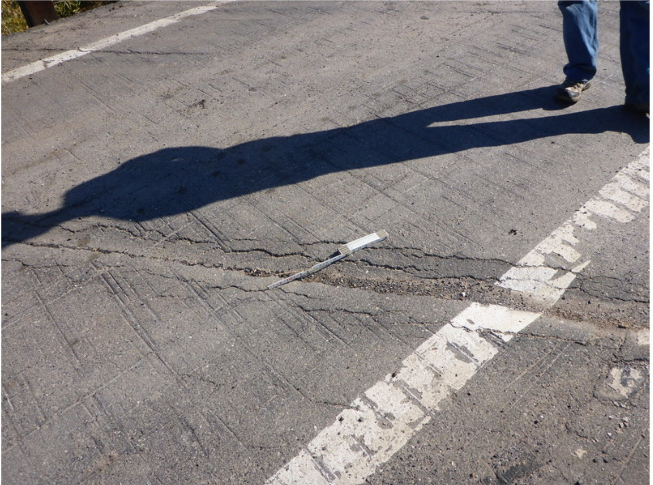
Photo No. 2 Transverse dip in the deck AC at midspan of Span 2
