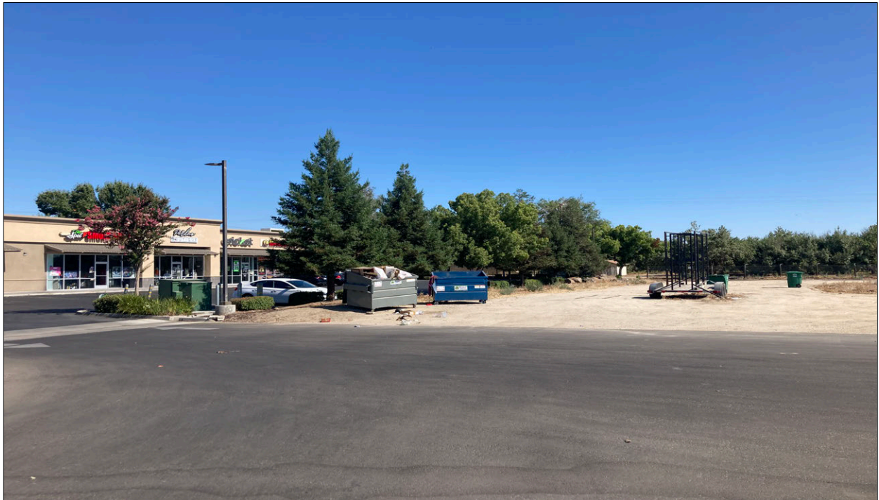
Figure 7. Photograph of a sewer line repair site, looking northwest from a commercial parking lot, showing commercial development with an orchard in the background.
