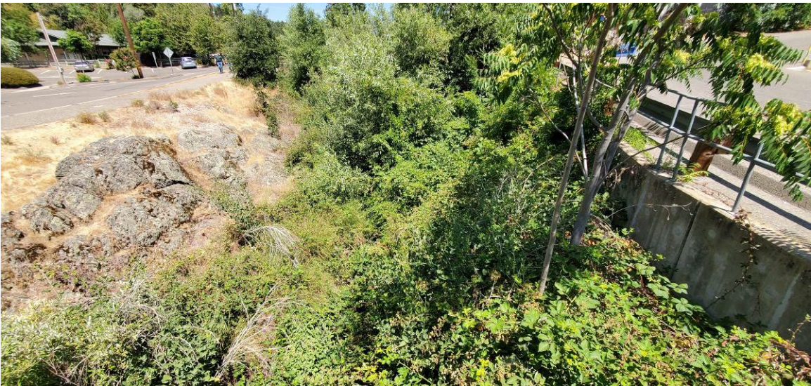
Photo 8: Mariposa Creek channel south of 8 th Street choked with Himalayan blackberry and other vegetation.
