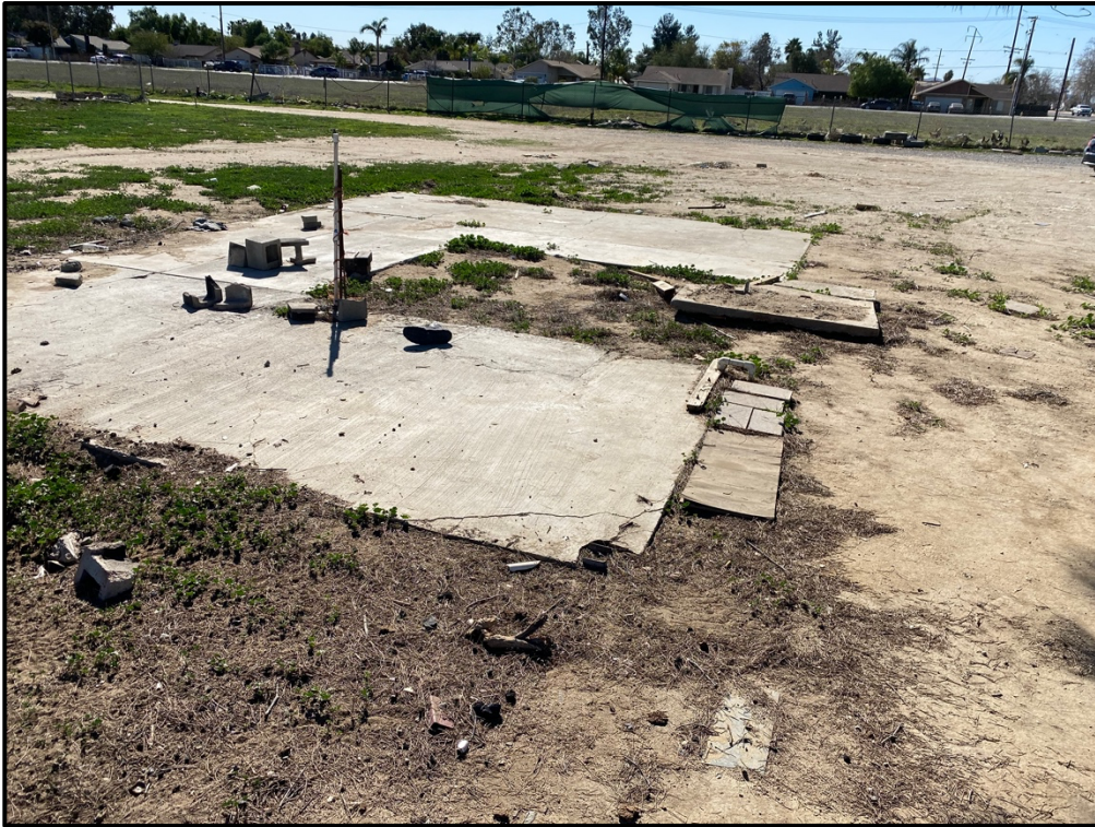
Plate 3: View of the remnant concrete pad and building materials from the recently demolished 1983 prefabricated residence, facing southeast.
