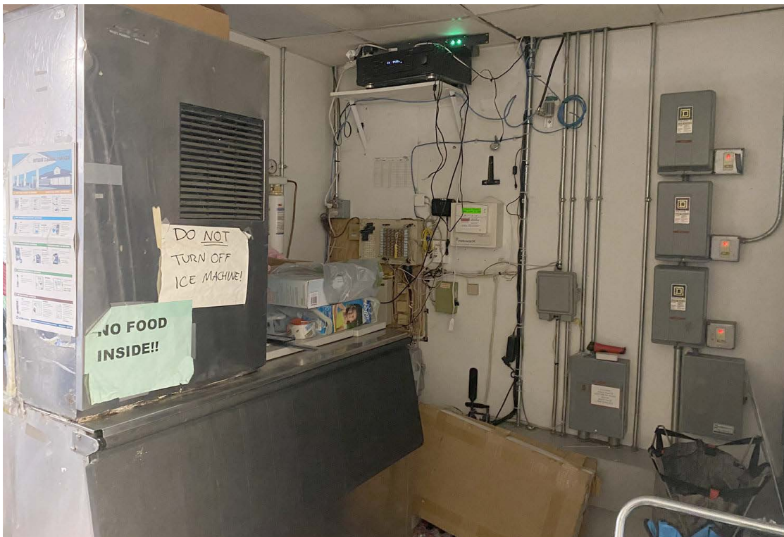
Photo No. 6 Ice machine and electrical panels in convenience store
