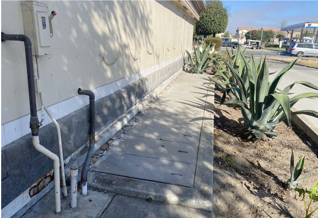
Photo No. 11 View to the north along eastern side of the Site of recycled water access for car wash
