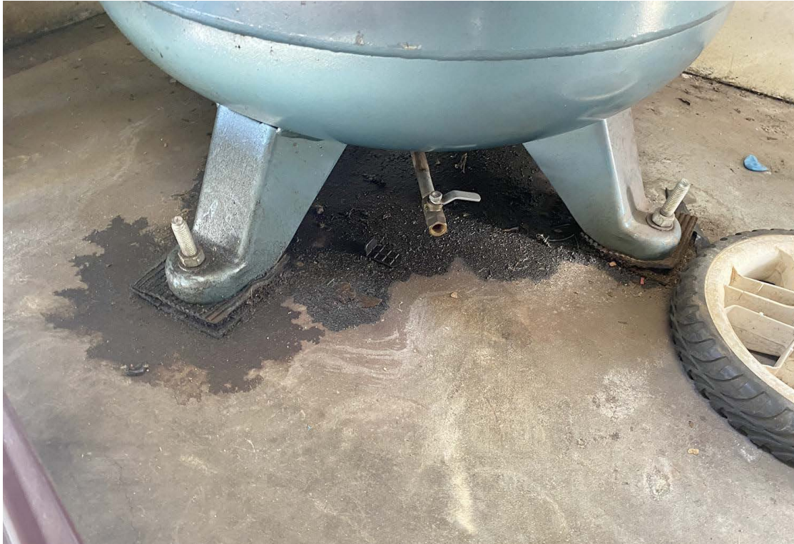
Photo No. 9 De minimis staining beneath air compressor in equipment room
