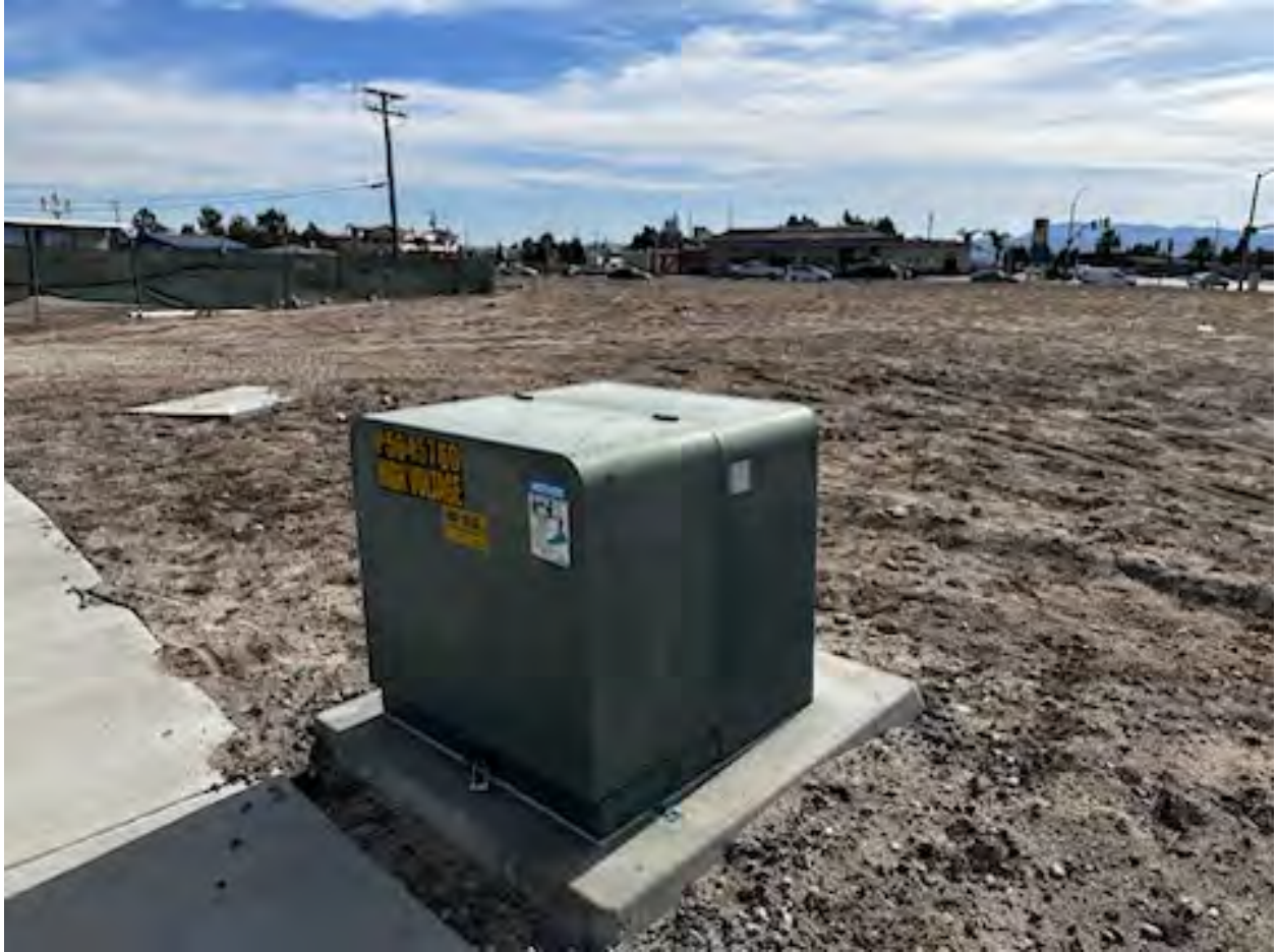
Pad mounted transformer located at the northern boundary of the site.
