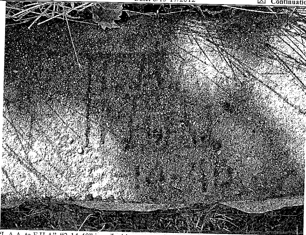
"L.A.A. to F.H.A", "2-14-40" inscribed in stone retaining wall (Feature 8). View to south, 8/17/2012.
