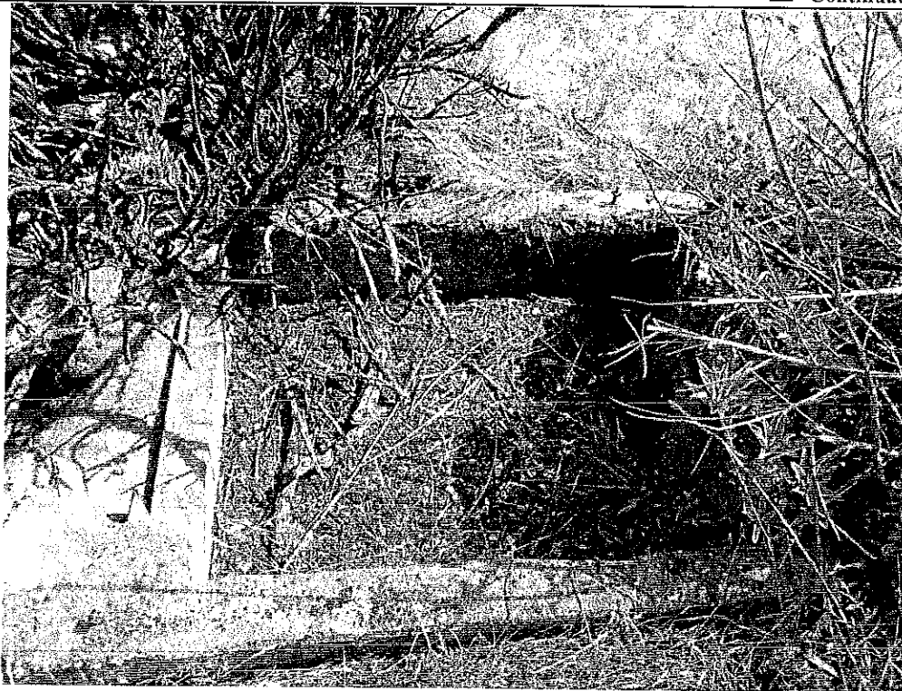
Concrete weir box attached to concrete reservoir (Feature 22d). View to south, 8/15/2012.
