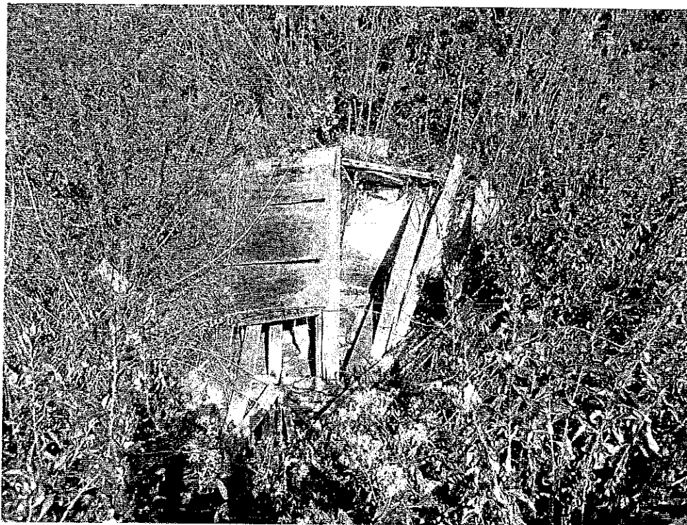
Concrete weir box with collapsed roof (Feature 22e), east of concrete reservoir (Feature 22d). View to northeast, 8/15/2012.
