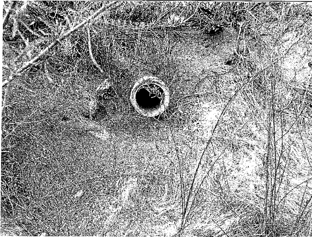
Concrete irrigation pipe in north half of site (Feature 25). View to south, 8/16/2012.
