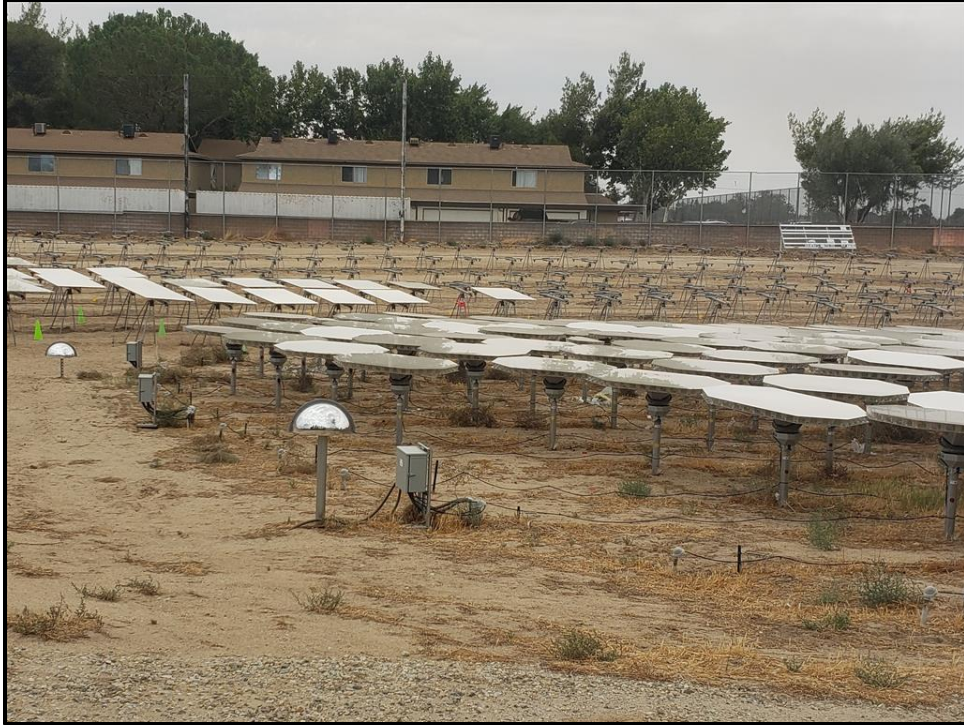
Photo 4. Solar reflector panels in the southwest of the subject property.
