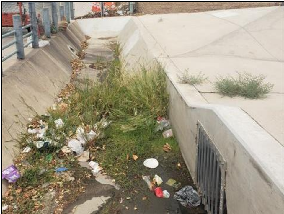
Photo 17. View of debris at front section of spillway.
