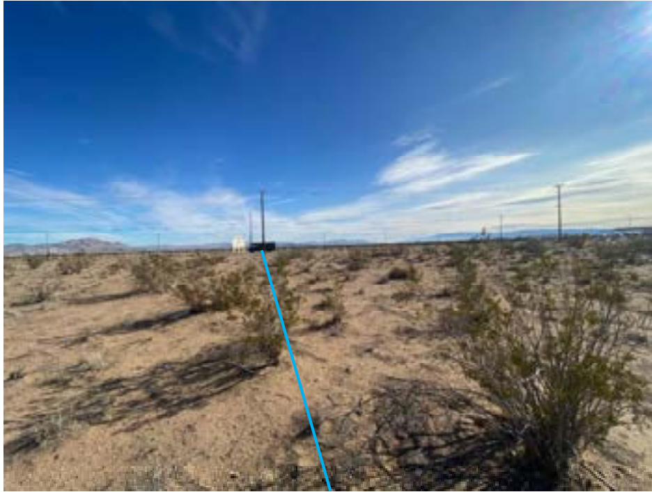
Location of 240 ft. of power and Telco trenching. View to east. Blue line represents trenching location.
