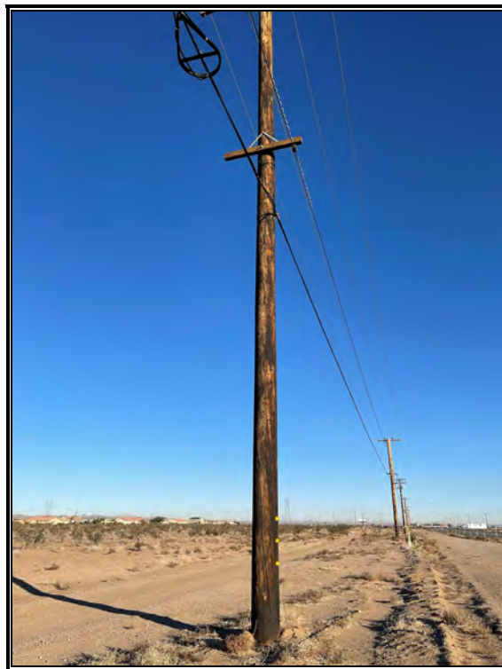
View north at existing utility pole on HWY 395 for AT&T proposed POC.
