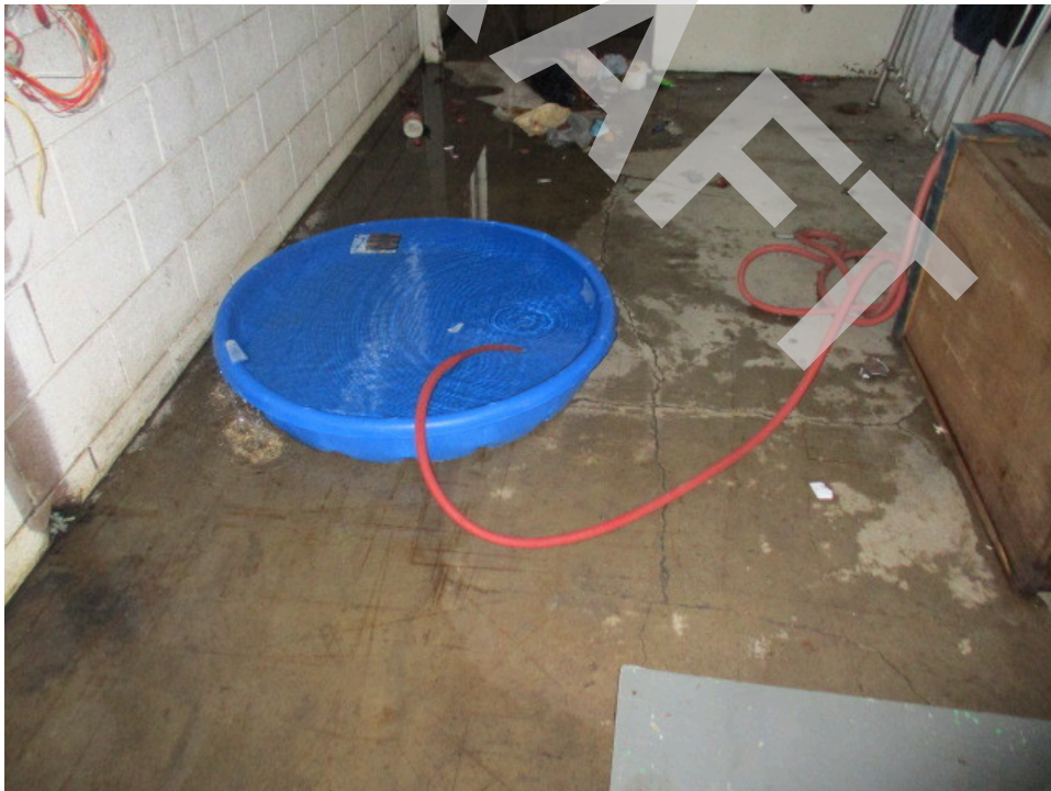
18. Standing water in the restroom/equipment building on the southwestern side of the subject property
