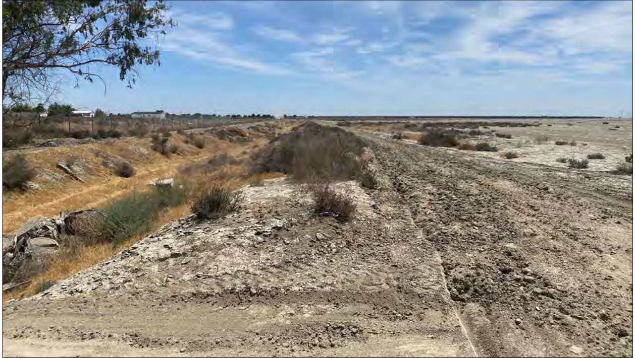
Figure 12. Photograph of a drainage ditch, oriented north-south, crossing the Avenue 36 alignment and the proposed sewer line pathway west of Allensworth Elementary School.
