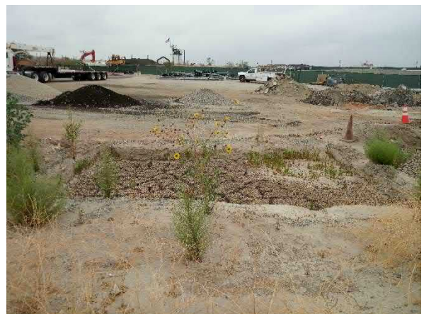
Photo #24 Concrete washout area inside a construction laydown yard located along the western site boundary.
