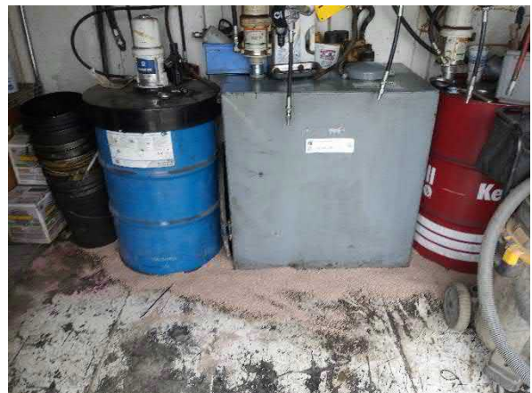
Photo #12 View of the approximately 100-gallon AST and 55-gallon drums containing motor oil located in the hazardous materials shed on Lot 35.
