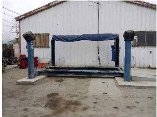
Photo #10 View of the aboveground hydraulic lift located adjacent to the maintenance garage on Lot 35.
