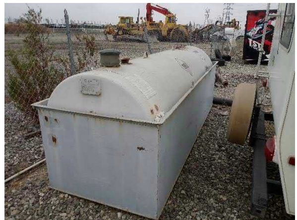
Photo #6 Empty and non-operation 1,000-gallon diesel fuel AST located on Lot 35.
