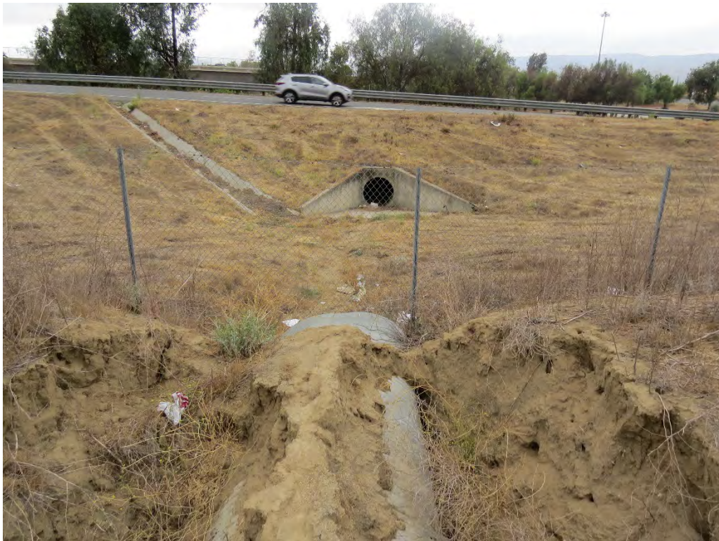
Photograph 18: Looking at the culvert that receives water flows from Drainage 2 and conveys water under Interstate 15.
