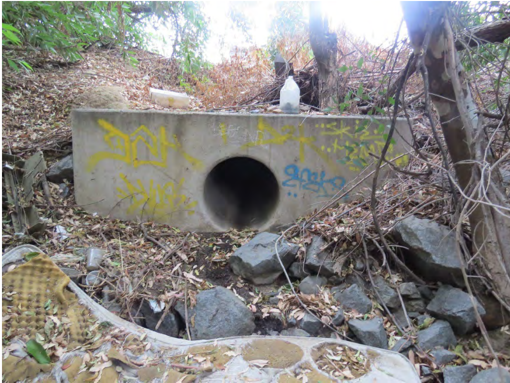
Photograph 21: One of the culverts that conveys flows into Drainage 1 on the southeast corner of the site.
