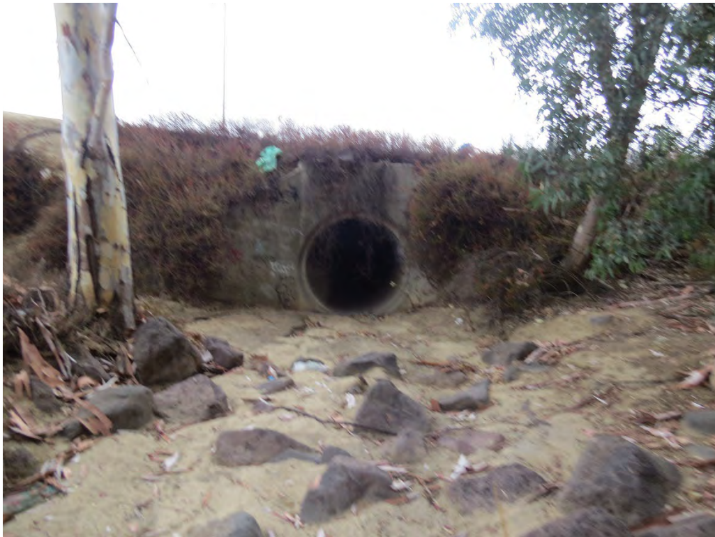
Photograph 26: Looking at the culvert at the western end of Drainage 1 that receives water flows from Drainage 1 and conveys under Murrieta Hot Springs Road.
