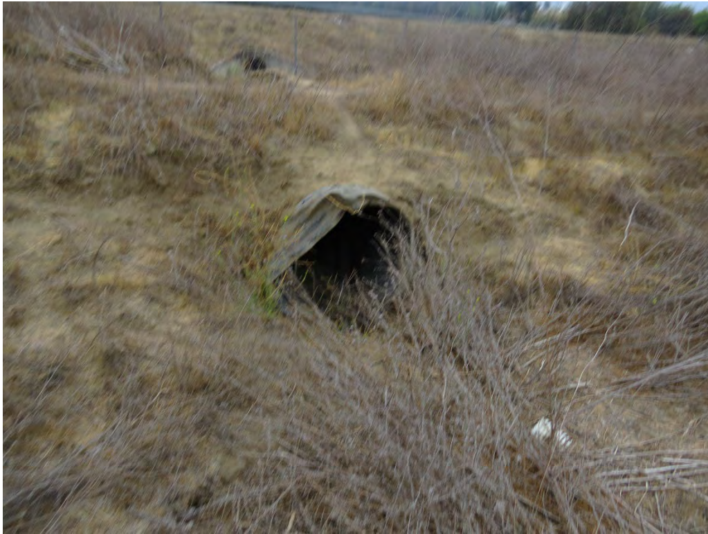
Photograph 17: 36-inch culvert that Drainage 2 flows into on the western boundary of the site.
