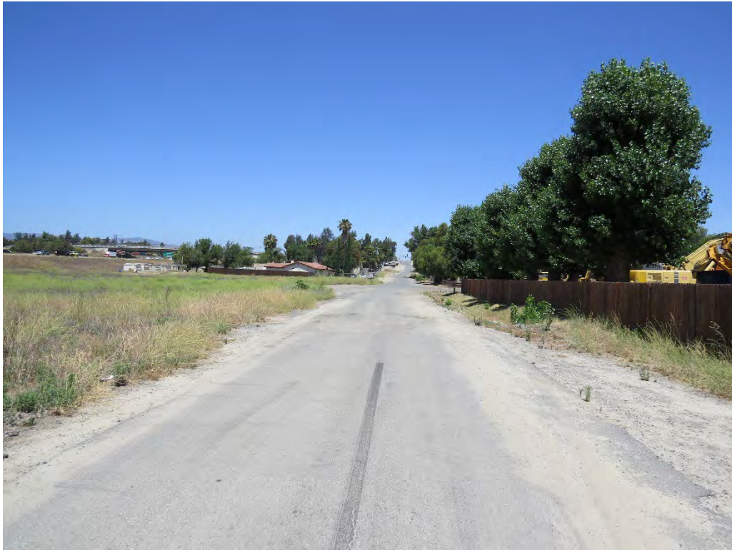
Photograph 31: Looking north along Monroe Avenue where street improvements will occur, north of the low water crossing.
