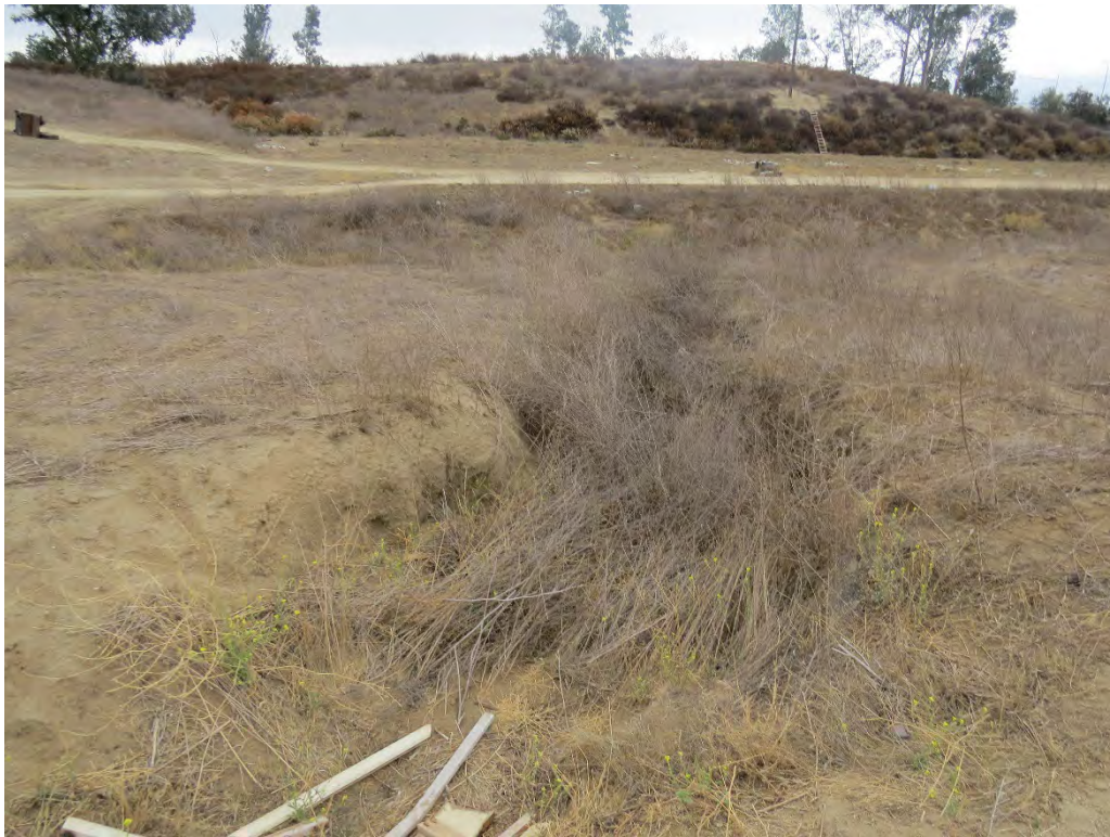
Photograph 14: Looking south at the area where the northern finger of Drainage 2 connects with the main drainage at the topographic low spot onsite.
