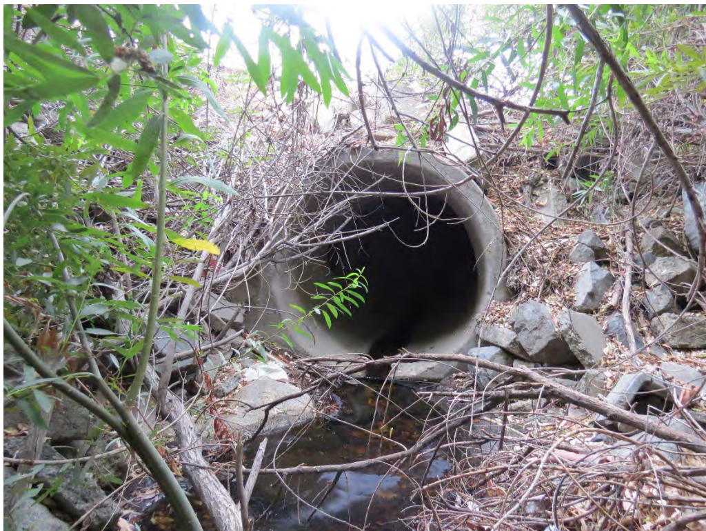
Photograph 19: Main culvert that conveys flows into Drainage 1 on the southeast corner of the site.
