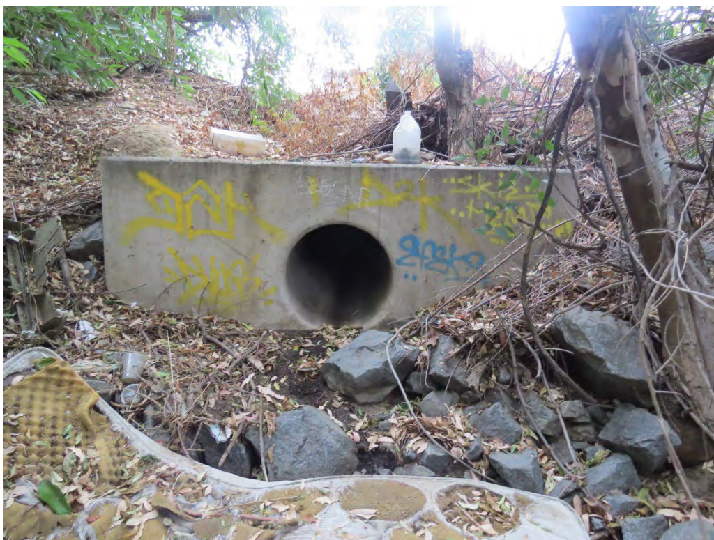
Photograph 12: One of the culverts that conveys flows into Drainage 1 on the southeast corner of the site.
