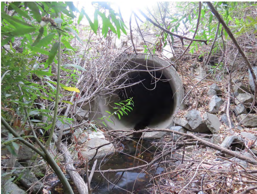
Photograph 11: Main culvert that conveys flows into Drainage 1 on the southeast corner of the site.
