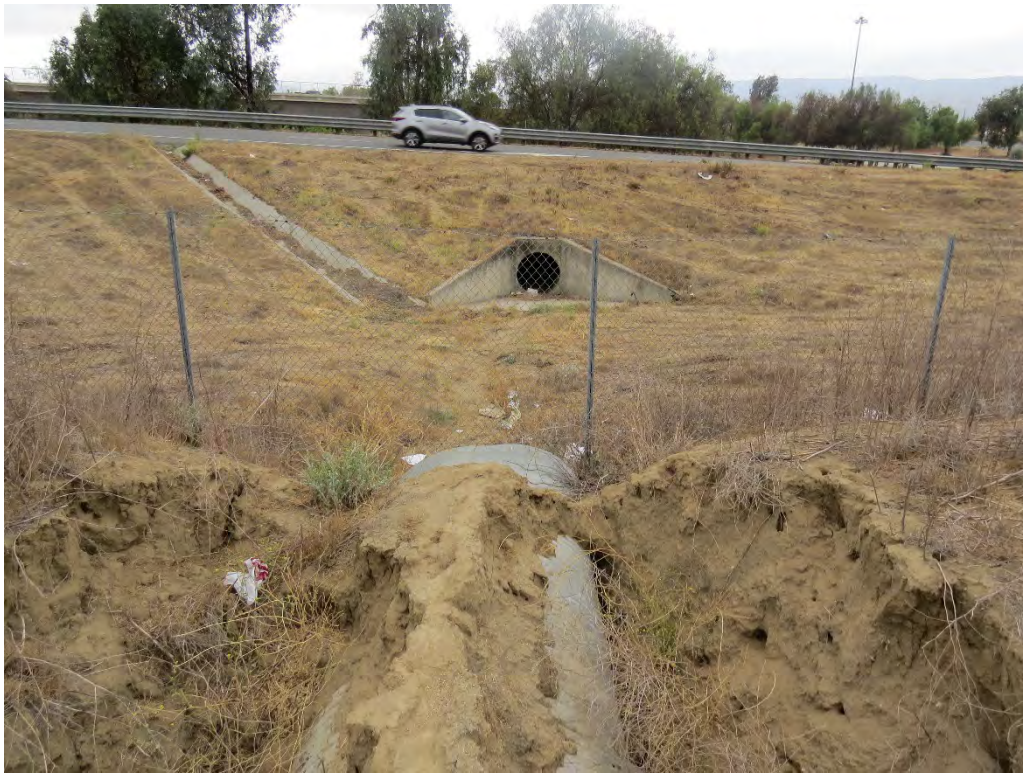
Photograph 9: Looking at the culvert that receives water flows from Drainage 2 and conveys water under Interstate 15.
