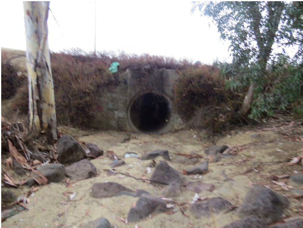
Photograph 17: Looking at the culvert at the western end of Drainage 1 that receives water flows from Drainage 1 and conveys under Murrieta Hot Springs Road.
