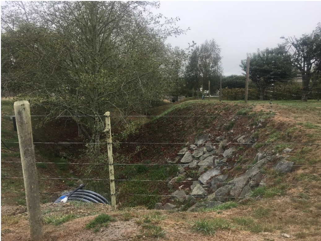
Photo 6. View north of Gravelly Point Creek outlet
