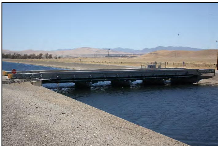
Photograph 58: View of 24-foot-wide County Highway Bridge at M.P. 96.28 along McCabe Road, with three concrete piers and concrete parapet walls with metal guard-rail extensions on both ends; camera facing downstream from left bank, June 13, 2022 (C0178).
