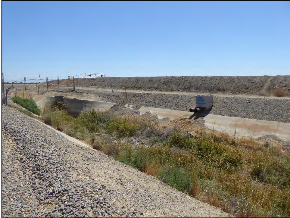
Photograph 6: Upstream view of San Luis Drain from right bank O&M road, with non-original inlet drain (center right) and Delta-Mendota Canal left-bank levee (background); camera facing east, July 20, 2022.
