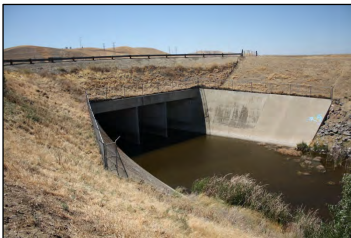
Photograph 104: Culvert channeling the O'Neill Forebay Wasteway beneath the DMC at M.P. 69.62; camera facing northwest, June 13, 2022 (C0214).
