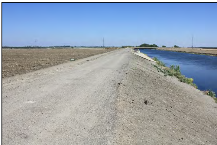
Photograph 15: View of embankment and maintenance road from approximately M.P. 111.28; camera facing downstream from left bank, June 14, 2022 (C0489).
