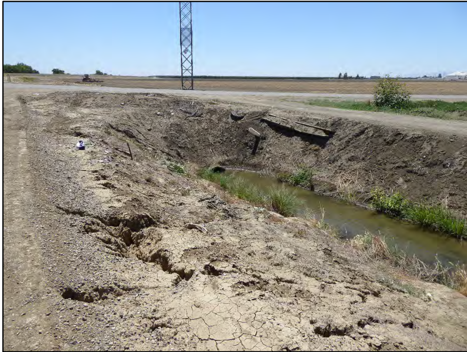
Photograph 8: Upstream view of Drain U-121.2 culvert undercrossing at Sierra Avenue; camera facing southeast, July 20, 2022.
