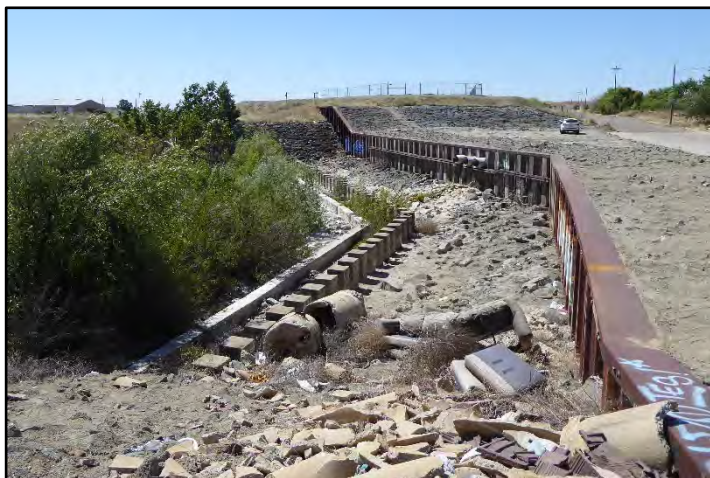
Photograph 254: Retaining wall around siphon and culvert that was repaired in 1995 after sheet piles were damaged in severe storm, fence around siphon outlet visible on elevated embankment in background (top center); camera facing south, May 13, 2022 (A00946).
