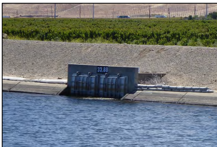
Photograph 50: Altered flap-gate style, concrete inlet drain along the right bank at M.P. 33.88; camera facing from left bank, May 11, 2022 (A00699).
