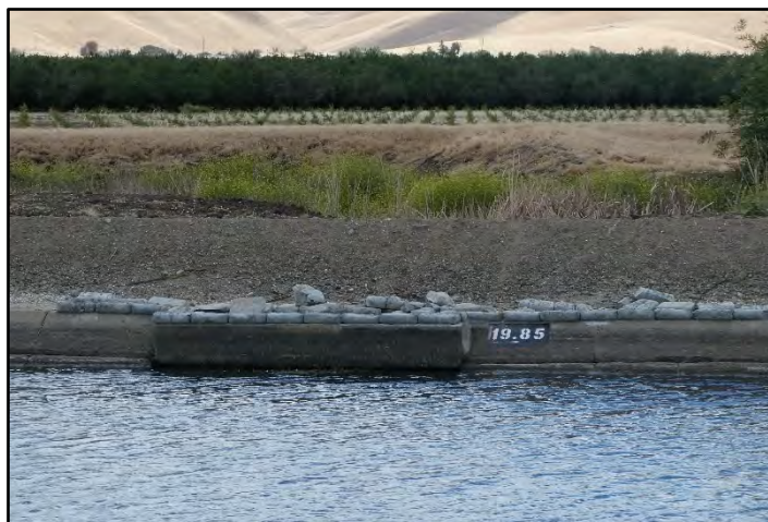
Photograph 158: View of sandbags lining the top of the canal wall at turnout site at M.P. 19.85; camera facing right bank from left bank, May 10, 2022. (B00070)
