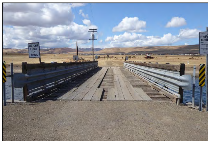
Photograph 67: Detail view of Farm Bridge with timber deck at M.P. 13.96, with its original timber handrails reinforced by the addition of corrugated steel sheets and modern steel guard-railings; camera facing southwest from left bank, May 10, 2022 (A00397).
