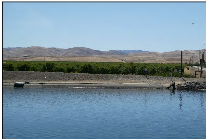
Photograph 239: Cracking in right bank canal lining between a large repair to canal wall just below Marshall Road bridge at M.P. 43.24 and drain inlet with flap gate on right bank at M.P. 43.26; camera facing right bank from left bank, May 12, 2022 (B00448).
