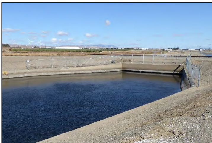
Photograph 141: South Pacific Railroad Siphon outlet headwall at M.P. 11.51; camera facing upstream from left bank, May 10, 2022 (A00353).
