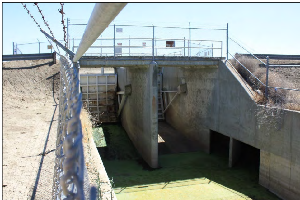
Figure 30: Radial gates at Firebaugh Wasteway's inlet structure; camera facing upstream from wasteway's right bank, June 14, 2022.
