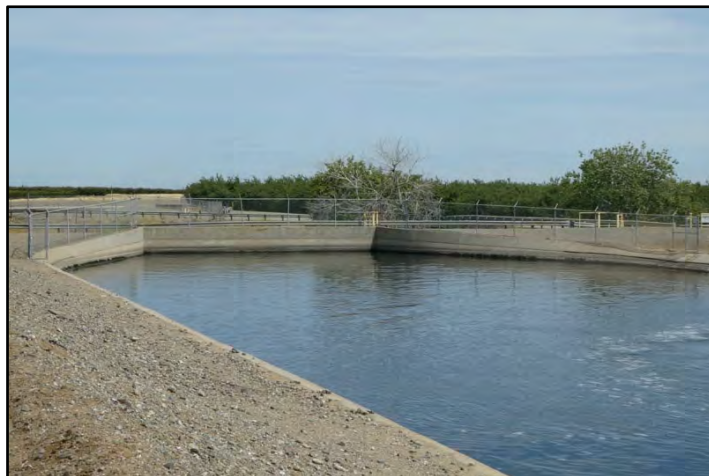
Photograph 214: Upstream view of siphon outlet headwall at M.P. 37.31; camera facing upstream from right bank, May 12, 2022 (B00252).
