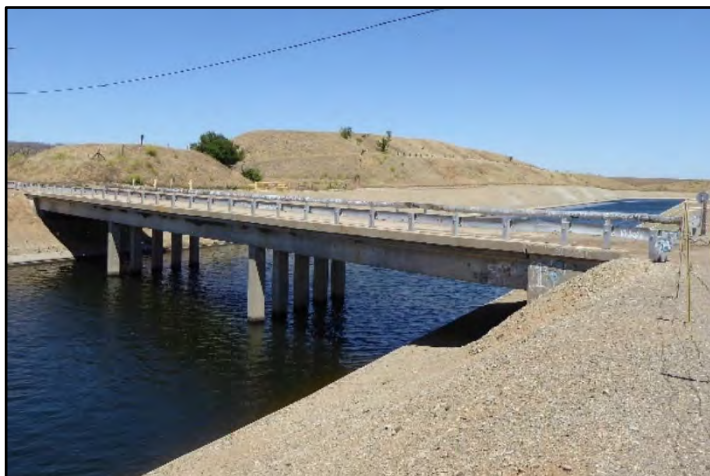
Photograph 56: Detail view of concrete bents supporting County Highway Bridge with concrete deck at M.P. 53.43 along Shiells Road; camera facing upstream from left bank, May 13, 2022 (A00979).
