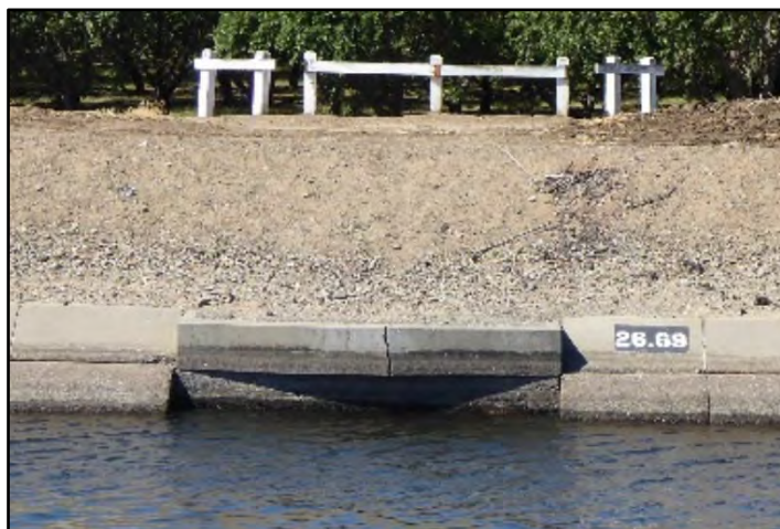
Photograph 180: Cracking on concrete lining around turnout at M.P. 26.69; camera facing right bank from left bank, May 11, 2022 (A00535).
