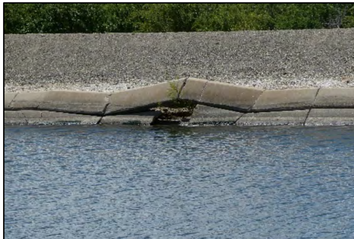
Photograph 156: New cracking at a repair to the canal lining at M.P.; camera facing right bank from left bank, May 10, 2022. (B00029)
