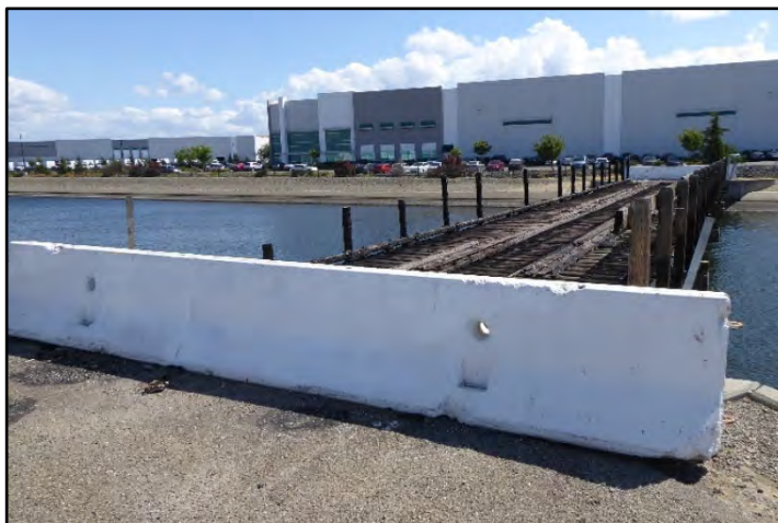
Photograph 70: View of fire-damaged Farm Bridge at M.P. 9.87, with timber deck and timber railing on upstream side; camera facing southwest from left bank, May 9, 2022 (A00297).
