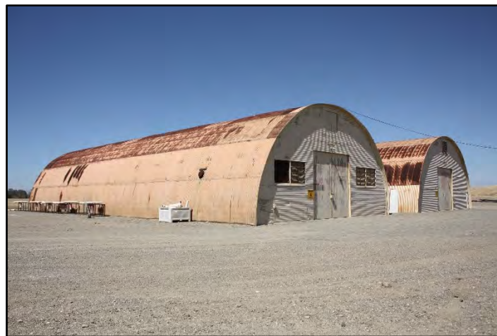
Photograph 294: Quonset huts in O&M yard approximately at M.P. 69.90; camera facing northeast, June 13, 2022 (C0223).
