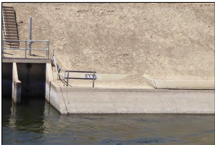
Photograph 13: View of concrete canal lining on right bank around double-barrel turnout at M.P. 3.54, lining has been raised on either side of the turnout, but the top of the original canal wall is unchanged immediately surrounding the structure; camera facing right bank from left bank, May 9, 2022 (A00203).
