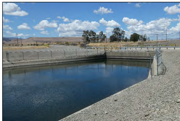
Photograph 154: Corral Hollow Creek Siphon outlet headwall at M.P. 16.34; camera facing upstream from left bank, May 10, 2022 (B0002).
