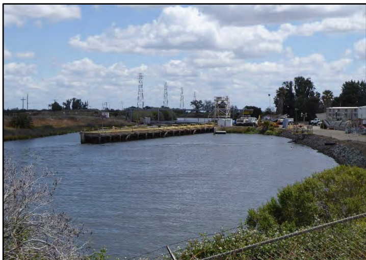
Photograph 2: View of riprap (right) and earth lining (left) at the beginning of Earth Section No. 1 of the Delta Mendota Intake Canal at the Tracy Fish Collection Facility, M.P. 0.09; camera facing upstream from left bank, May 9, 2022 (A00165).
