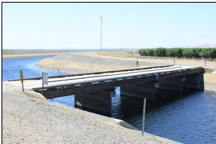
Photograph 68: View of Farm Bridge with timber deck at M.P. 85.47, where original timber handrails have been removed and not replaced; camera facing downstream from left bank, June 14, 2022 (C0338).
