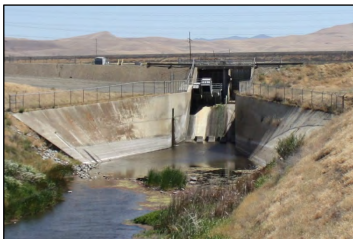
Photograph 290: Upstream view of the Volta Wasteway, with its inlet structure in the background; camera facing upstream from wasteway's left bank, June 13, 2022 (C0219).
