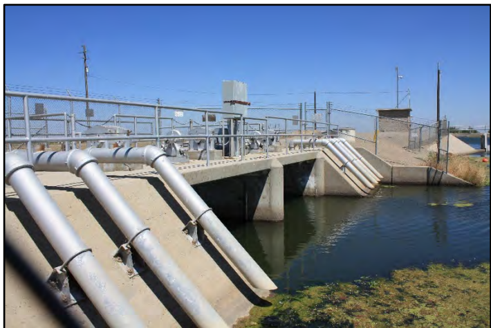
Photograph 355: Detail view of the Firebaugh Wasteway inlet structure at M.P. 111.22; camera facing downstream from left bank, June 14, 2022 (C0482).
