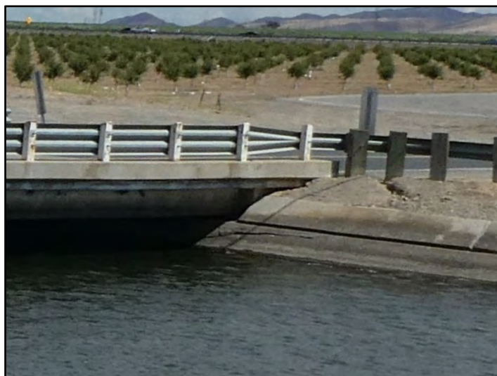
Photograph 171: Cracking in canal lining at right abutment of BRIDGE at M.P.; camera facing downstream from left bank, May 10, 2022 (B00116).
