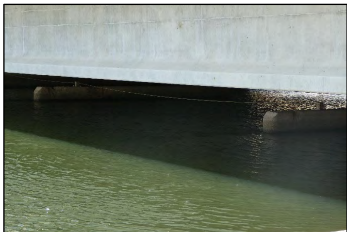
Photograph 232: Non-original replacement county highway bridge at M.P. 39.81 along Sperry Road/Hwy 130, with footings of the original bridge still evident underneath the current bridge; camera facing upstream from left bank, May 12, 2022 (B00350).
