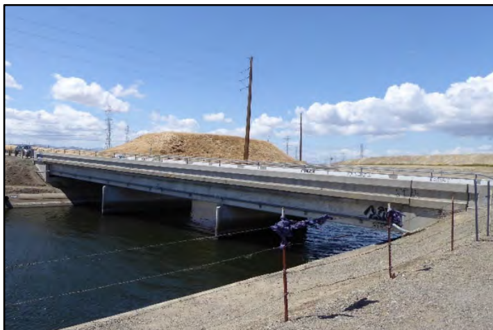
Photograph 82: View of 26-foot-wide State Highway Bridge at M.P. 6.6 along Old Highway 50, with replacement parapet walls with additional metal-pipe railing on top; camera facing upstream from left bank, May 9, 2022 (A00245).
