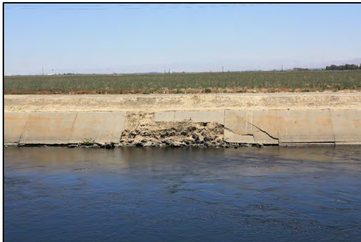
Photograph 339: Deteriorated concrete lining along right bank at approximately M.P. 96.82; camera facing right bank from left bank, June 14, 2022 (C0411).
