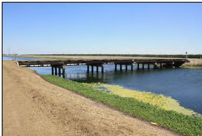
Photograph 71: View of 20-foot-wide Farm Bridge at M.P. 99.82, with original timber deck supported by five replacement concrete bents, with no handrails; camera facing downstream from left bank, June 14, 2022 (C0428).
