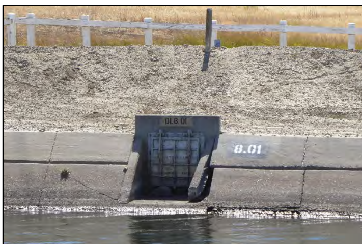
Photograph 49: Altered flap-gate inlet drain along the right bank at M.P. 8.01; camera facing from left bank, May 9, 2022 (A00266).
