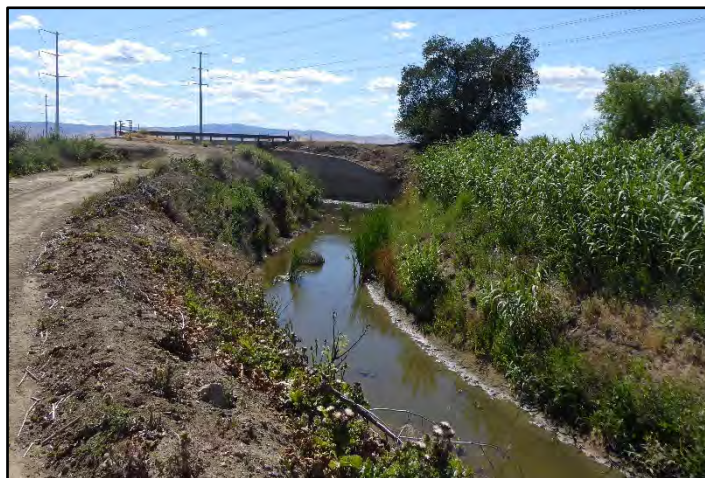
Photograph 195: Upstream view of earth section of Westley Wasteway around wasteway M.P. 3.85; camera facing upstream from wasteway’s right bank, May 11, 2022 (A00778).
