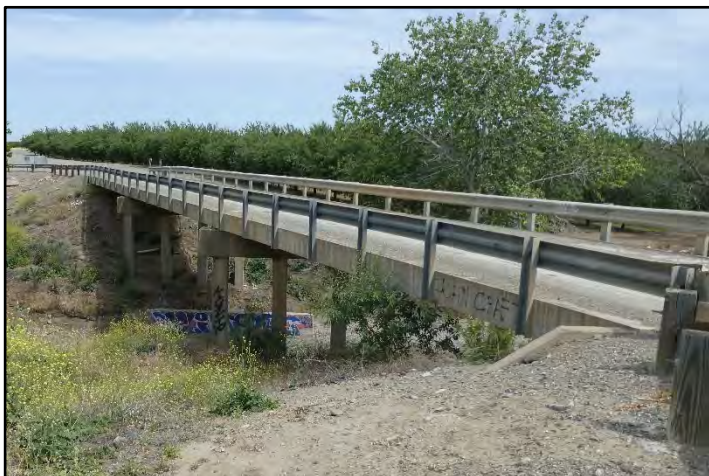
Photograph 78: View of Concrete Operating Bridge at M.P. 37.28 crossing over the Del Puerto Creek culvert; camera facing south from left bank, May 12, 2022 (B00257).
