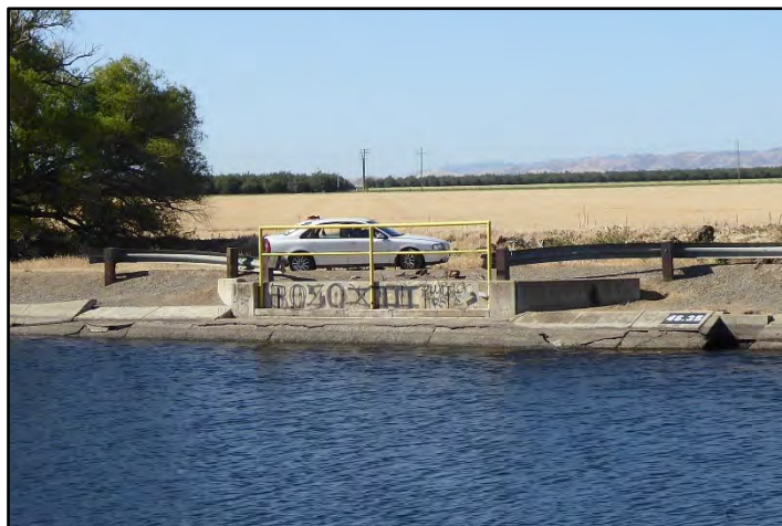
Photograph 244: Right abutment from a no longer extant farm bridge at M.P. 46.36, with cracking visible along the canal lining; camera facing right bank from left bank, May 13, 2022 (A00848).
