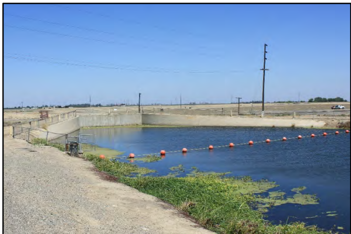
Photograph 351: Siphon inlet headwall at M.P. 110.96; camera facing downstream from left bank, June 14, 2022 (C0477).
