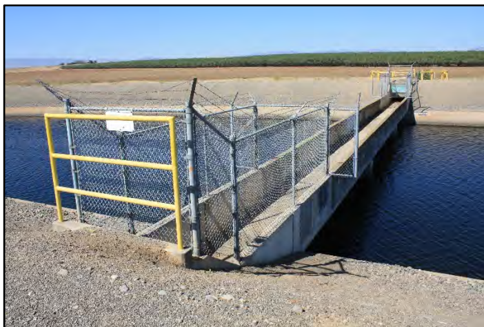
Photograph 43: Overchute at M.P. 78.59, showing the unreinforced box; camera facing right bank from left bank, June 14, 2022 (C0275).
