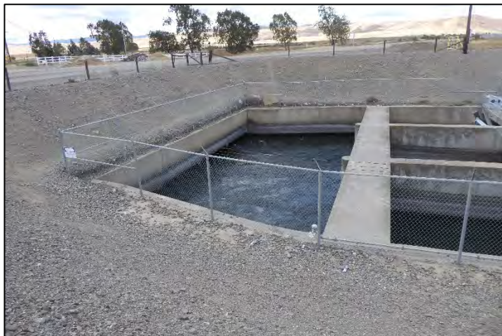
Photograph 151: Transition between Check No. 2 and Tracy Boulevard Siphon, showing the siphon's inlet headwall; camera facing right bank from left bank, May 10, 2022 (A00452).
