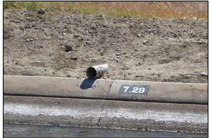
Photograph 52: CMP shoulder drain along the right bank at M.P. 7.29; camera facing from left bank, May 9, 2022 (A00258).
