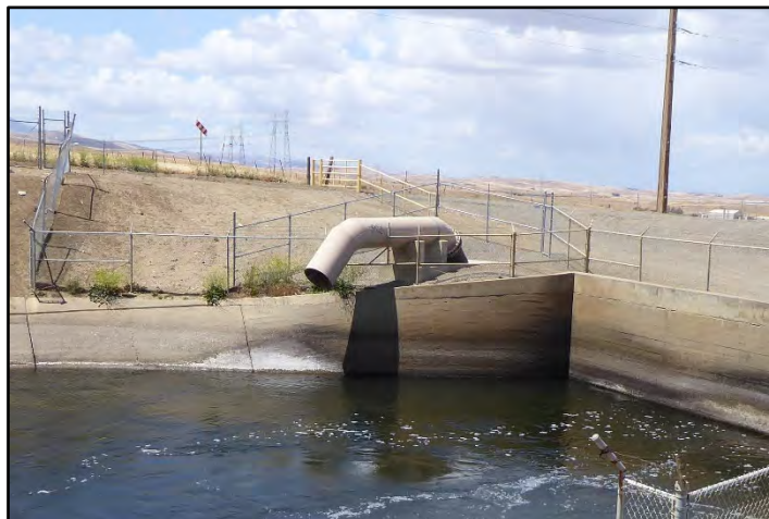
Photograph 125: View of BBID pump-in for Tracy Hills at M.P. 3.50, adjacent to discharge pipes inlet headwall (right); camera facing right bank from left bank, May 9, 2022. (A00199)
