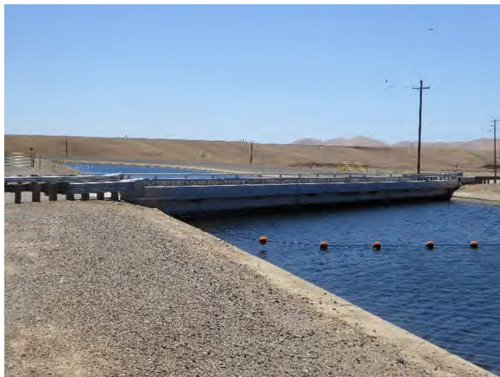
Photograph 271: View of concrete County Highway bridge at M.P. 56.60 along Pete Miller Road with parapet concrete walls, rather than the typical steel guard-rails; downstream from left bank, May 13, 2022 (A01027).
