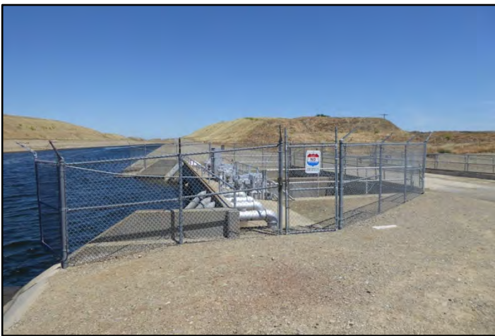
Photograph 31: Newman Wasteway inlet structure; camera facing upstream from left bank, May 13, 2022 (A00994).
