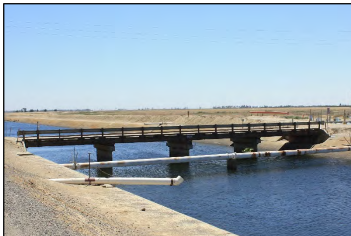
Photograph 69: View of Farm Bridge with timber deck at M.P. 93.24 which has only one modern steel guard-rail on the upstream side, but no handrail on the downstream side; camera facing downstream from left bank, June 14, 2022 (C0384).
