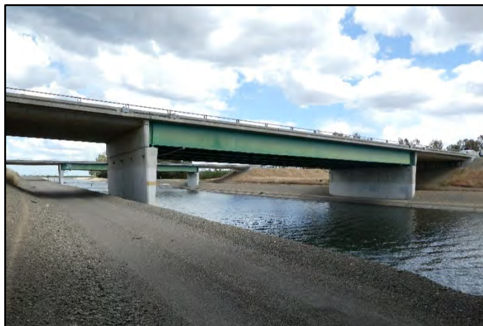
Photograph 89: View of non-original (post-1958) State Highway Bridge at M.P. 22.73, along State Highway 5 Northbound, with 50-foot-wide concrete deck supported by a steel stringer strung between two monolithic concrete piers, abutments further back in embankment; camera facing downstream from left bank, May 10, 2022 (B00162).
