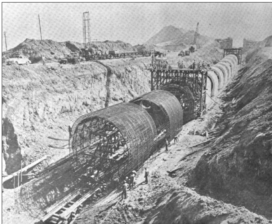
Figure 2: Construction of Mountain House Road Siphon showing concrete placement in progress, October 24, 1948.
