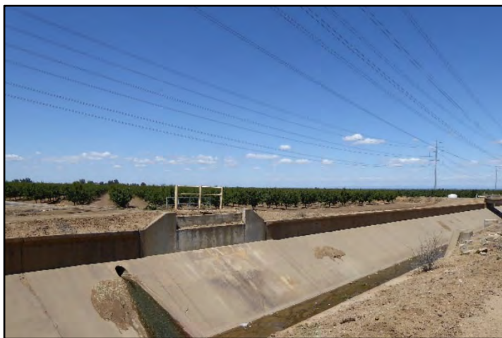
Photograph 192: View of wasteway concrete chute and missing bridge around M.P. 0.35 on the Westley Wasteway; camera facing downstream from right bank, May 11, 2022 (A00730).
