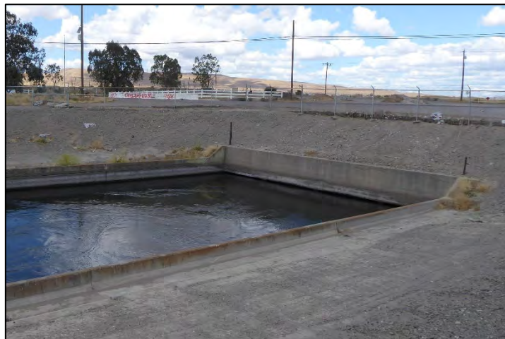
Photograph 152: Tracy Boulevard Siphon outlet headwall at M.P. 16.25; camera facing upstream from left bank, May 10, 2022 (A00454).
