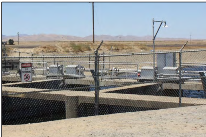
Photograph 277: Detail view of Check No. 11's gate hoisting equipment; camera facing upstream from left bank, June 13, 2022 (C0088).
