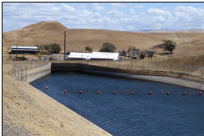
Photograph 22: Mountain House Road Siphon's inlet headwall at M.P. 4.41; camera facing downstream from left bank, May 9, 2022 (A00216).
