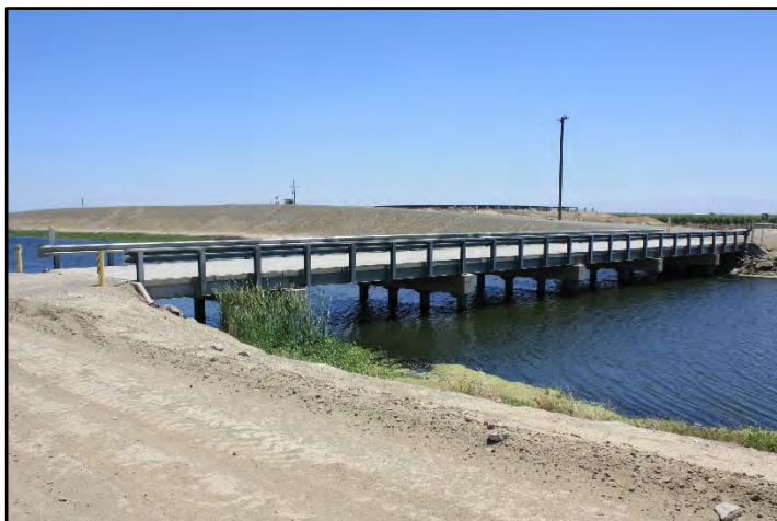
Photograph 92: View of replacement Farm Bridge built in 2004 at M.P. 106.58, with 20-foot-wide concrete deck, supported by five concrete bents; camera facing downstream from left bank, June 14, 2022 (C0460).
