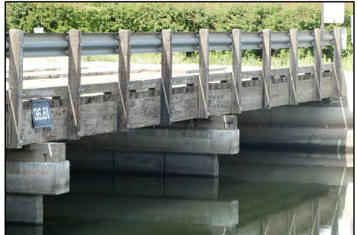
Photograph 77: Detail view of replacement concrete piers on Timber Operating Bridge at M.P. 36.81; camera facing southwest from left bank, January 16, 1948 (B00225).
