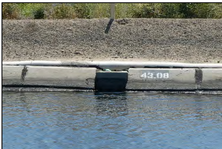
Photograph 236: Patches to right bank canal lining with fresh cracks visible around turnout at M.P. 43.08; camera facing right bank from left bank, May 12, 2022 (B00434).
