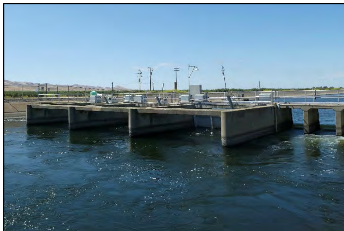
Photograph 242: Upstream view of Check No. 8; camera facing upstream from left bank, May 13, 2022 (B00457).
