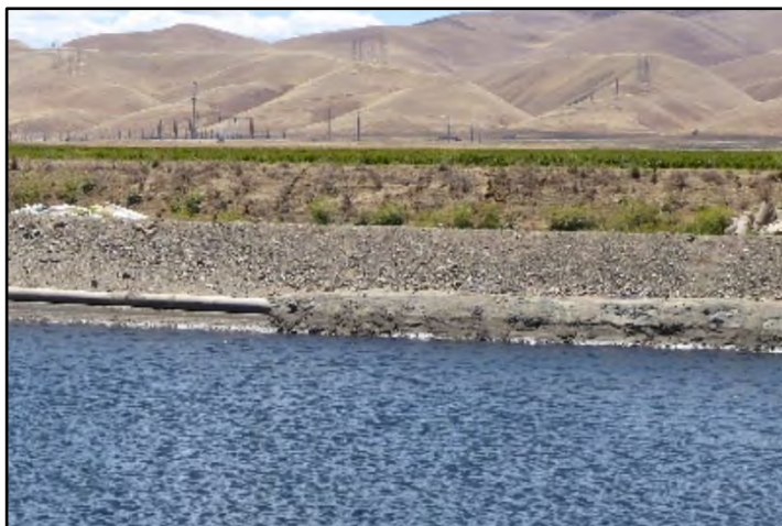
Photograph 202: View of patch to canal wall transitioning to bags laid on top of the concrete lining at approximately M.P. 33.71; camera facing right bank from left bank, May 11, 2022 (A00697).
