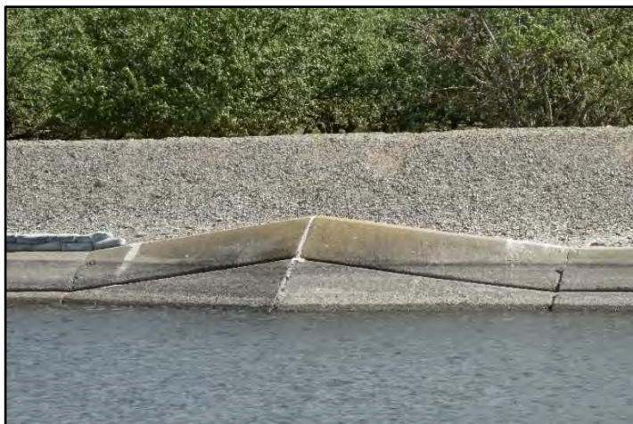
Photograph 172: View of repair to concrete lining around M.P. 22.90., with sandbags on top of wall downstream; camera facing right bank from left bank, May 10, 2022 (B00180).
