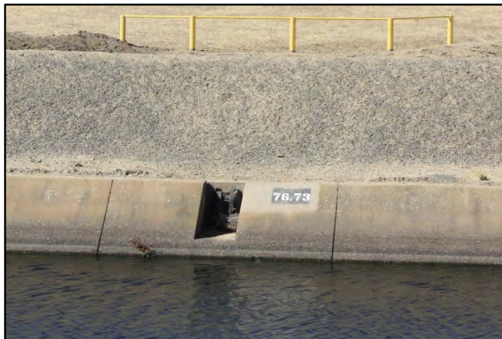
Photograph 48: Flap-gate inlet drain along the right bank at M.P. 76.64; camera facing from left bank, June 14, 2022 (C0253).
