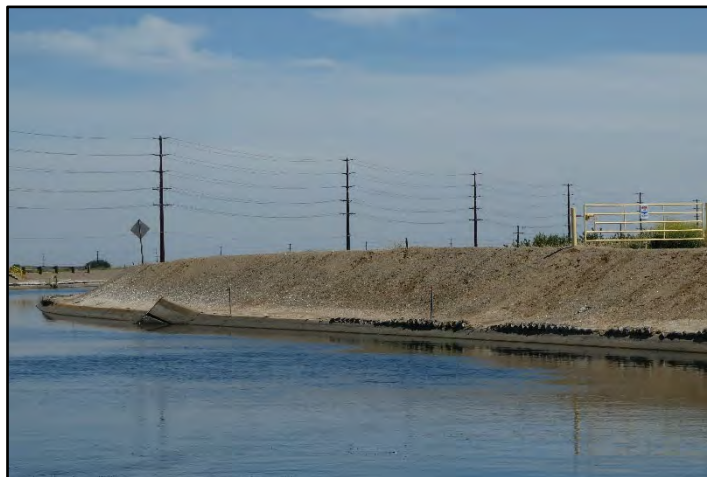
Photograph 235: Repairs to the right bank canal lining around M.P. 42.53; camera facing right bank from left bank, May 12, 2022 (B00426).
