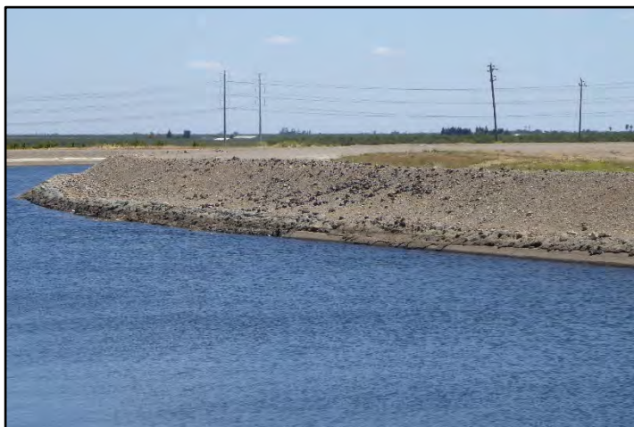
Photograph 200: View of large patch on right embankment above concrete lining at approximately M.P. 33.71; camera facing downstream from left bank, May 11, 2022 (A00693).
