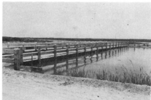
Fig. 7. Effect of Subsidence on Bridge at Near Capacity Flow
