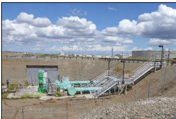
Photograph 145: View of overlining type turnout at M.P. 15.95, for the City of Tracy, Tracy Water Treatment Plant visible in background (upper right corner); camera facing upstream from left bank, May 10, 2022 (A00436).
