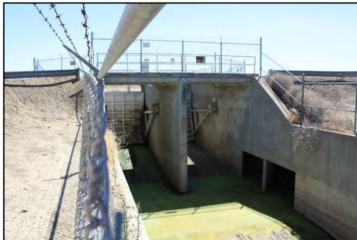
Photograph 354: Firebaugh Wasteway inlet structure at M.P. 106.58, showing the radial gates (center) and an outlet to one of the automatic-siphon spillways (bottom, right); camera facing upstream from the wasteway's right bank, June 14, 2022 (C0485).
