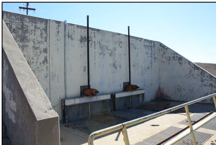
Photograph 309: Detail view of Wolfsen Bypass inlet structure along left bank at M.P. 76.04, showing the gates for each box-barrel-type turnout; camera facing east, June 14, 2022 (C0251).
