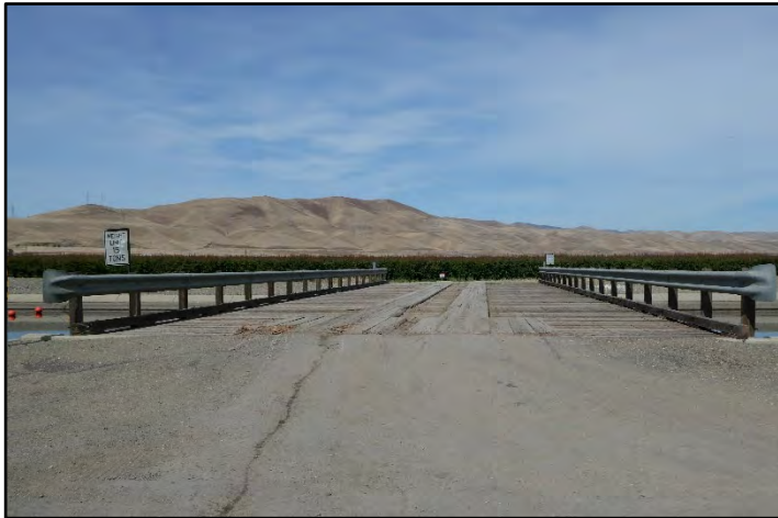
Photograph 76: Detail view of Timber Operating Bridge with 30-foot-wide deck at M.P. 36.81, with steel guard-rails; camera facing west from left bank, May 12, 2022 (B00226).
