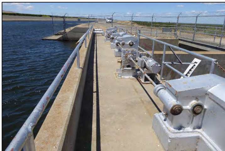
Photograph 188: Detail view of Westley Wasteway's inlet structure's top deck and gate-hoisting equipment; camera facing upstream from left bank, May 11, 2022 (A00713).
