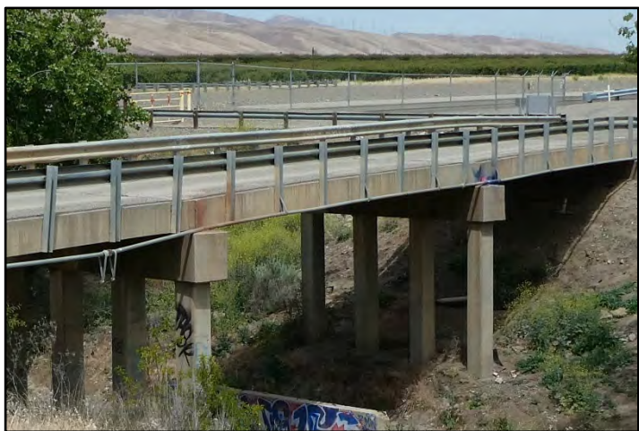
Photograph 211: Detail view of concrete bents on Operating Bridge at M.P. 37.28; camera facing northwest, May 12, 2022 (B00256).
