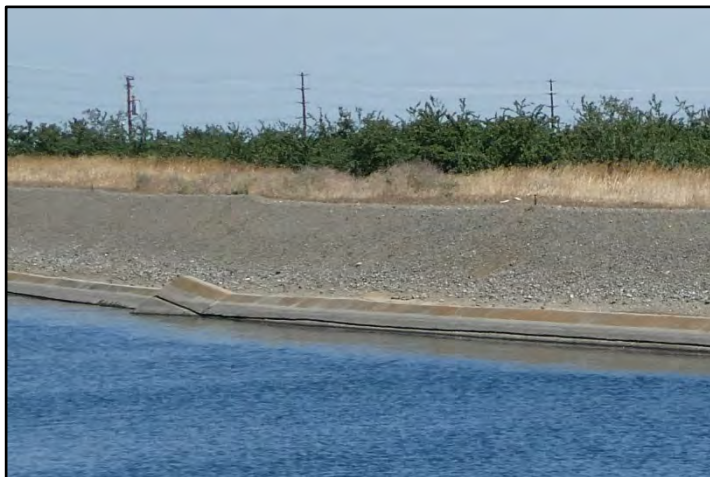
Photograph 234: Repair to the right bank canal lining around M.P. 42.3; camera facing right bank from left bank, May 12, 2022 (B00417).
