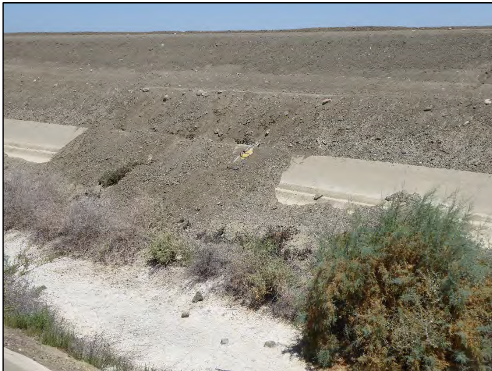
Photograph 11: Downstream view of San Luis Drain stainless steel safety ladder (partially obscured by erosion from the embankment); camera facing northwest, July 20, 2022.
