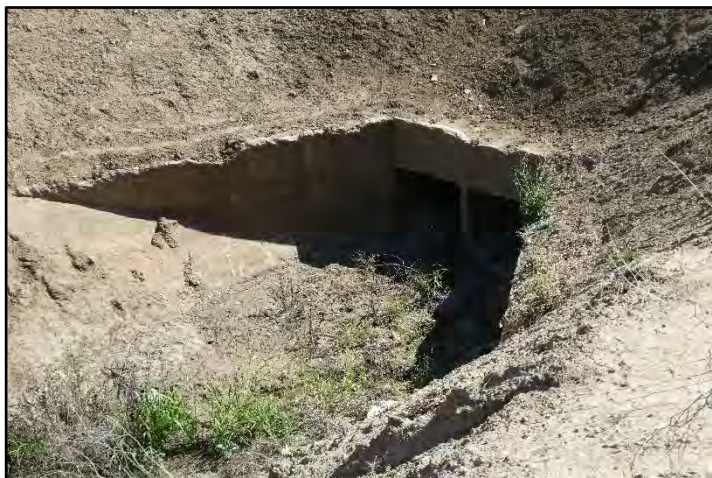
Photograph 102: Two-barrel siphon undercrossing outlet at M.P. 45.75 (left); camera facing southeast, May 12, 2022 (B00475).
