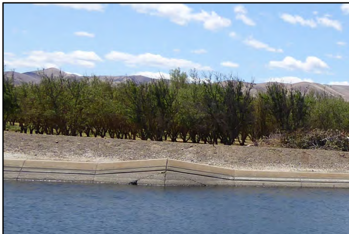
Photograph 198: View of a new crack on a repair to the canal wall near M.P. 30.63; camera facing right bank from left bank, May 11, 2022 (A00634).
