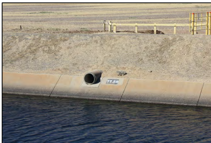
Photograph 46: Free-flowing inlet drain along the right bank at M.P. 77.58; camera facing from left bank, June 14, 2022 (C0261).
