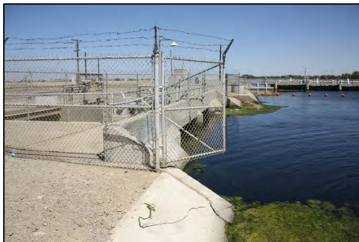
Photograph 288: Volta Wasteway's inlet structure at M.P. 69.98, with Check No. 13 in the background; camera facing downstream from left bank, June 13, 2022 (C0194).
