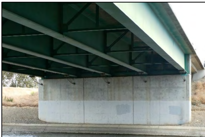
Photograph 88: Detail view of steel stringers and interior trusses on non-original (post-1958) State Highway Bridge at M.P. 22.73, along State Highway 5 Northbound; camera facing south from left bank, May 10, 2022 (B00165).
