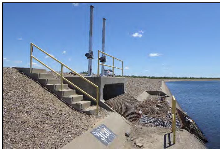
Photograph 197: Concrete box turnout at M.P. 31.31; camera facing downstream from left bank, May 11, 2022 (A00645).
