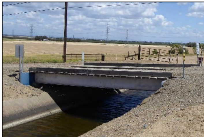
Photograph 121: View of bridge crossing over Irrigation Canal 120, around M.P. 3.12; camera facing east, May 9, 2022. (A00181)
