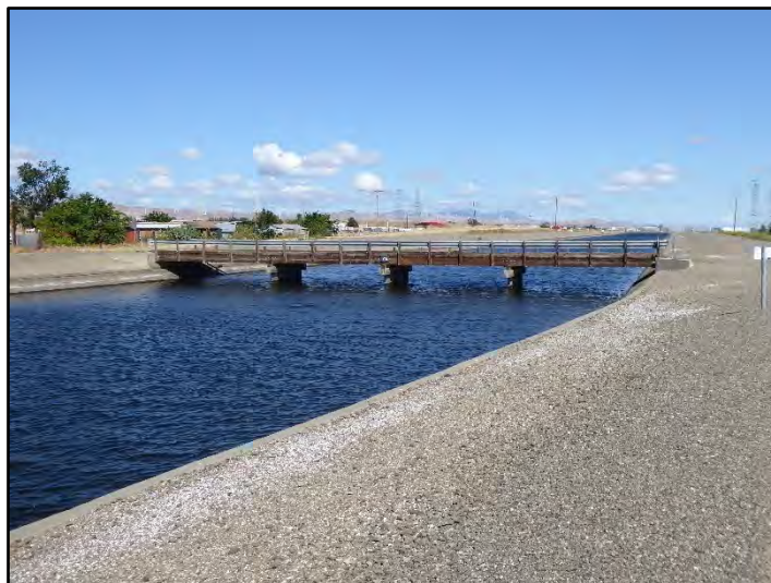
Photograph 65: View of Farm Bridge at M.P. 12.31 with 16-foot-wide timber-deck, replacement concrete piers, and modern steel guard-rails; camera facing upstream from left bank, May 10, 2022 (A00365).
