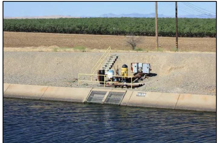
Photograph 38: Modern, two-barrel concrete pipe turnout along right bank at M.P. 78.56; camera facing from left bank, June 14, 2022 (C0270).
