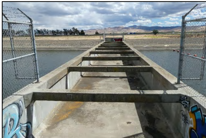
Photograph 42: Overchute at M.P. 21.91, showing the reinforced box; camera facing right bank from left bank, May 10, 2022 (B00127).
