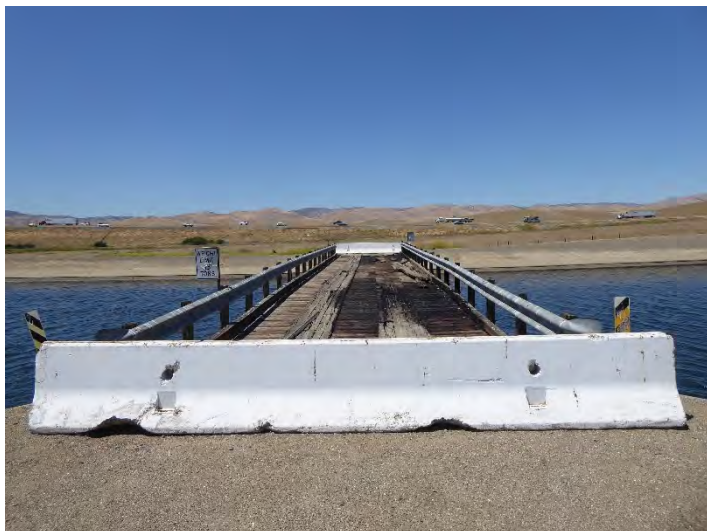
Photograph 270: Detail view of fire damaged deck of Operating Bridge at M.P. 56.02; right bank from left bank, May 13, 2022 (A01020)
