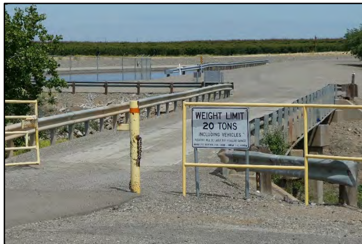
Photograph 210: View of concrete deck on Operating Bridge at M.P. 37.28; camera facing right bank from left bank, May 12, 2022 (B00255).
