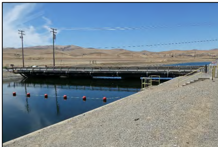
Photograph 55: View of 30-foot-wide County Highway Bridge with concrete deck at M.P. 39.21 along Rogers Road; camera facing upstream from left bank, May 12, 2022 (B00336).
