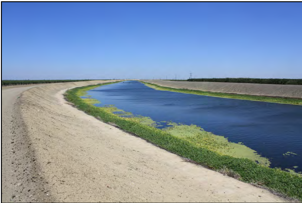
Figure 30: View of earth-lined section of canal from approximately M.P. 104.22; camera facing downstream from left bank, June 14, 2022.
