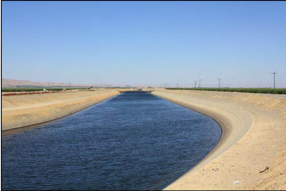
Figure 29: View of concrete-lined section of canal from approximately M.P. 91.36; camera facing upstream from left bank, June 14, 2022.
