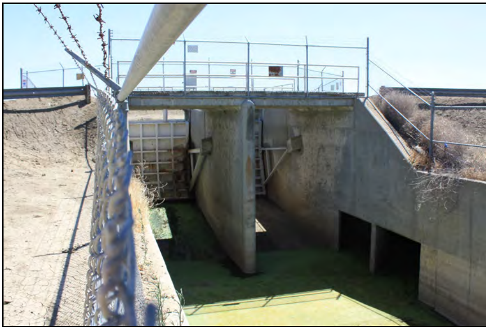
Figure 39: Radial gates at Firebaugh Wasteway's inlet structure; camera facing upstream from wasteway's right bank, June 14, 2022.
