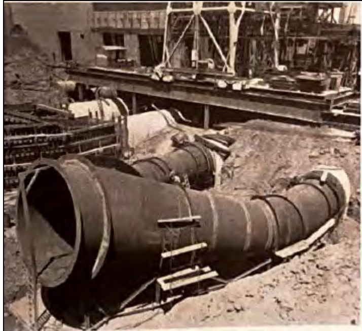
Figure 9: One of six 84-in. vertical shaft bottom suction twin volute centrifugal pumps. 44
