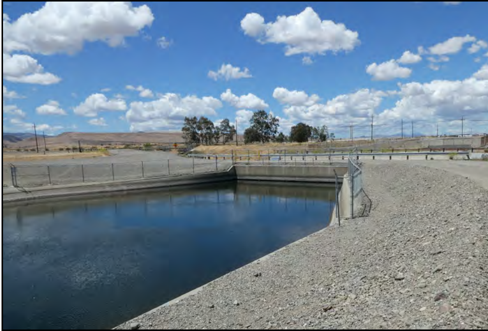
Figure 36: Four-barrel siphon outlet headwall at M.P. 16.34; camera facing upstream from left bank, May, 10, 2022.
