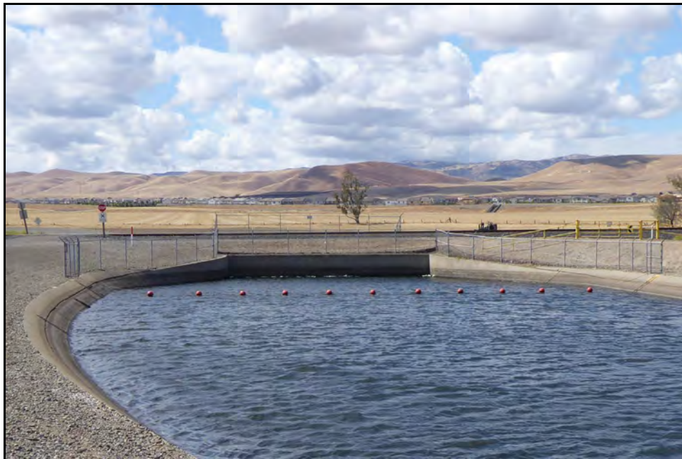
Figure 35: Three-barrel siphon inlet headwall at M.P. 13.67; camera facing downstream from left bank, May 10, 2022.
