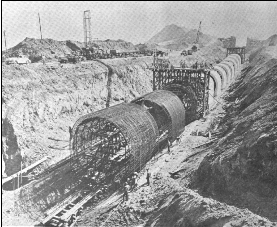
Figure 4: Construction of Mountain House Road Siphon showing concrete placement in progress, October 24, 1948. [130]
