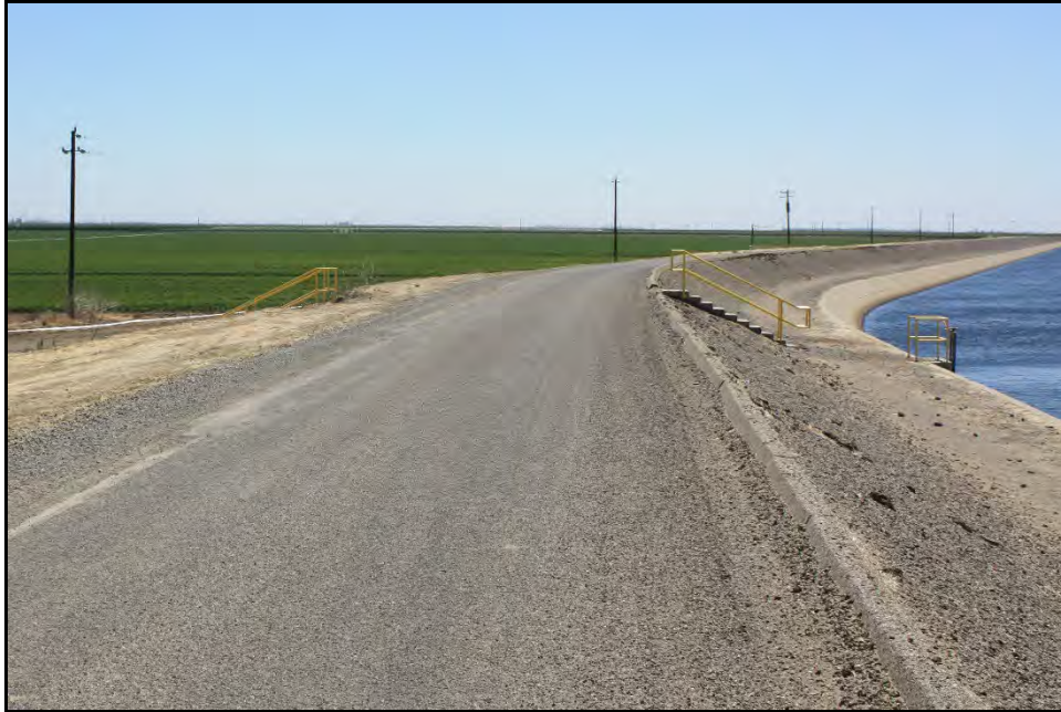
Figure 31: View of embankment and concrete-lined section of canal; camera facing downstream from left bank, June 14, 2022.
