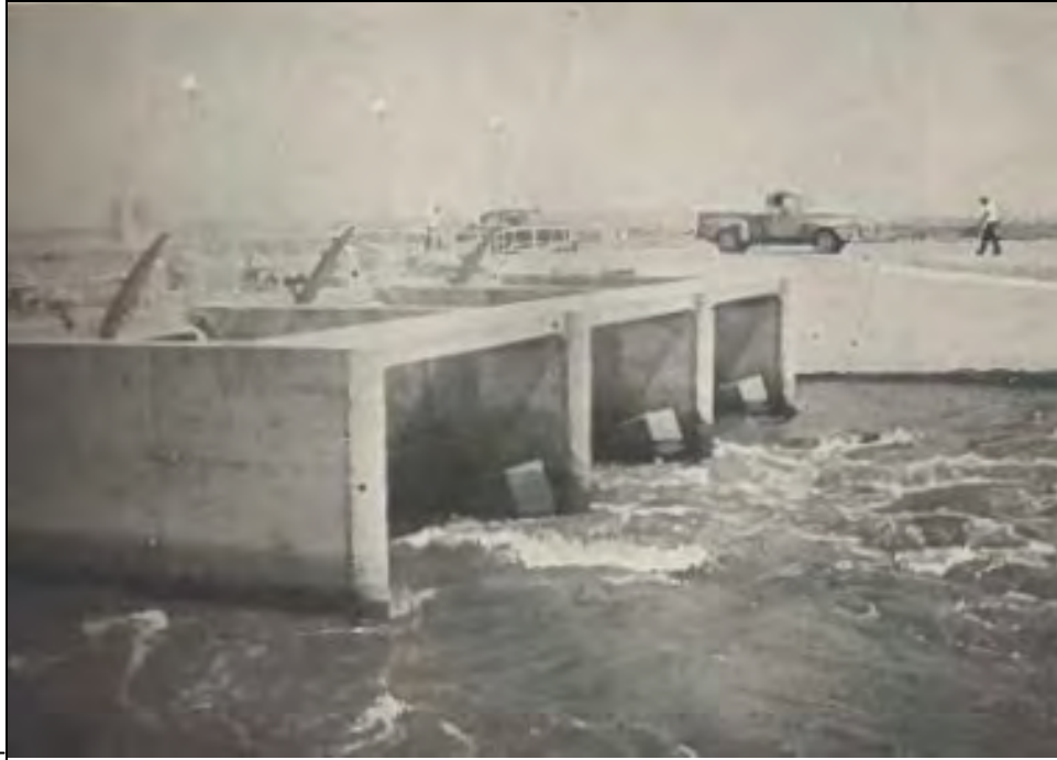
Figure 20: Note rough silty water below gates at Check No. 19, May 16, 1970. 74
