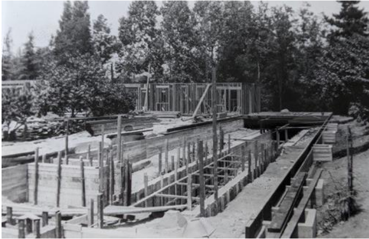
View of Central Block and North Wing (La Casa Soñada) Under Construction, 1939. Source: Chris Morrison.
