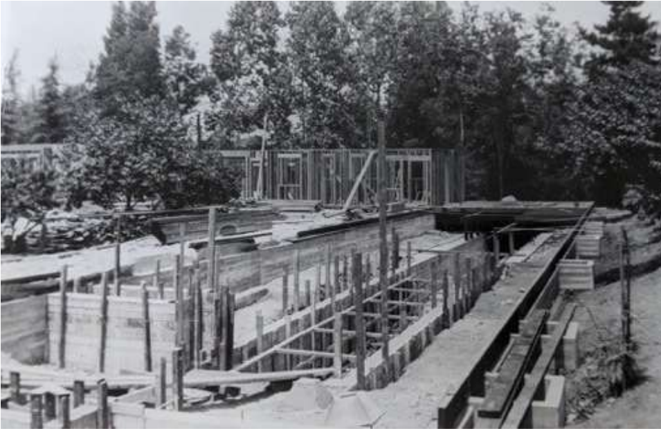
View of Central Block and North Wing (La Casa Soñada) of Morrison House Under Construction, 1939. Source: Chris Morrison.
