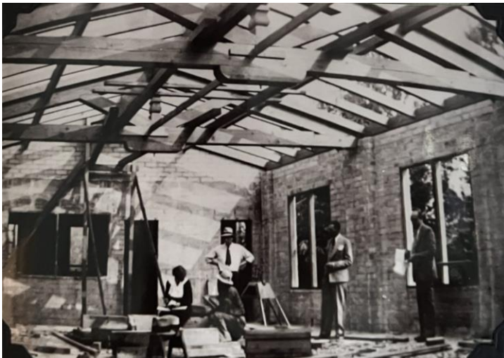
Construction of South Wing (El Sueño) of Morrison House, Lucile Morrison with builders, 1935. Source: Westminster Gardens.
