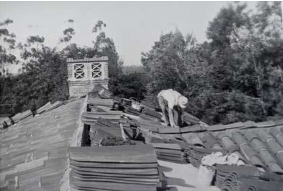
Roofing North Wing (La Casa Soñada) of Morrison House, 1939. Source: Chris Morrison.
