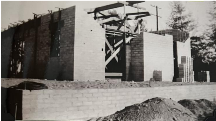
Construction of South Wing (El Sueño) of Morrison House, 1935. Source: Westminster Gardens.
