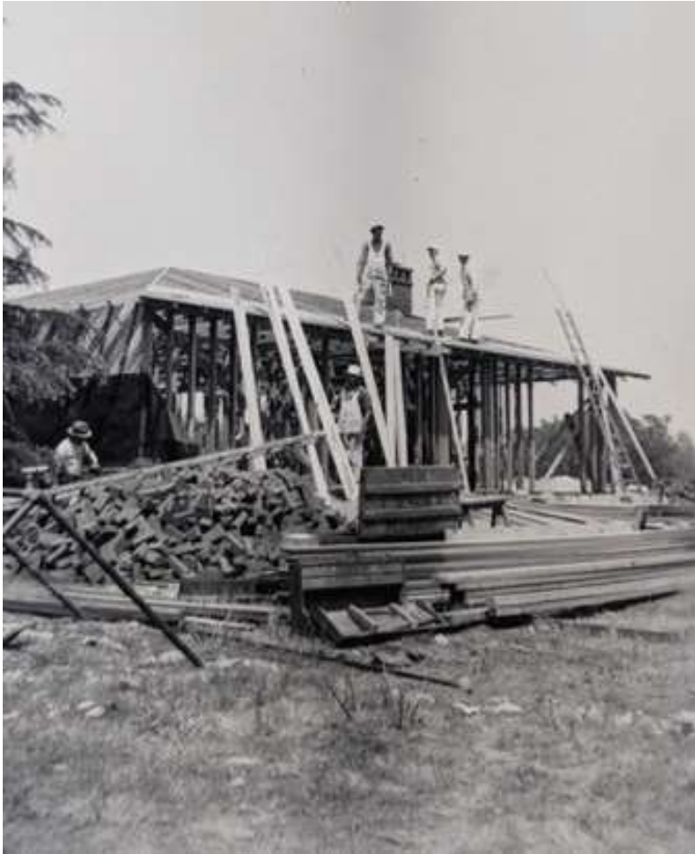
North Wing (La Casa Soñada) of Morrison House Under Construction, 1939. Source: Chris Morrison.
