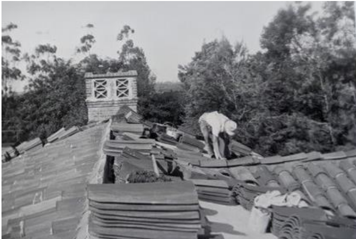
Roofing North Wing (La Casa Soñada) of Morrison House, 1939. Source: Chris Morrison.
