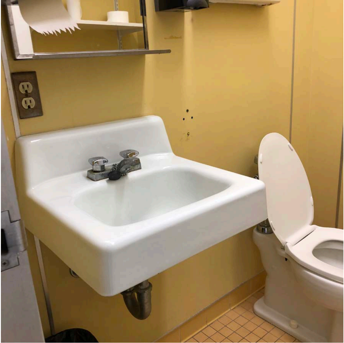
Restroom ceramic cove base contains lead. Yellow ceramic floor tile was found to be negative for lead.
