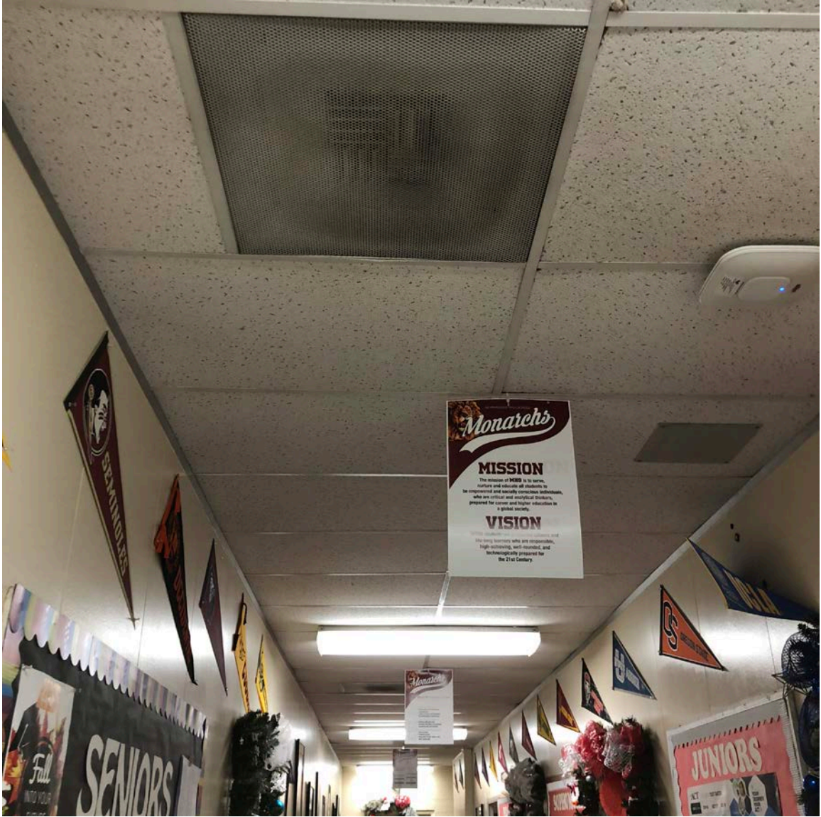
Building A light fixtures contained ballasts labeled “NO PCBs”
