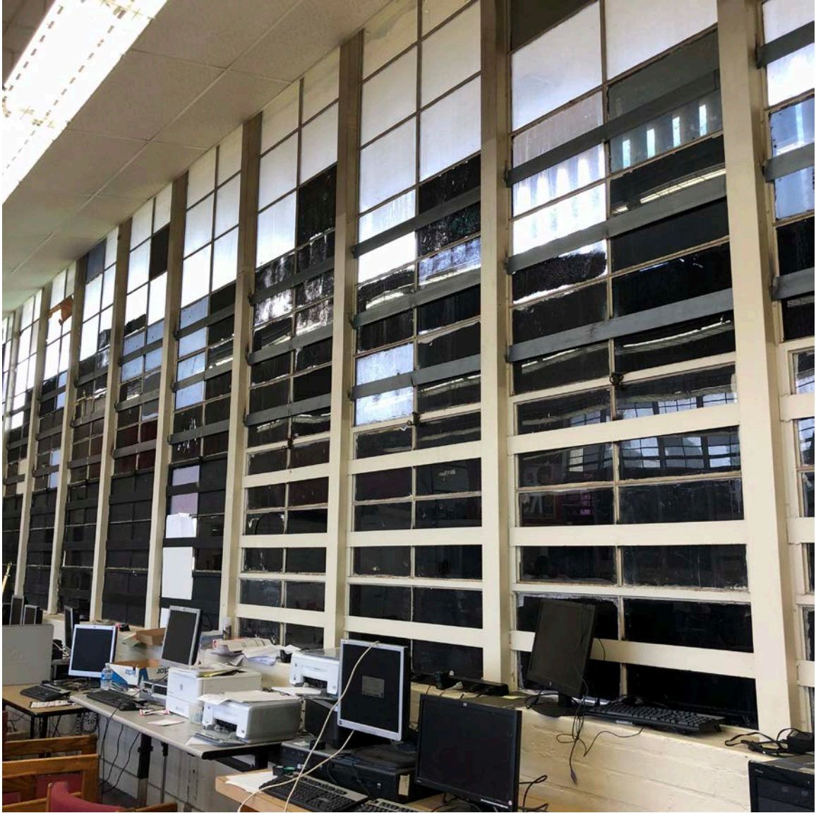
White window and window frame paint is lead based.
