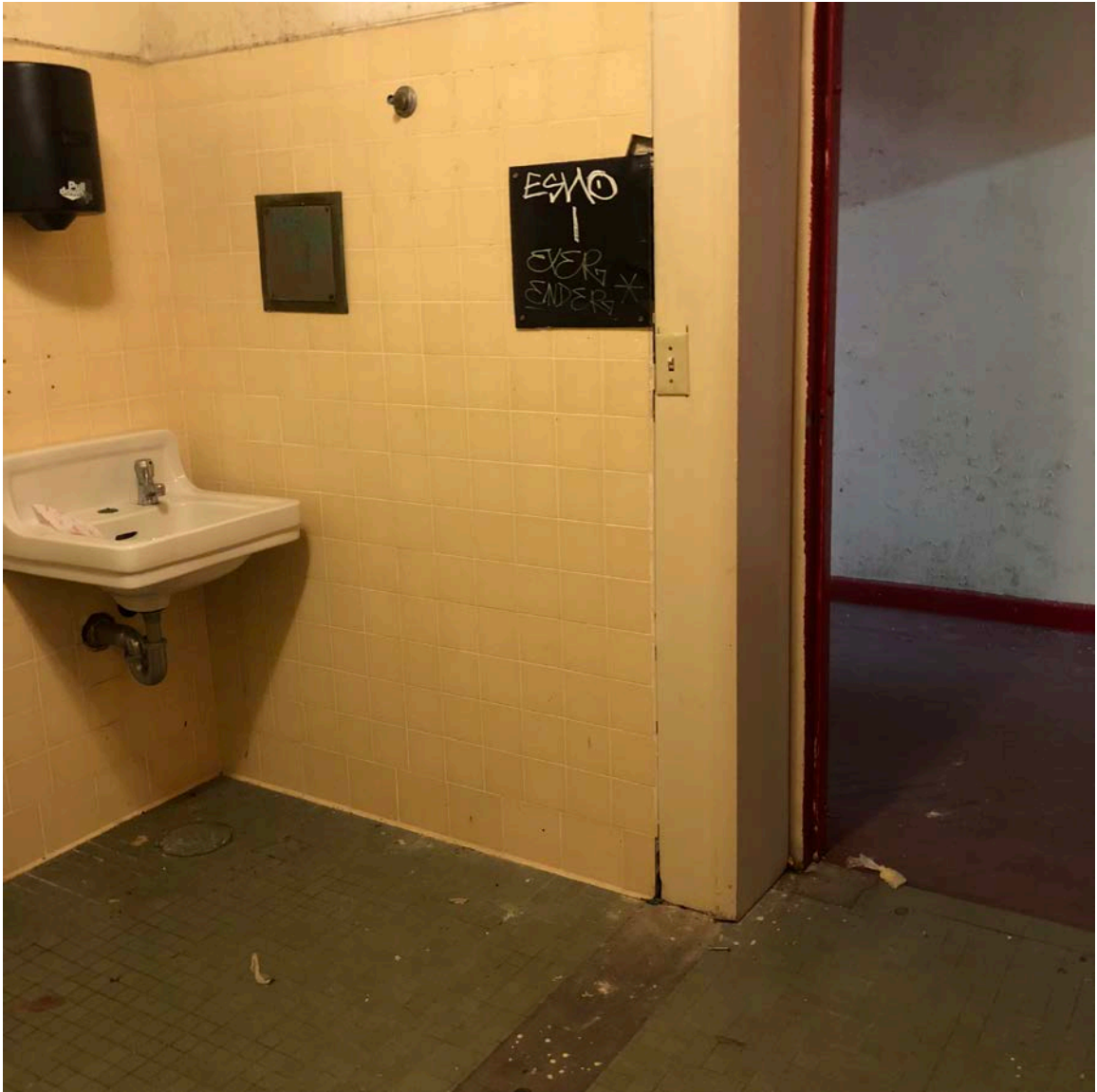
Beige 4-inch wall tile in the restrooms contains lead. Green 1-inch floor tile was negative.
