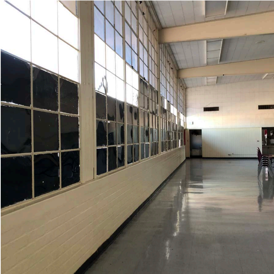
White window paint in Building R is lead-based.
