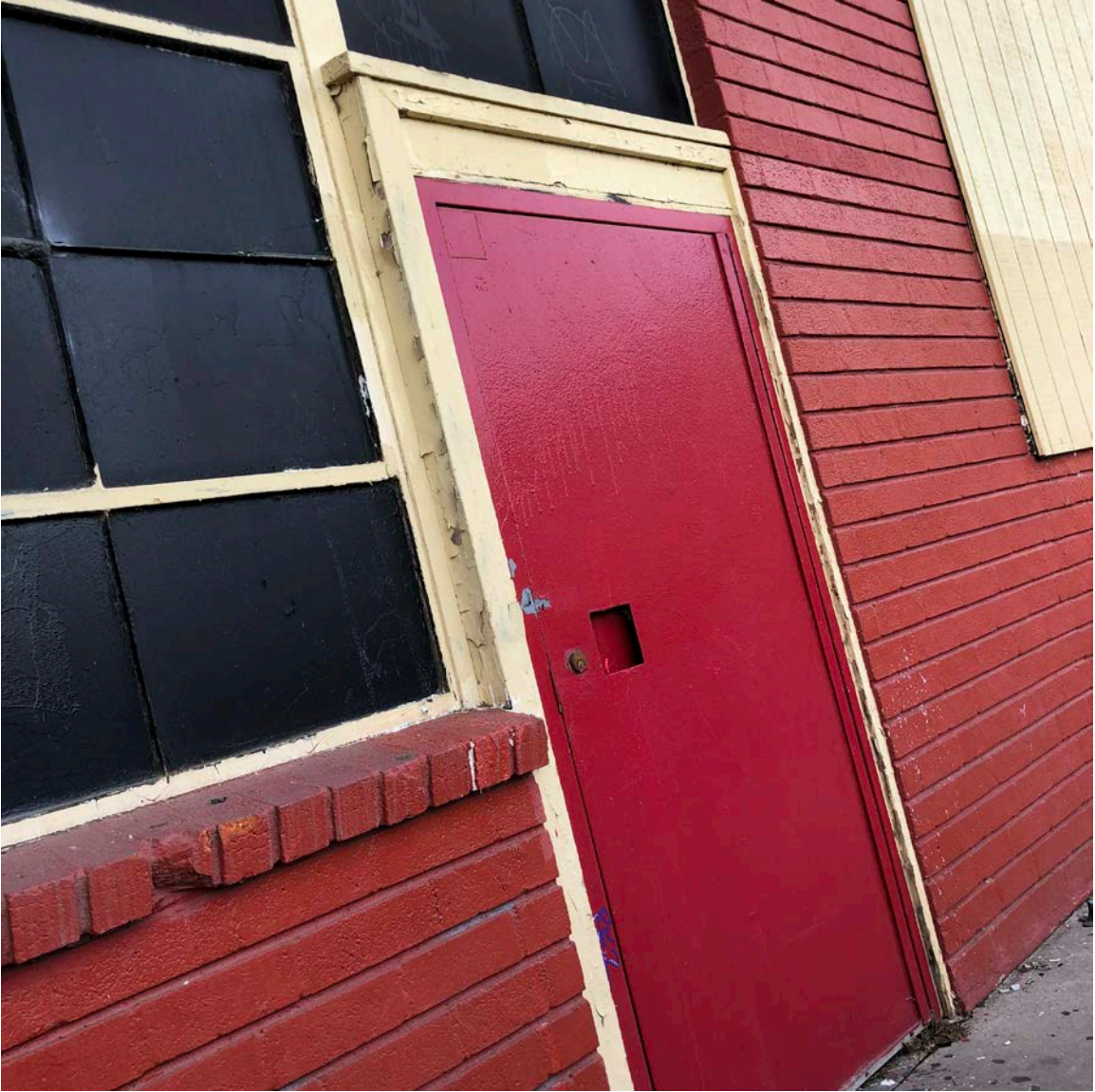
Wooden exterior door frame is coated with yellow lead-based paint.
