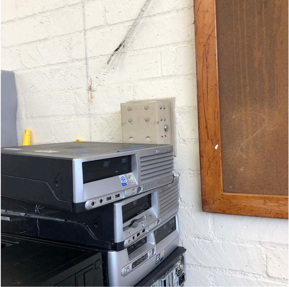
Mercury containing thermostat in classroom H3.
