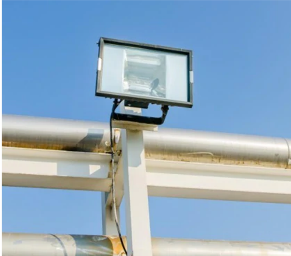
Figure 7 - Existing Building Mounted Flood Lighting
