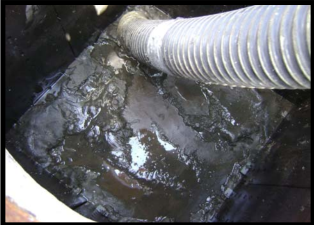
Sediment Chamber Is Vacuumed Clean Of All Accumulated Sediment And Associated Pollutants.
