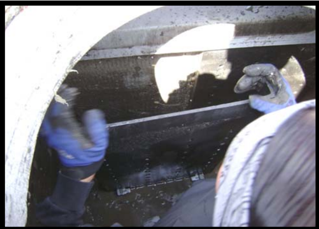
Filter Media Shields Are Removed To Expose BioMediaGREEN Filter Media To Be Cleaned Or Replaced.
