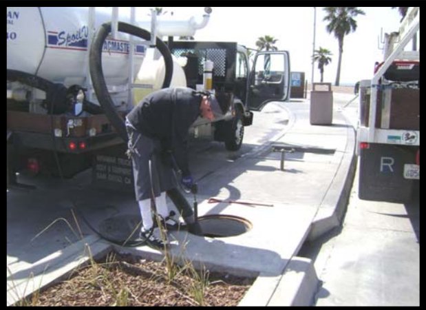
Assess Condition and Pollutant Loading. A Few Gallons Of Water Are Sprayed Into Sediment Chamber To Allow Sediment To Be Vacuumed.
