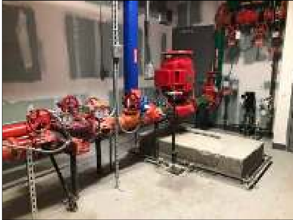
Photo 27: View of the fire riser (basement level).
