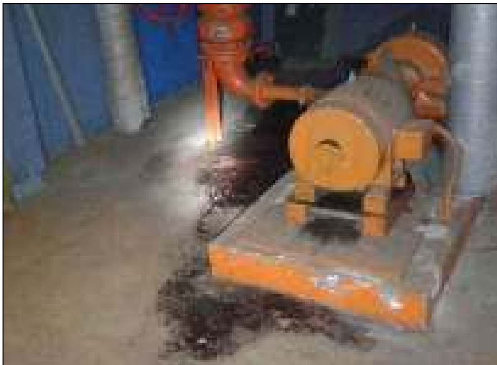
Photo 4: View of staining in vicinity of drain/sump in upper basement level and electric fire pump equipment
