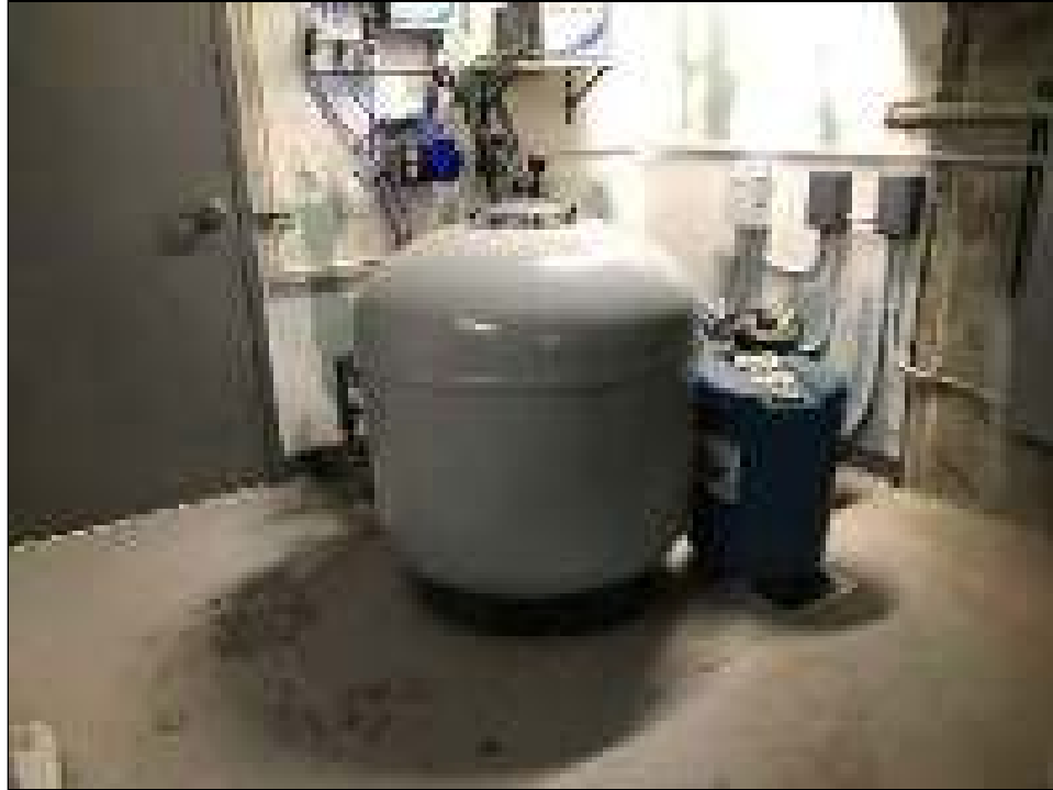
Photo 28: View of the pool equipment (basement level).
