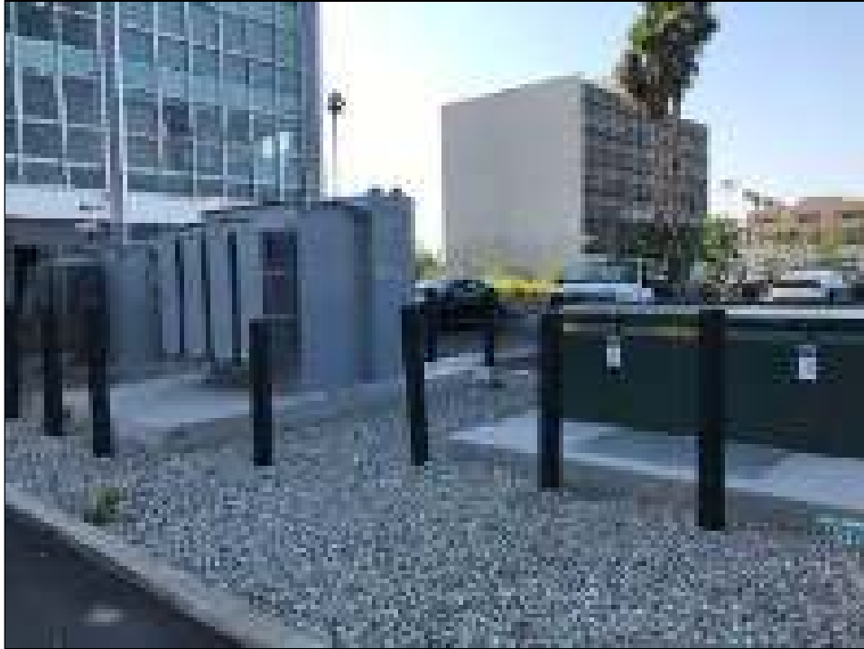
Photo 14: View of three transformers located in the residential parking lot.
