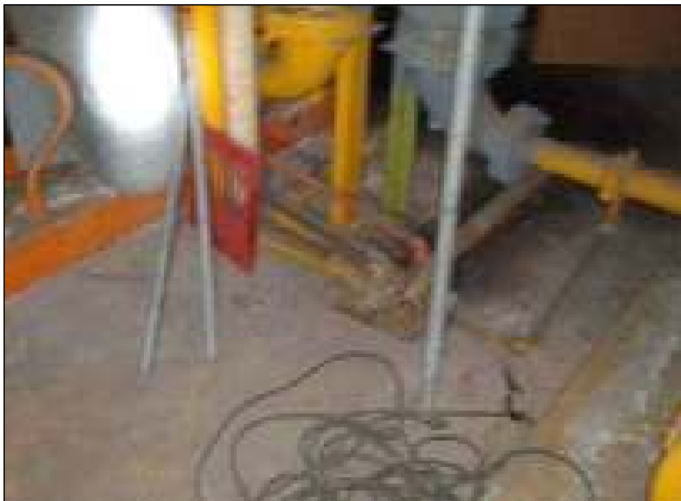
Photo 2: View of drain/sump in upper basement level and electric fire pump equipment
