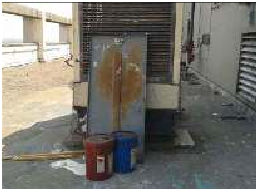
Photo 9: View of diesel-powered emergency generator
