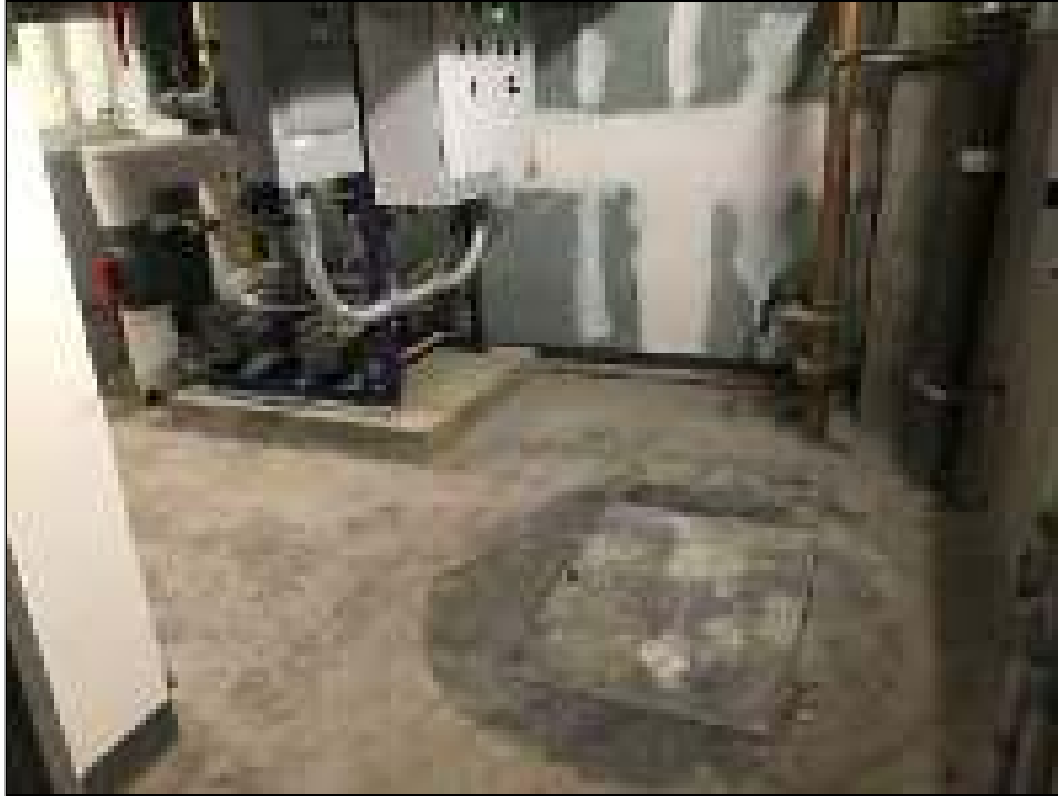
Photo 29: View of the sewer-connected sump-pump (basement level).
