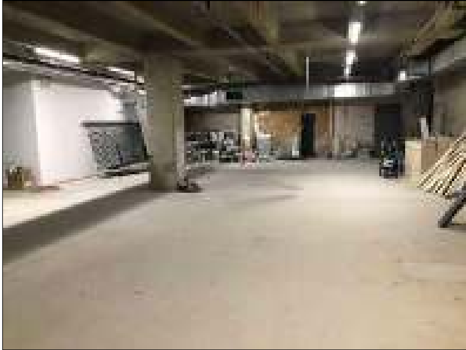
Photo 25: View of the storage and maintenance room (basement level).
