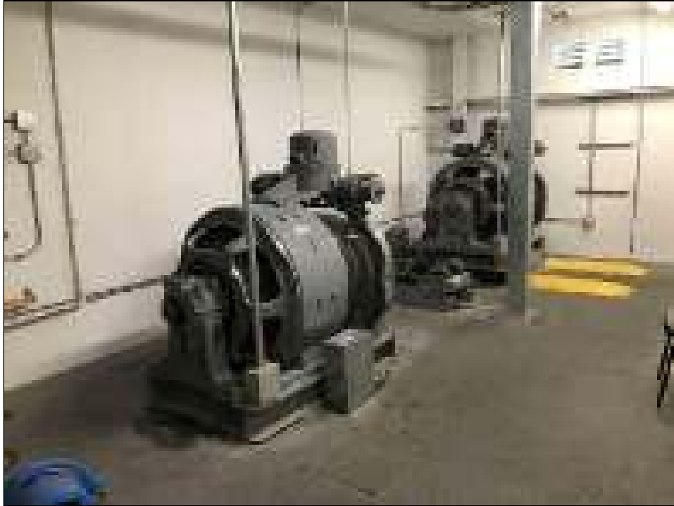
Photo 32: View of the traction elevator equipment.
