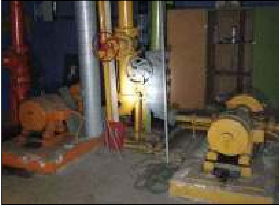
Photo 5: View of drain/sump in upper basement level and electric fire pump equipment
