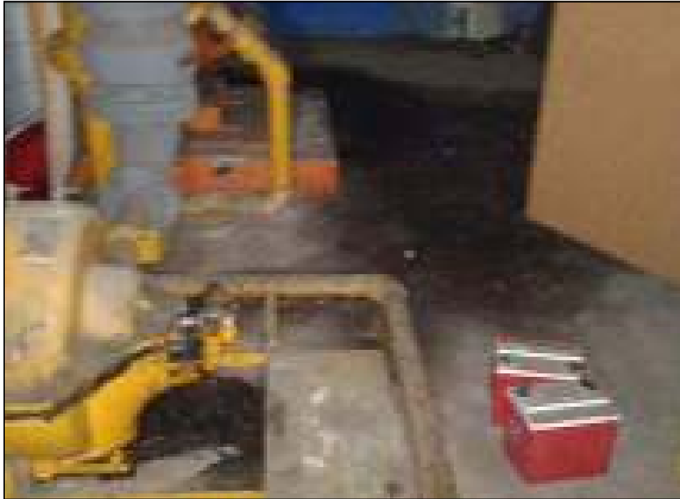
Photo 3: View of staining in vicinity of drain/sump in upper basement level and electric fire pump equipment
