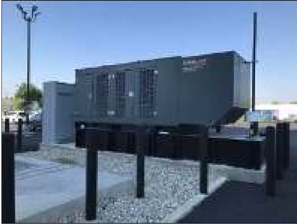
Photo 15: View of the Panorama Tower's emergency generator and attached belly-tank (AST).
