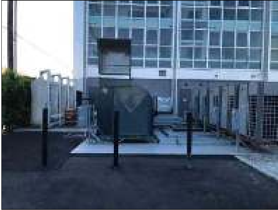
Photo 13: View of the electrical and HVAC equipment located in the residential parking lot.
