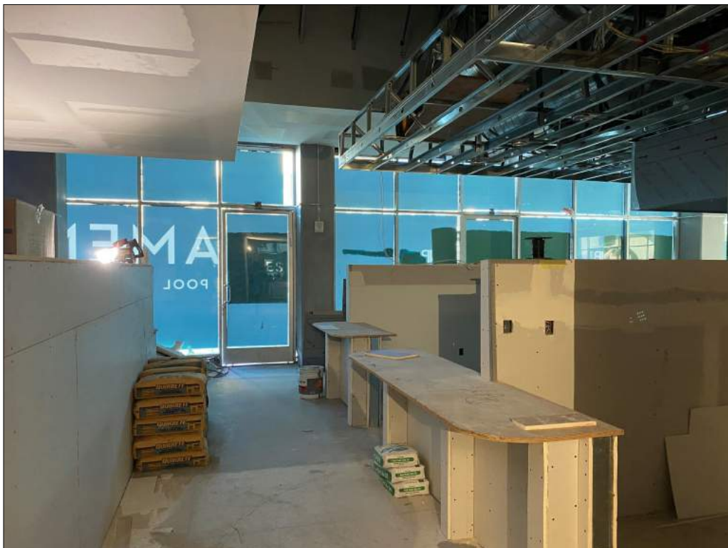
Figure 8: Panorama Towers, 8155 Van Nuys Blvd., interior of retail space at east elevation under construction, view east (Snow, 2022)
