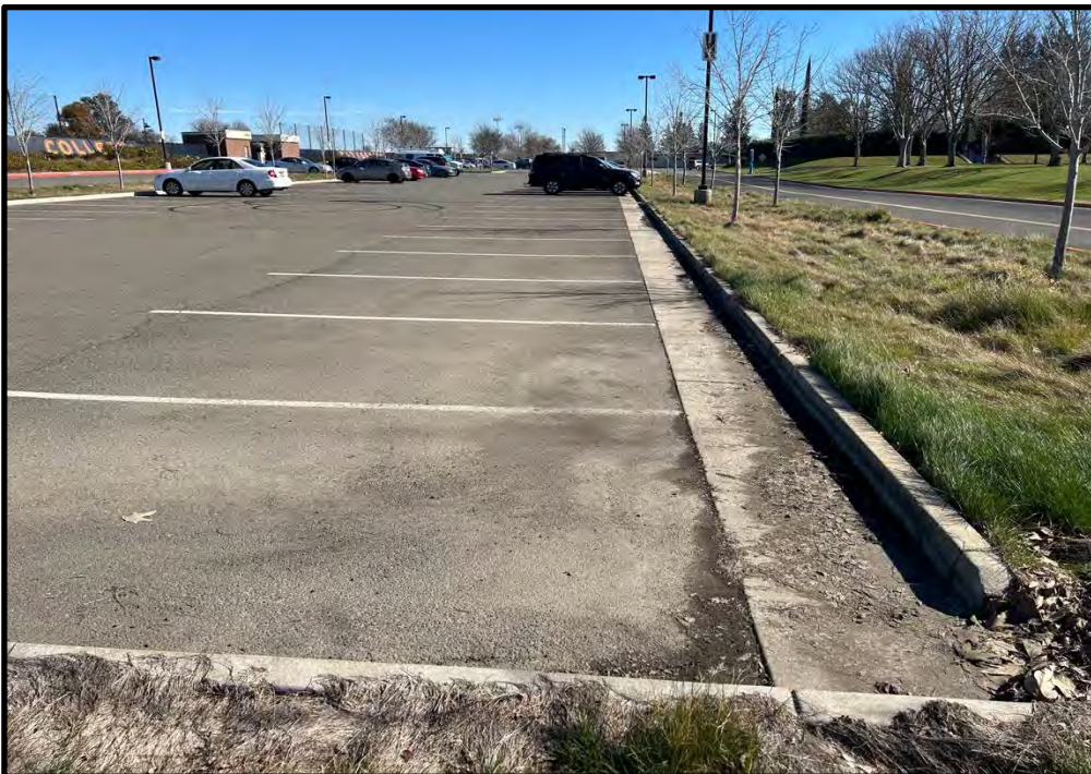
South edge of the north parking lot, looking east from the southwest corner of the north parking lot; 02/06/23.
