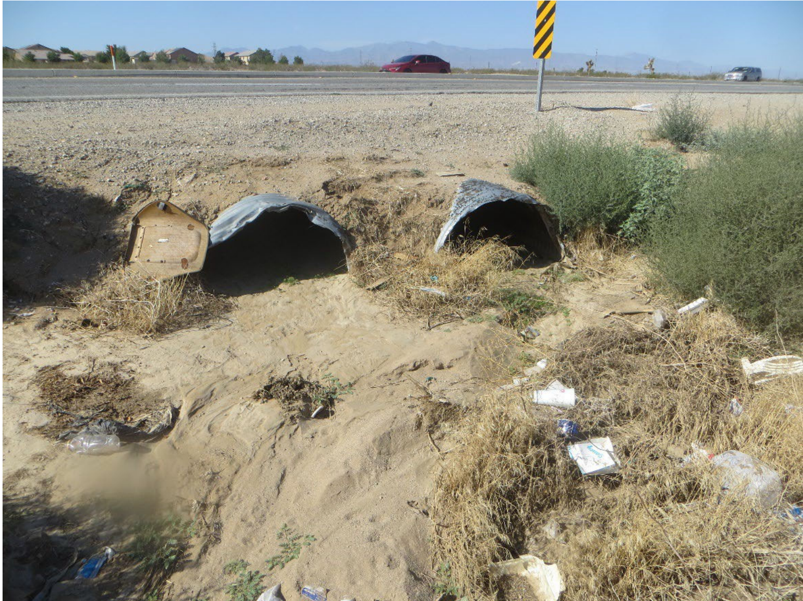
Culverts located at the southern project boundary. Drainage flow conveys toward the northeast.
