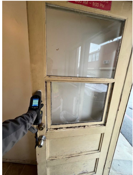
Picture 2: XRF detected lead-based paint on the laundry room door of 6016 Norwalk Blvd. Whittier
