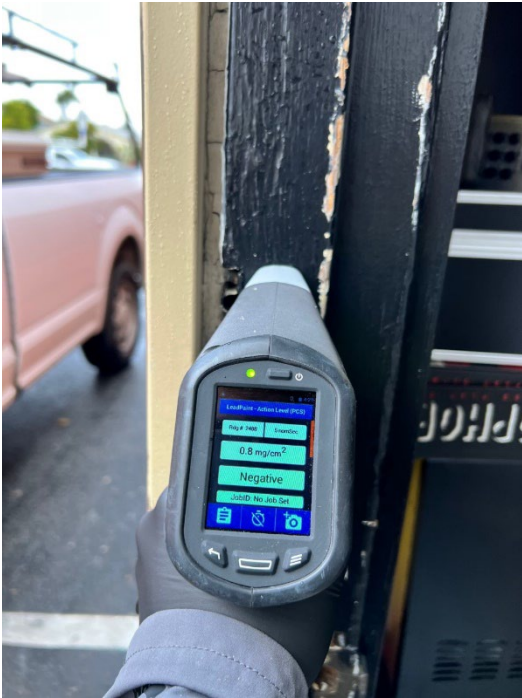
Picture 1: XRF detected lead-based paint on the door jam of 6014 Norwalk Blvd. Whittier
