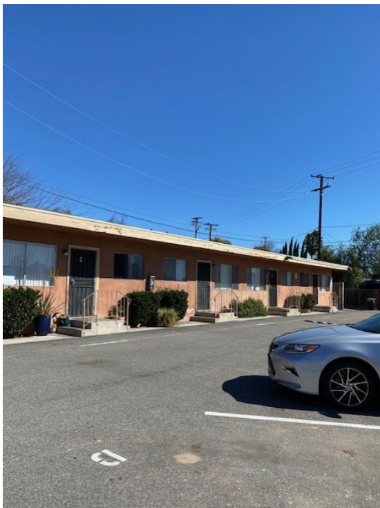
Picture 5: Scope of the stucco sampled from the property
