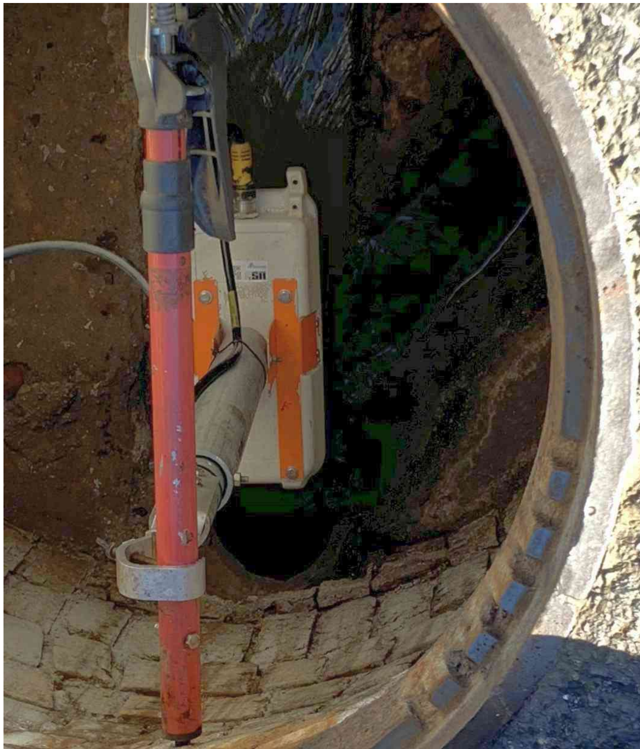
Figure 10 above: City MH 20 provided access to a 10-in sewer line, which entered from the northeast and discharged to the southwest, with a lateral entering from the east. Gas levels were within OSHA permissible exposure limits. The flow monitoring equipment was set to monitor the downstream west line on 2/19/2021 to get the total flow. US 3 followed up on this installation on 2/19/2021 to confirm equipment calibration
