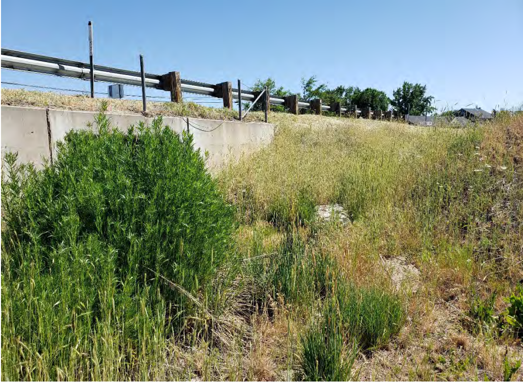
Image of an intermittent stream culverted beneath State Route 299 and connected on both sides by roadside ditches. View toward the northeast.
