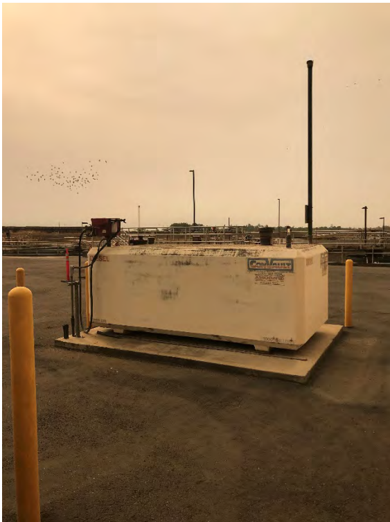
Photo 2: View of OPUD wastewater treatment facility diesel aboveground storage tank with secondary containment.
