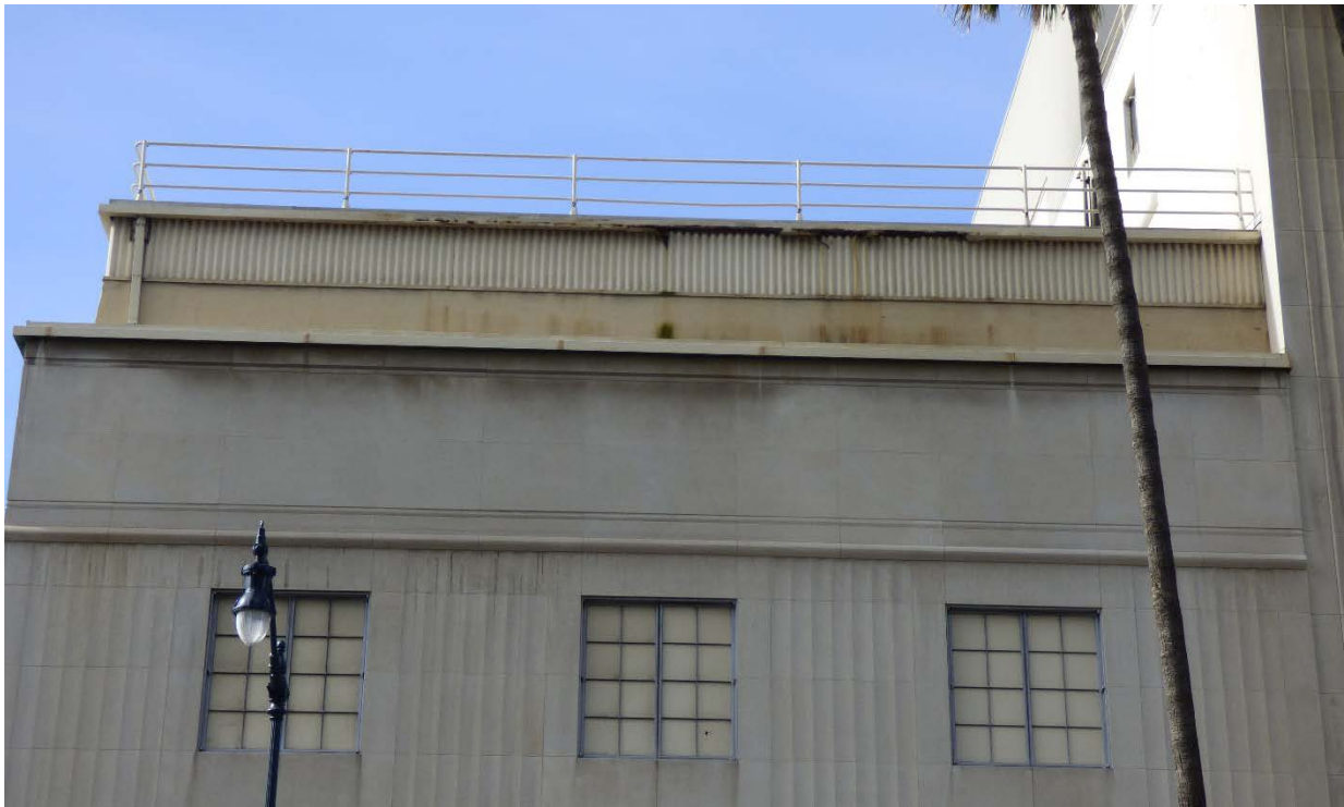
Image 5: Unit #1, existing rooftop addition at north (primary) façade, view south from Wilshire Boulevard
