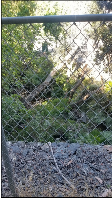
Photo 11. Looking west toward Tennis Club and at nonnative woodland and concrete debris in wash. June 10, 2020.
