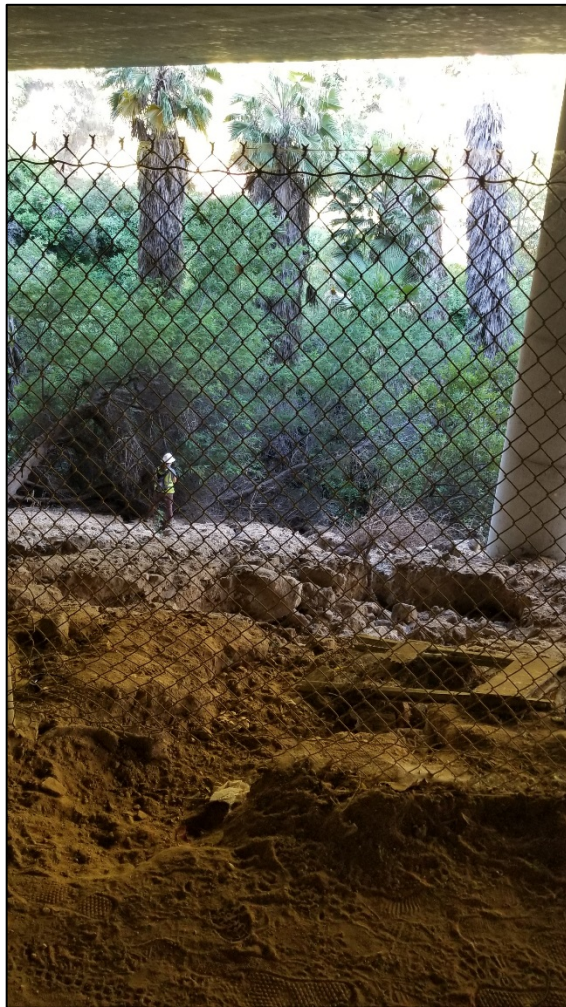
Photo 6. Looking at erosion downslope of trail under I-210 and disturbed willow riparian habitat west of I-210. June 10, 2020.
