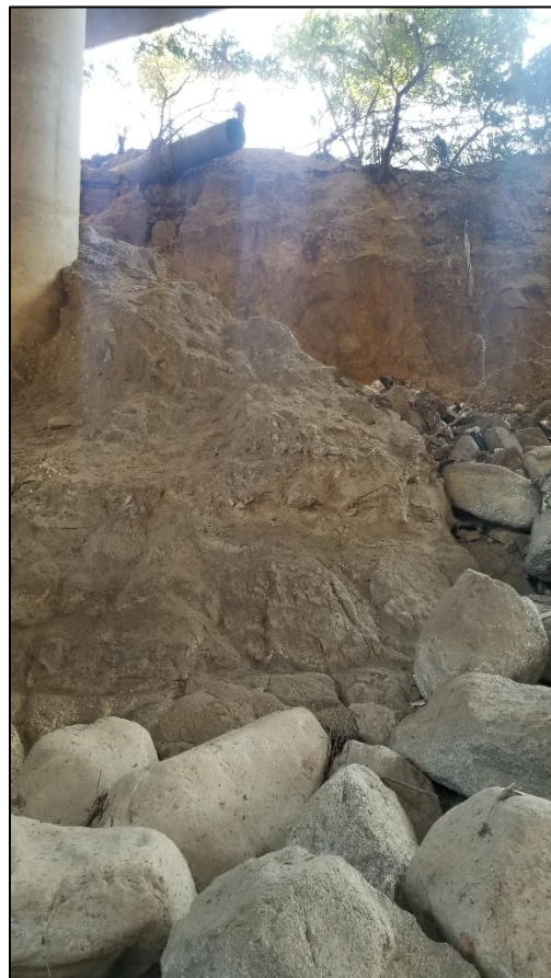
Photo 4. Looking north toward trail at erosion under I-210. July 17, 2020.
