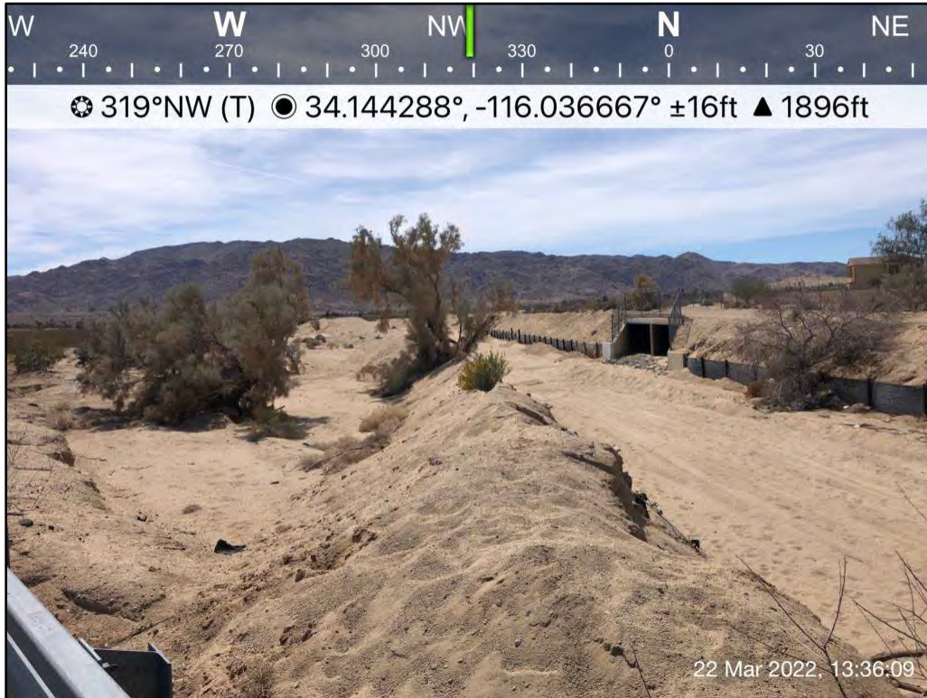
Photo 5. View upstream of flood control channel (Desert Wash System) from Utah Trail.
