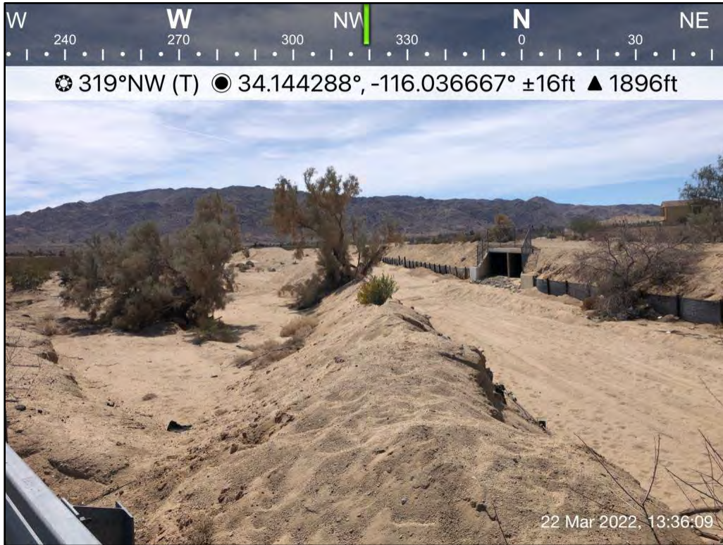
Photo 5. View upstream of flood control channel (Desert Wash System) from Utah Trail.
