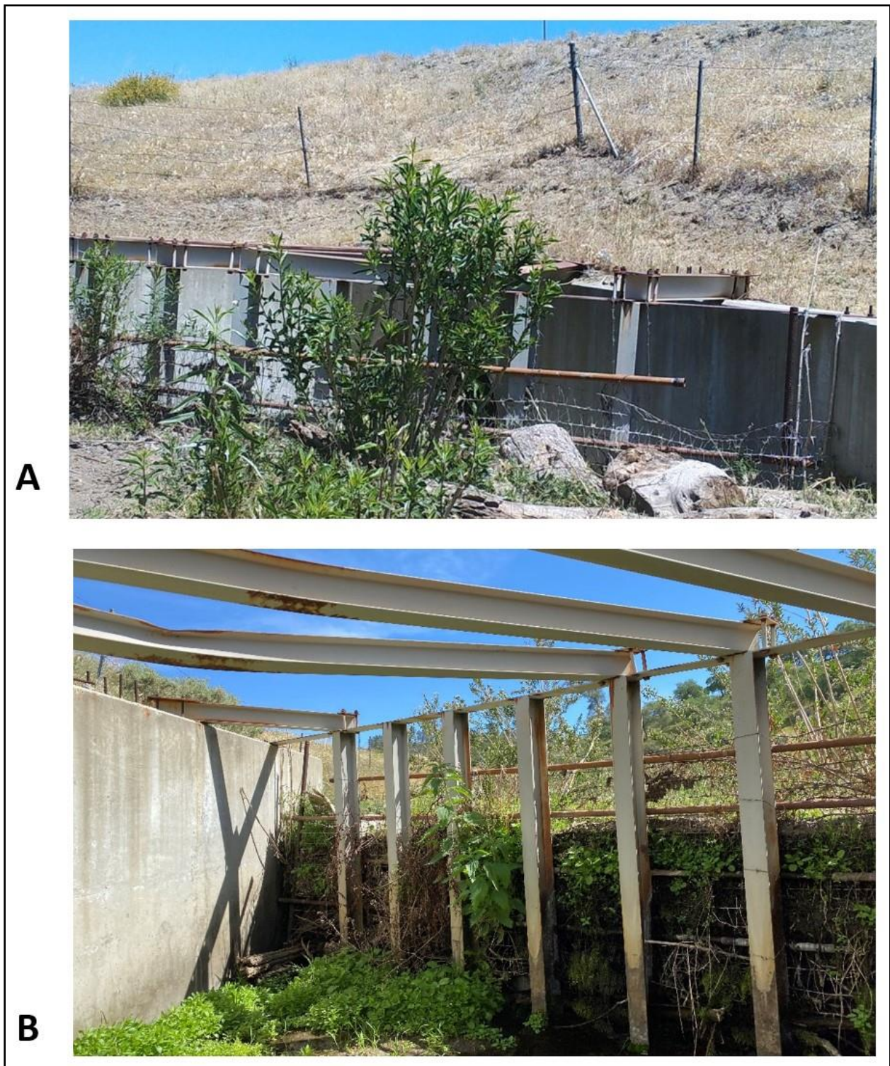
Figure 14 - Debris deflector structure located on a 5-foot culvert inlet within the project area. Images show a view from outside (A) and inside (B) the structure. Wildlife have difficulty using the culvert to pass under the roadway because of the structure.
