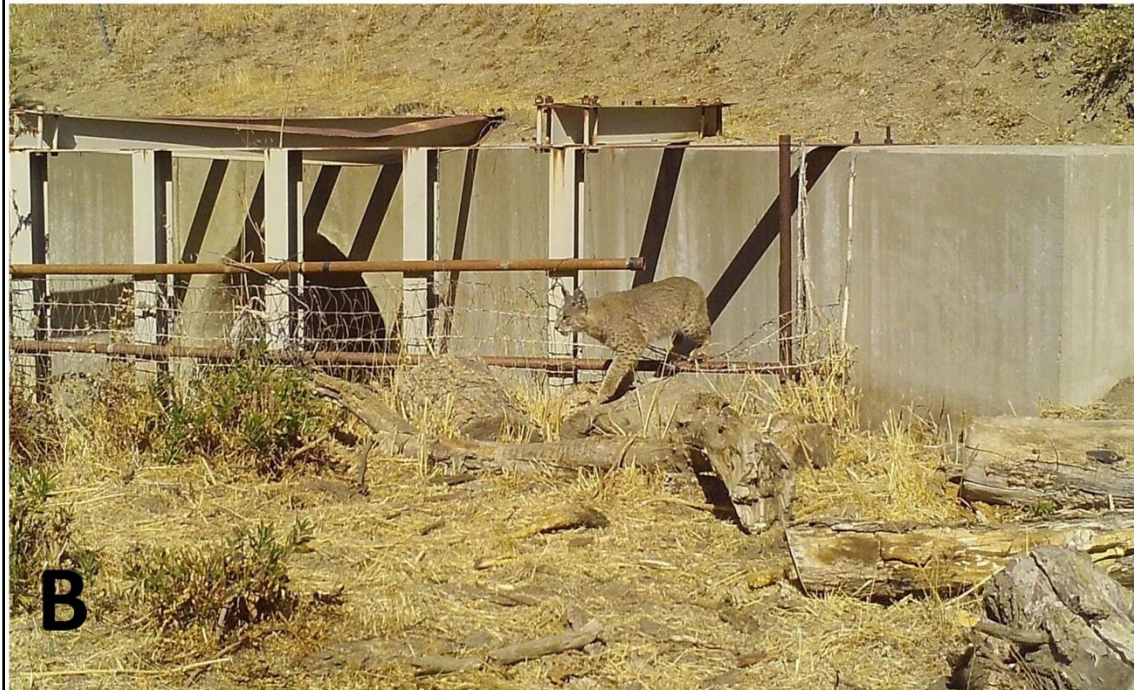
Figure 17 - Photos of bobcats using the culvert outlet (A) and inlet (B) at post mile 78.7. Photo B shows a bobcat exiting the debris structure from the damaged location where some wildlife enter and exit the culvert.
