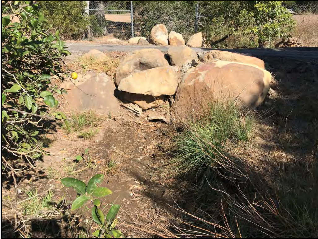
Photo 9: Clogged culvert along the main access driveway, near the middle of proposed Lot 1 (Aspect: North). Photo taken 10/31/2019.
