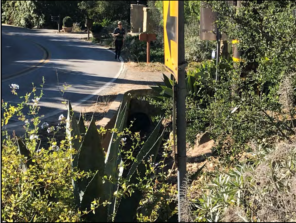
Photo 5: Downstream culvert along San Ysidro road that receives flow from the ephemeral drainage and channels it back to Oak Creek (Aspect: Southwest). Photo taken 10/31/2019.
