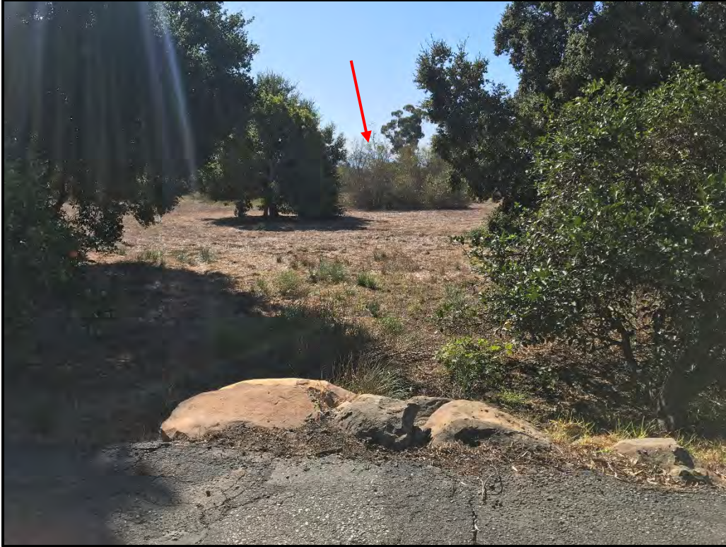
Photo 11: View from clogged culvert along the main access driveway, toward willows in the center of proposed Lot 1 (red arrow) (Aspect: South). Photo taken 10/31/2019.
