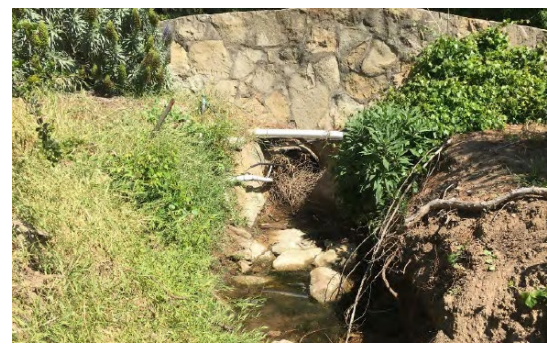
Photograph 4. An existing 24-inch culvert spans an unnamed ephemeral drainage bisecting the Project site.
