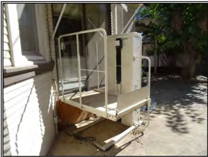
Looking at the wheelchair lift located adjacent to the southwestern wall of Structure B.
