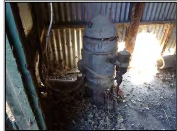
Looking at the irrigation well in the pump house.
