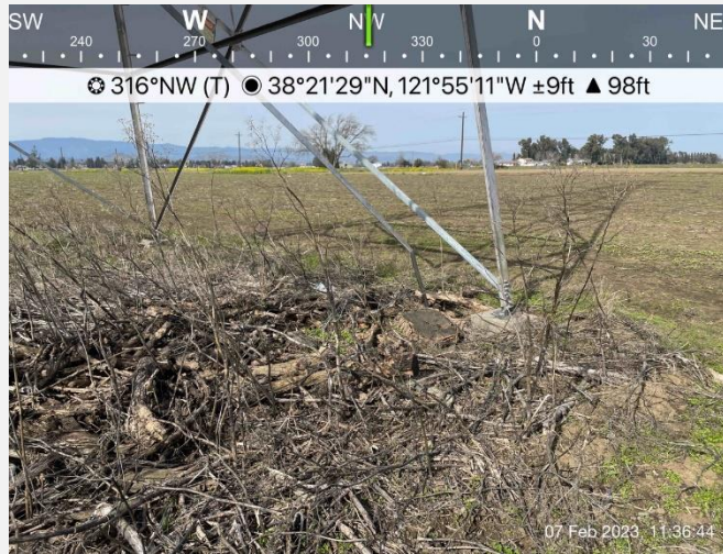
Photo 7. View of woody thatch below electrical tower near northeast corner of site.
