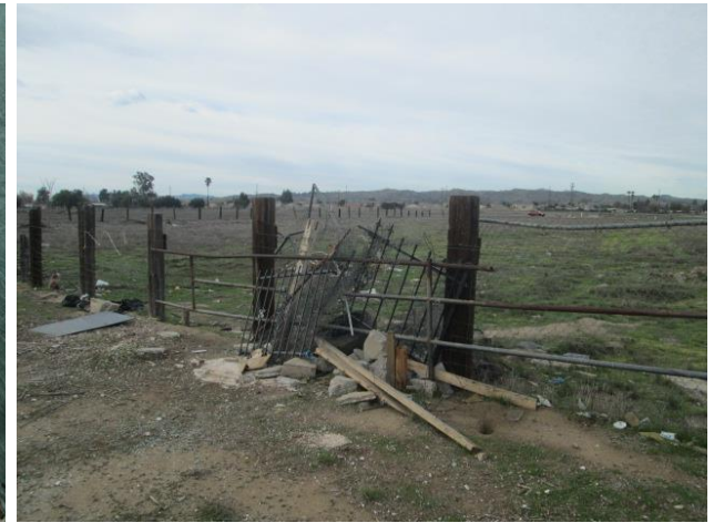
33. Typical debris/trash at 3060 Wilson Avenue.
